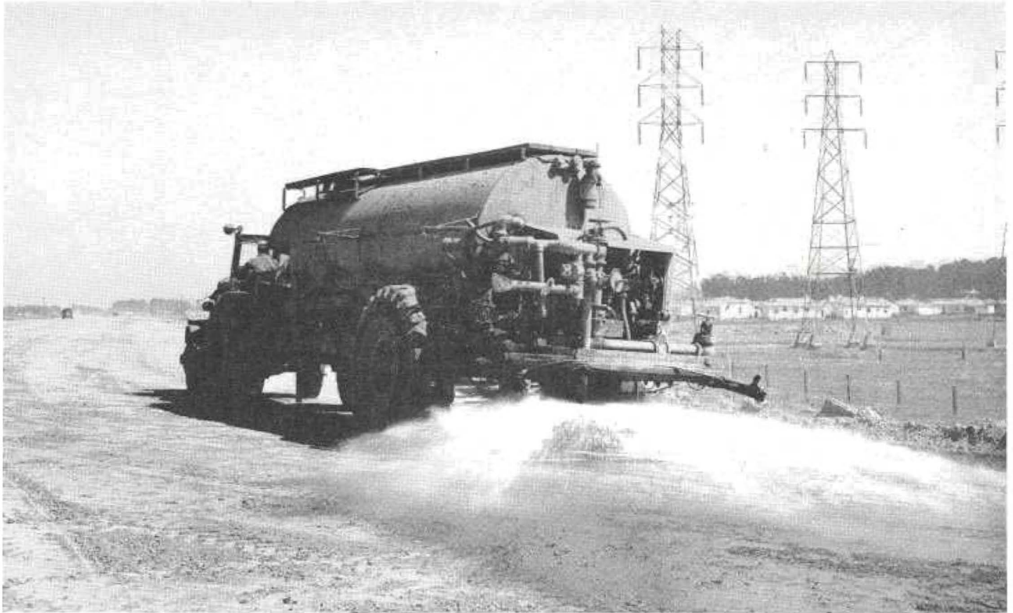
Fan sprays on 4,500-gallon water truck mounted on Euclid truck unit in operation
