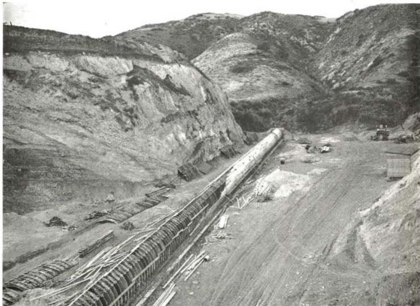
Concrete drainage culvert under construction in Puerto Canyon as a unit of the relocation of the Roosevelt Highway in Los Angeles County
