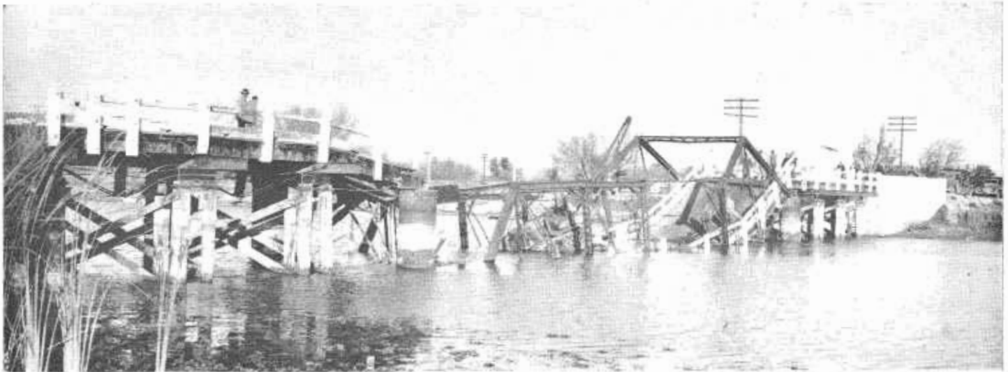
This is how the White's Bridge looked after it was wrecked. The 119-foot truss was completely destroyed
