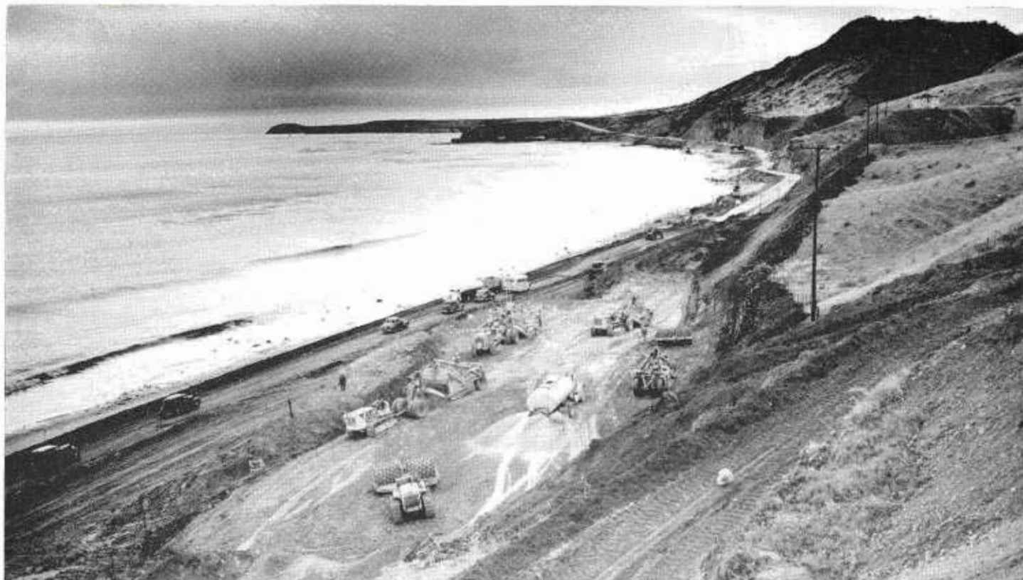
This view is looking north toward the end of the project involving the relocation of Roosevelt Highway north of Santa Monica
