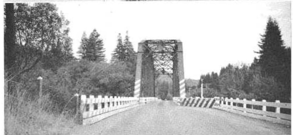
Upper—Existing bridge across South Fork of Feather River at Bidwell Bar, Butte County. Has been in use since 1856. The wire cables and wrought iron hanger rods were brought by ship around Cape Horn. When replaced it will remain as a foot bridge in the Bidwell Bar State Park. Center—This bridge is typical of many structures which are no longer able to meet the demands of highway traffic and must be replaced as soon as possible. Lower—Russian River Bridge at Hacienda, Sonoma County. A one-way bridge, originally designed for a single track railroad, which for many years has been used as a highway bridge. Reconstruction will provide for spreading the trusses and building new concrete approaches so as to make clearances for two lanes of traffic
