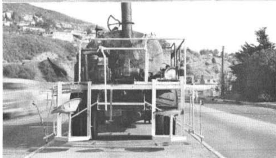
Upper—Using full circulating metal covered hose and nozzle arrangement on 940-gallon tank assemblies for longitudinal joint sealing. Center—Two types of assembly used for joint sealing. Old type in operation on left, new type on right. Lower—Latest improvement of full circulating type assemblies with swivel joints for longitudinal joint sealing
