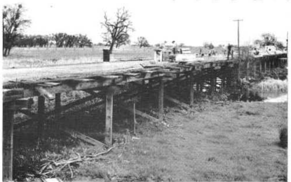
Bear Slough Bridge, Sacramento County. This picture shows a portion of the existing structure with construction forms under way for new bridge
