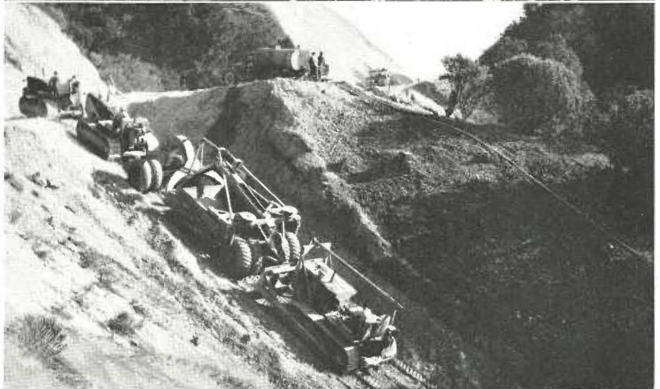
Upper—New construction virtually took a straight swath through the original crooked alignment. Lower—Starting the deep fills required cooperative tugging and pushing on part of heavy equipment
