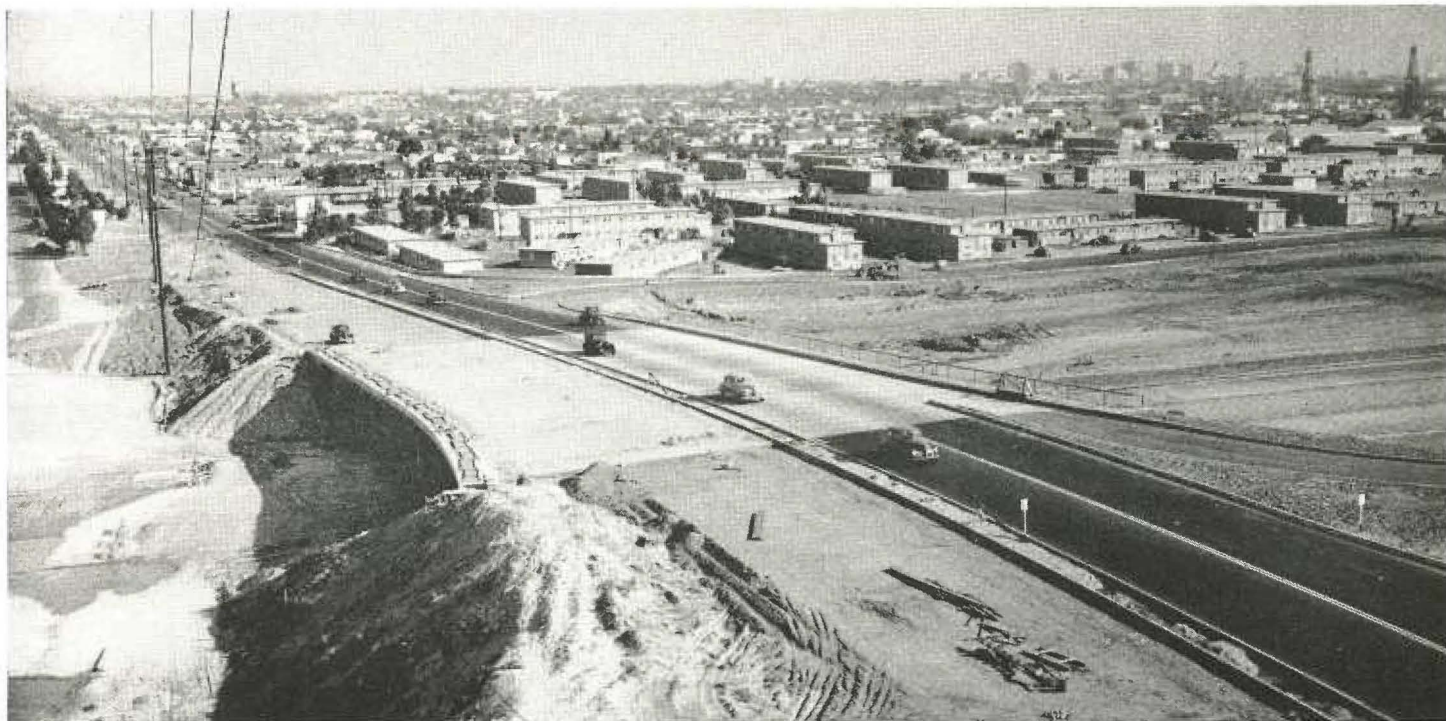
Terminal Island Freeway undercrossing looking east along State Street (Pacific Coast Highway)
