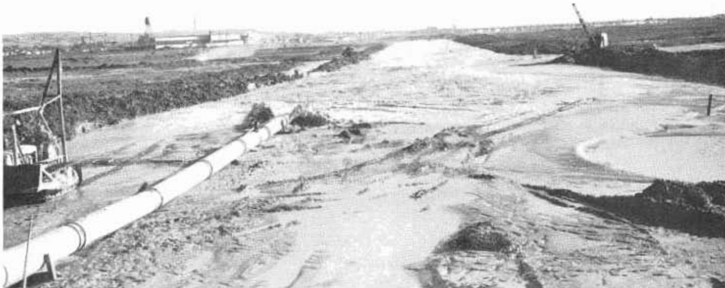
Elmhurst Creek, looking south and showing outfit of dredger pipe. Tractor on left used for moving and placing pipe and reinforcing levee.
