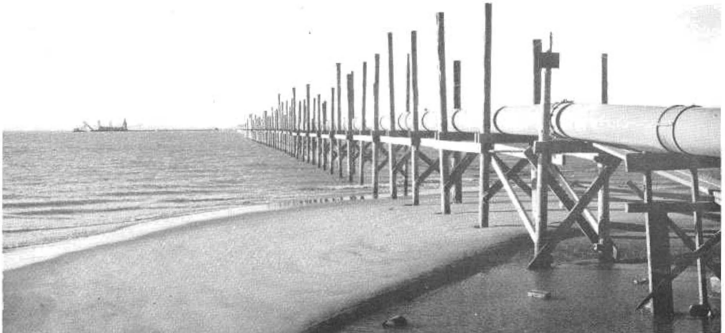
Levee on Bay Farm Island, looking west and showing trestle for dredger pipe. Suction dredge and floating line in background.
