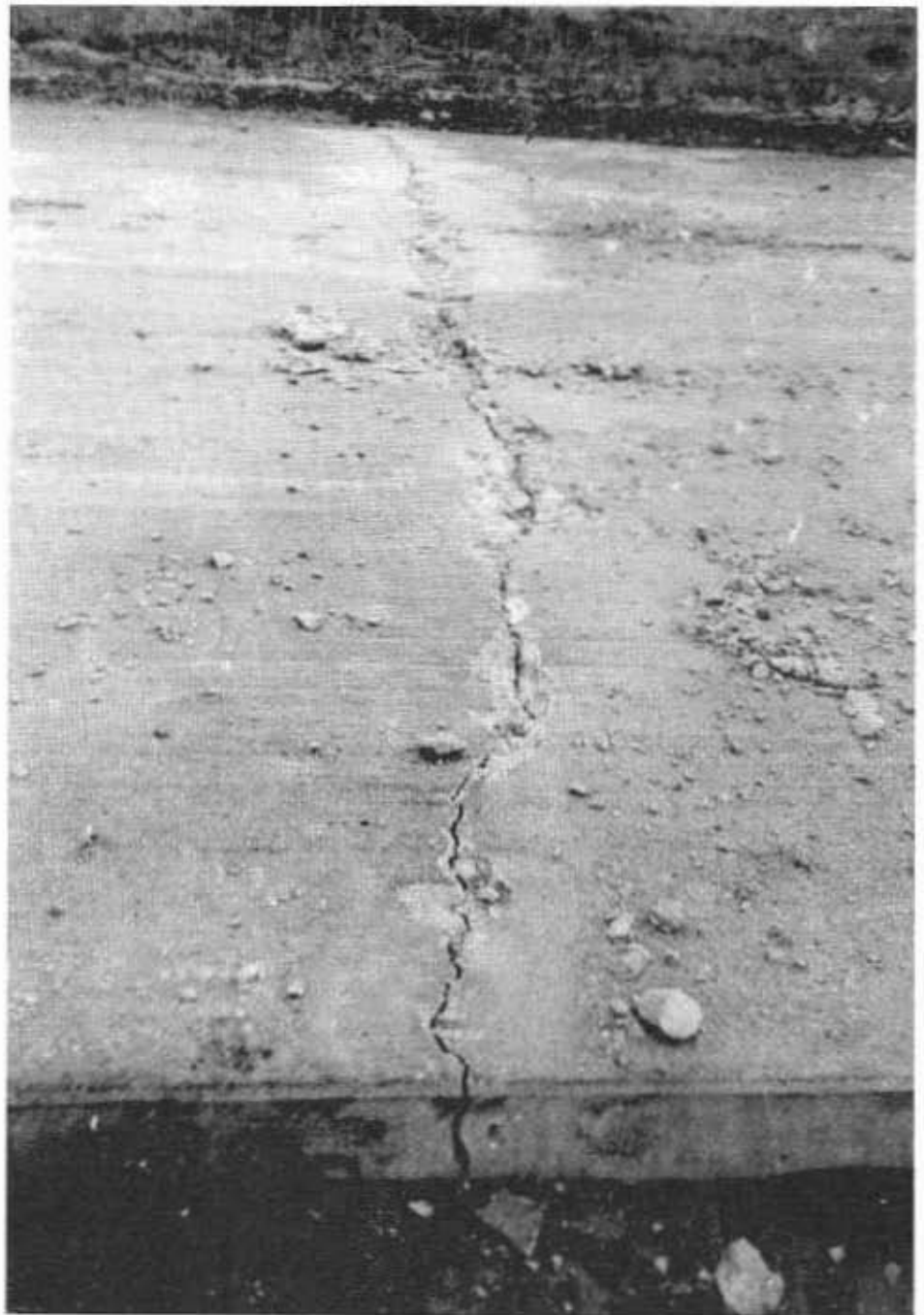
This photograph shows one of several similar cracks that developed between 80 and 300 feet from an unrestrained end of a long unreinforced concrete pavement. No expansion joints were provided
