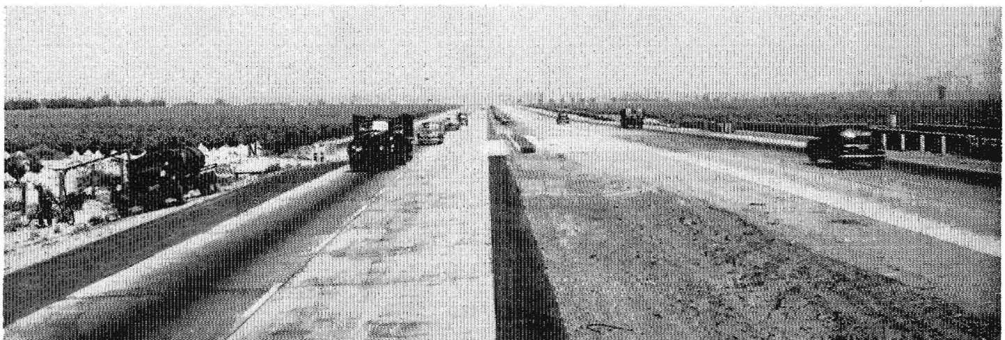
West of Etiwanda Avenue, showing heavy mixed truck and passenger traffic on new freeway. Pavement on right is former three-lane pavement now used for east bound traffic
