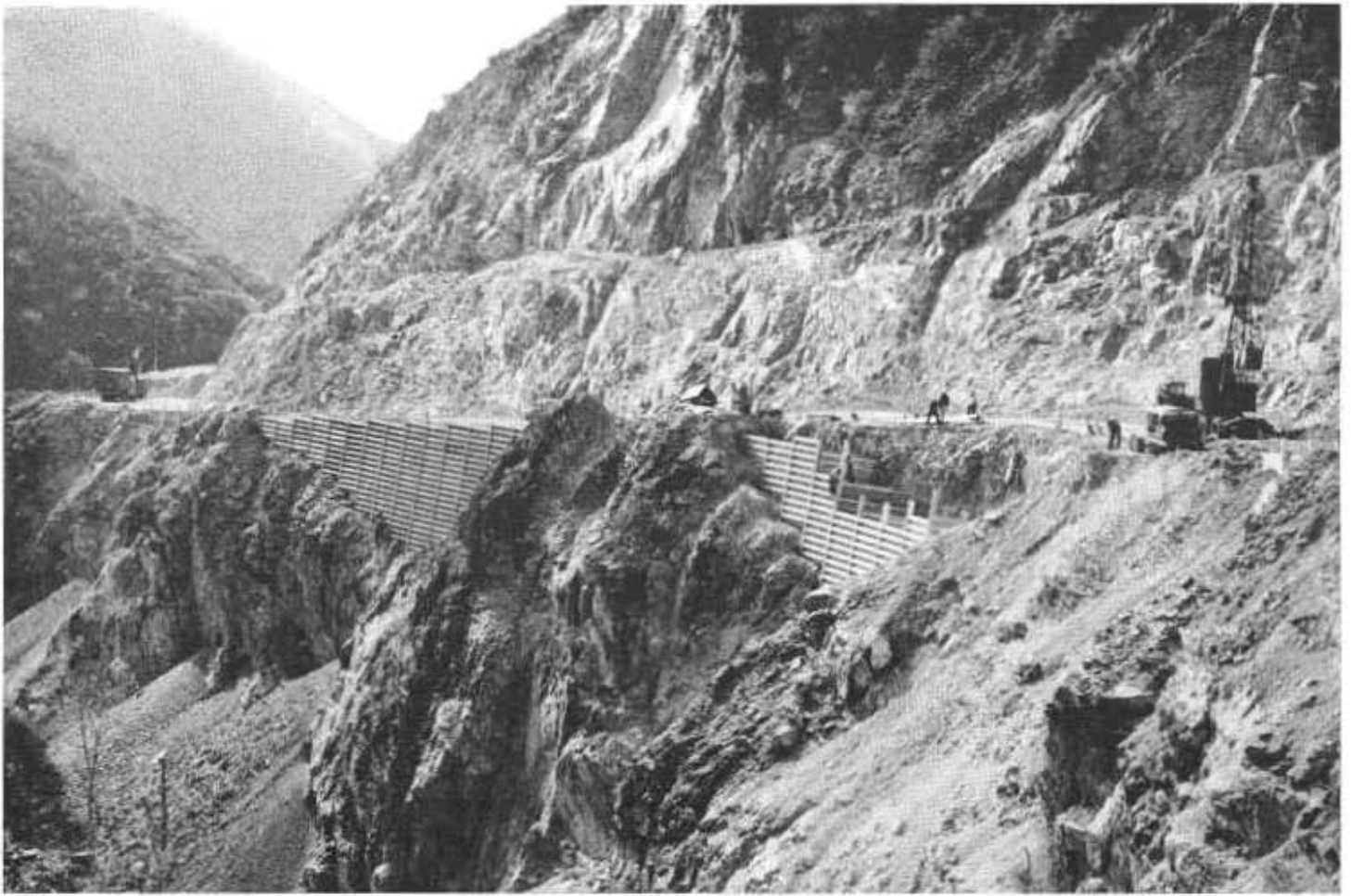
On a precipitous rock slope above the bed of City Creek on the First Unit are these two bin-type retaining walls. The one on left is completed, the one on right under construction. Remains of old road appear above
