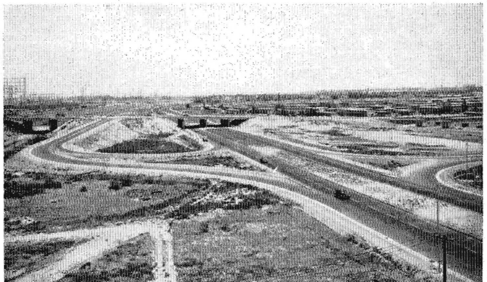
Looking north toward Pacific Coast Highway (US 101 Alt) grade separation over freeway, with Cloverdale connections in foreground
