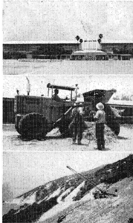
Upper—Race track. Center—Loading straw at stables. Lower—Rolling first application of straw with truck crane and tamping roller
