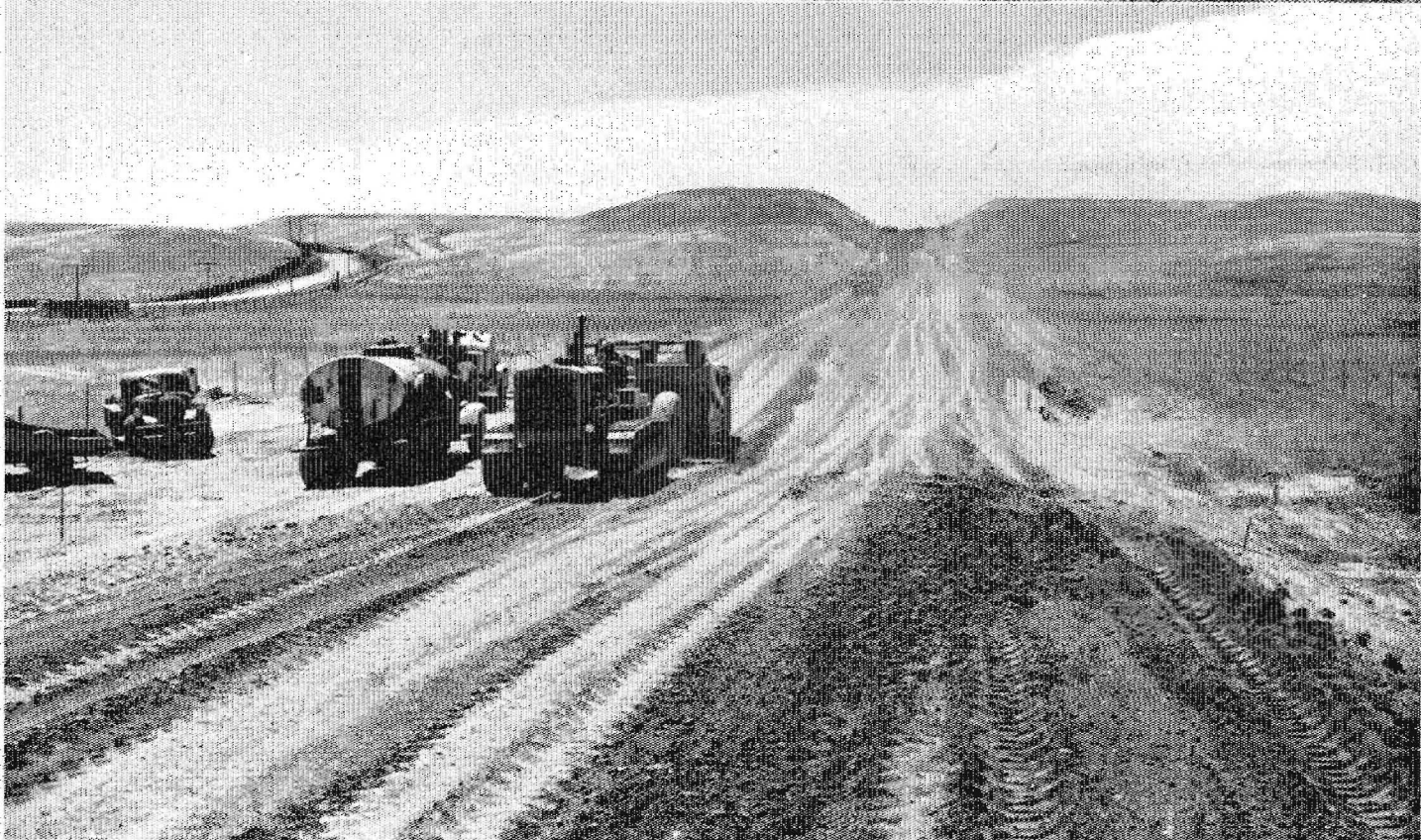
These two photographs show heavy equipment used in grading for the new Sacramento-Jackson Highway. Present winding road is shown at left of lower picture
