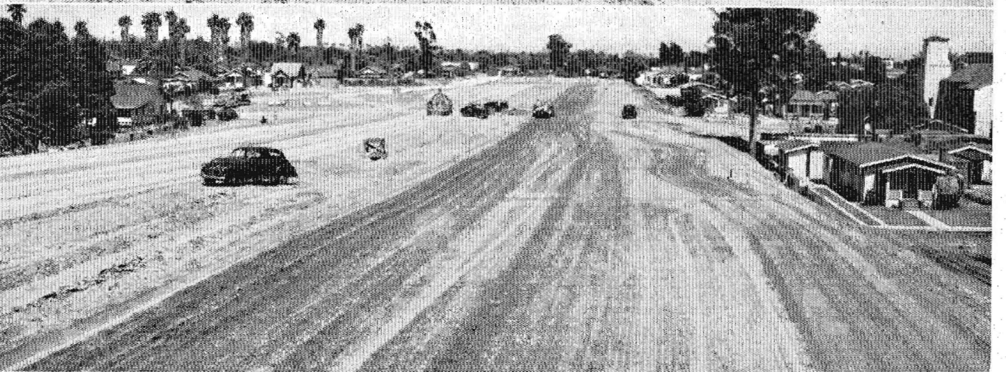
Upper—View looking west of Indiana Street grade separation, showing earth-moving and compacting equipment at work. Center—View looking east from Euclid Avenue grade separation, showing construction work in progress. Completed Lorena Street grade separation in background. Lower—Looking east from Indiana Street grade separation showing Eastman Avenue, the easterly terminus of the contract in the background. Grading is complete and roadway ready for subgrade and paving operations
