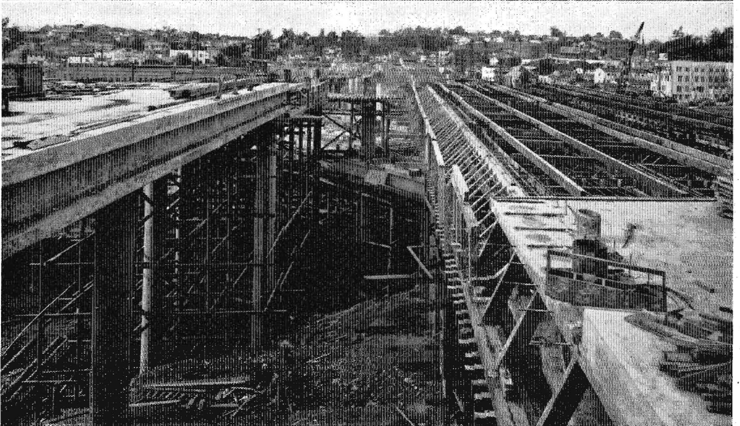
Upper—Figuroa Street undercrossing as viewed looking northwesterly with the Four-Level structure at left in the distance
