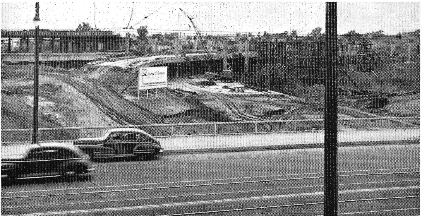
Four-Level structure looking south from the completed Sunset Boulevard Bridge over the Arroyo Seco Parkway
