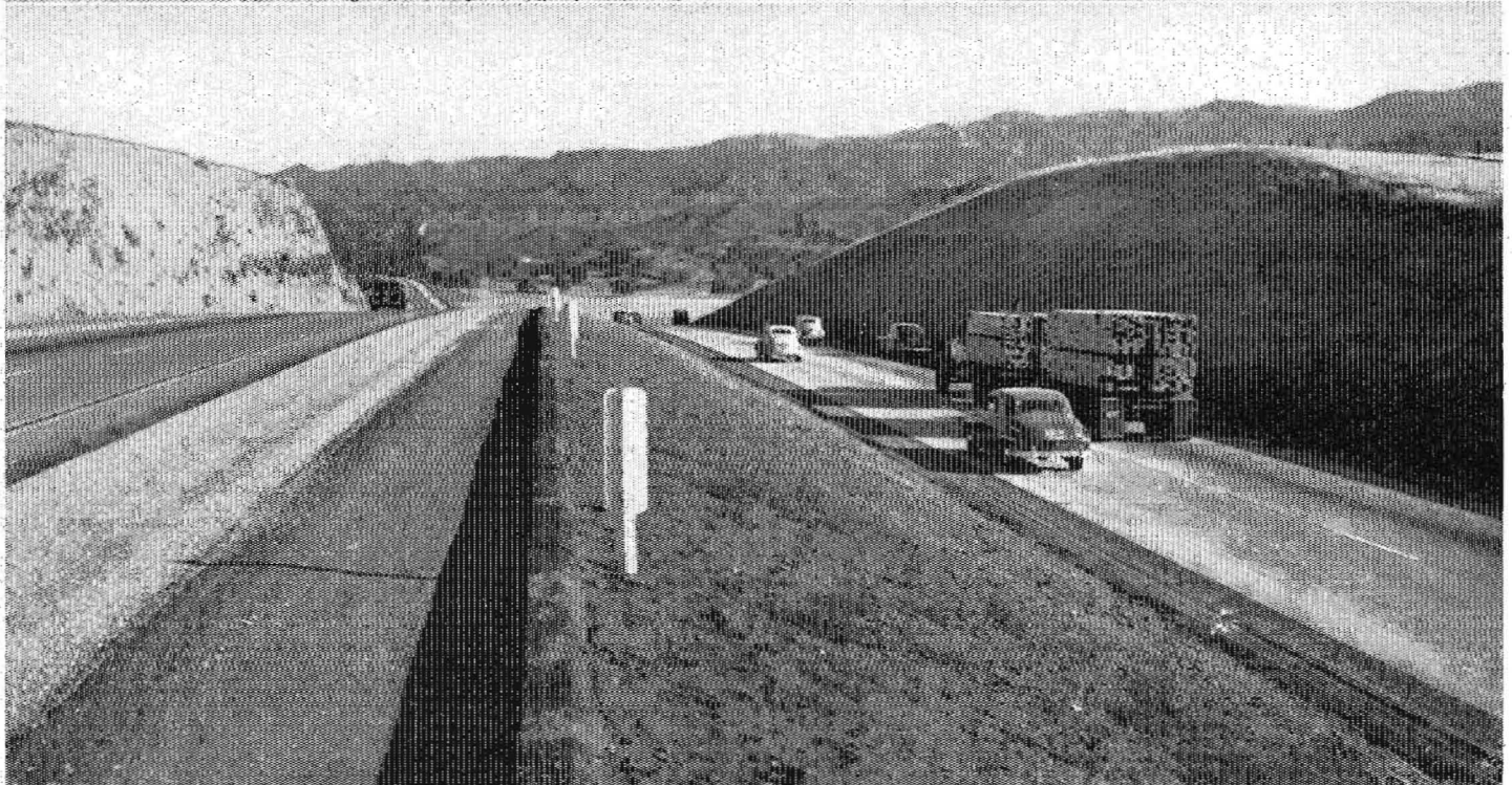
Upper—Completed section of Ridge Route north of Castaic. Lower—Completed section of Ridge Route between Santa Clara River and Pico Canyon, looking southerly, showing protection provided traffic where newly constructed pavement is lower in grade elevation than the existing pavement
