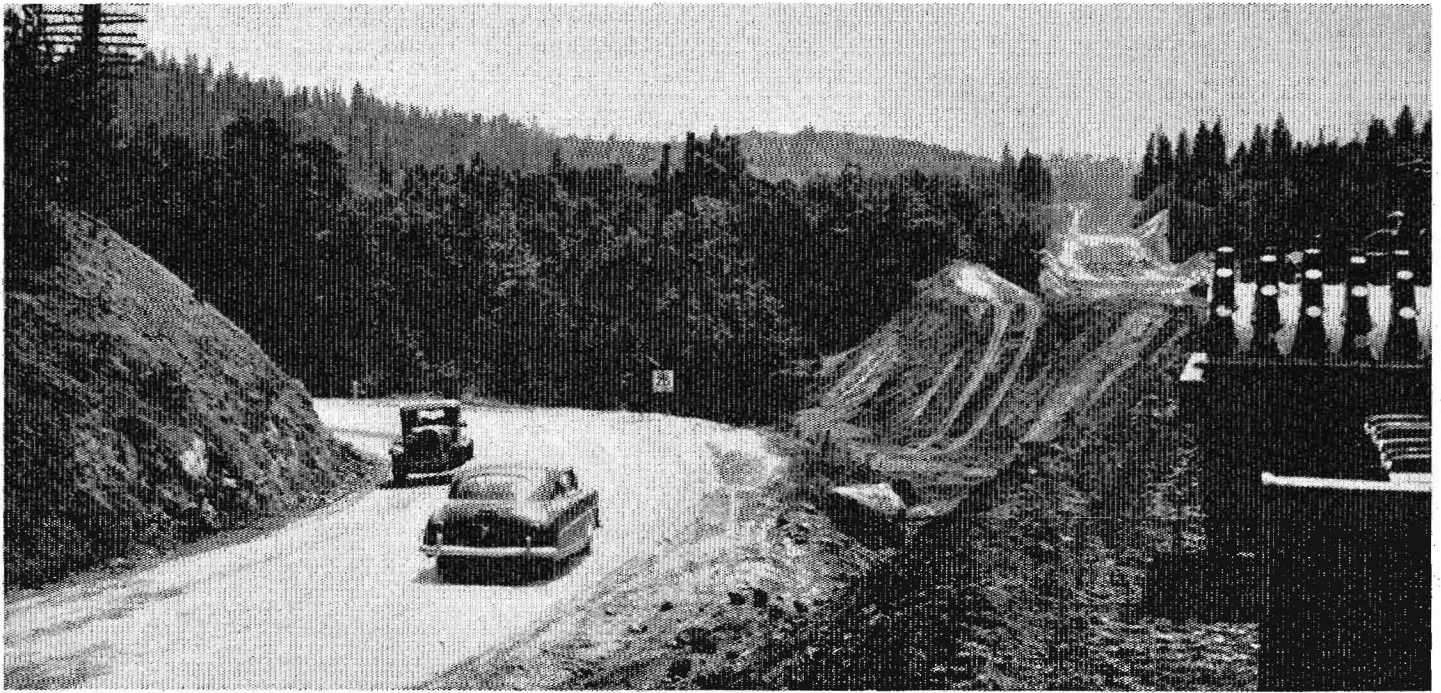
Beginning of construction of new four-lane divided highway on U. S. 40 between Applegate and Auburn in Placer County. Existing highway on left, grading for new location on right, looking west from Applegate
