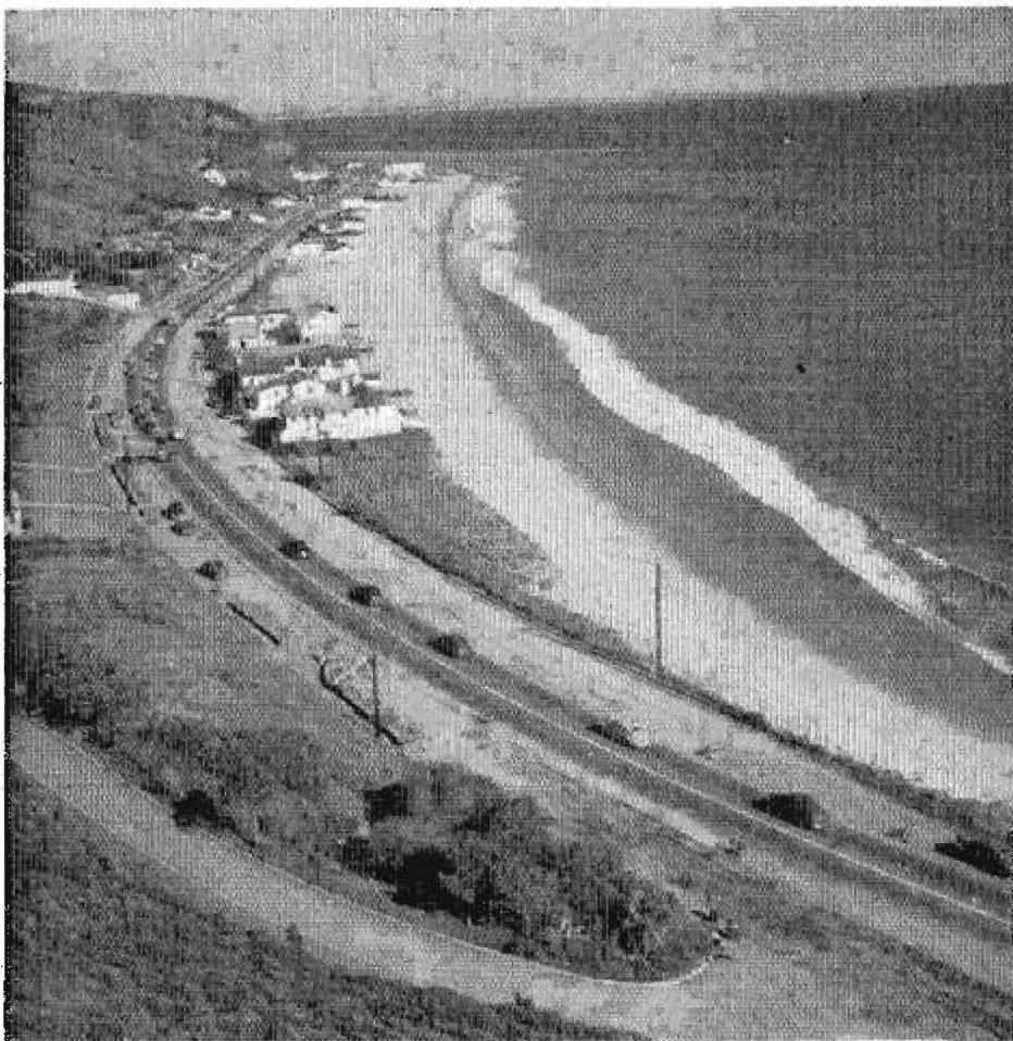
View from Carbon Point looking easterly and showing widening operations in progress
