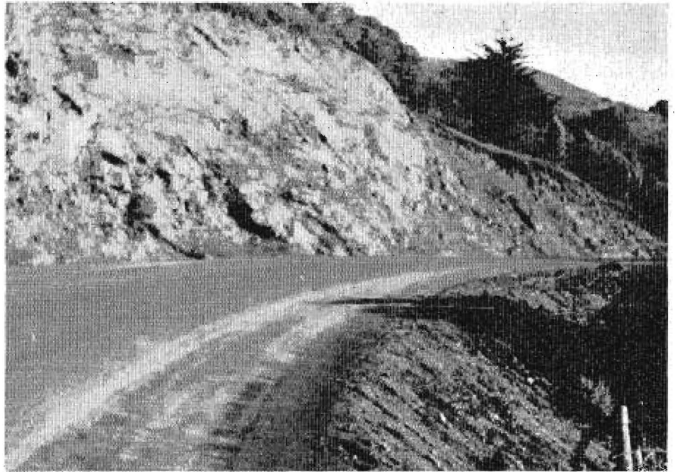
Looking westward at rock cut, where radius was increased from 85 feet to 250 feet
