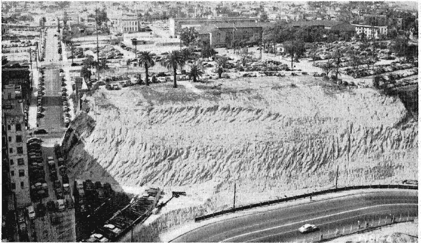
This portion of Moore Hill will be removed. Spring Street detour in foreground. California Street on left. Hollywood Freeway will go through to the right of California Street. South portal of Broadway Tunnel can be seen left center
