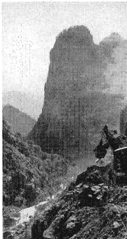
Pioneering Kings Canyon Highway in Fresno County with modern equipment, free operators, and inmate labor—1936
