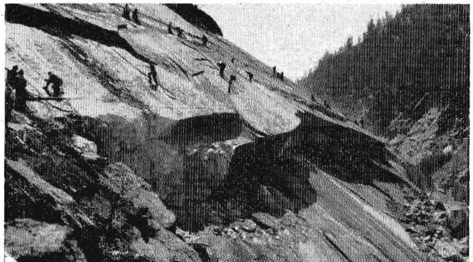
Typical hard rock excavation on Feather River Canyon Highway in Plumas County in 1936
