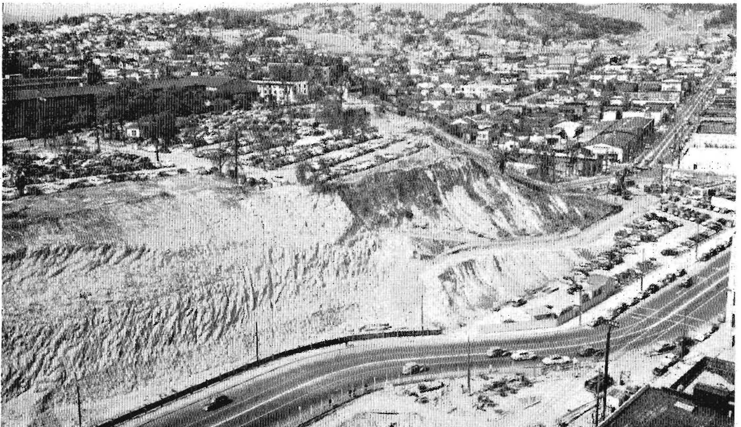
North end of Fort Moore Hill. Barricade erected by contractor along Spring Street detour to catch falling rock and dirt is shown in left foreground. Right center shows resident engineer's office, contractor's offices, construction yard and county parking ground
