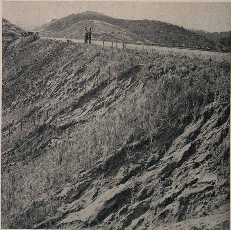
Damage on 1½:1 fill slope seeded to barley. No straw mulch was used. The soil is of a sandy and highly erosive nature
