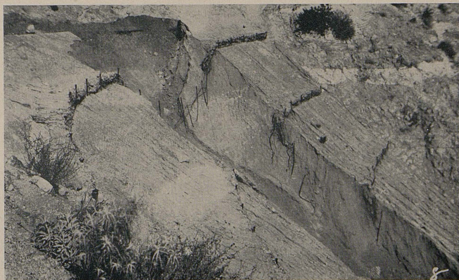
Iron pipe stakes and fencing fail to prevent slip out. Inadequate downdrains and resultant overlapping of the berm surface runoff contributed to failure. (Crest Drive, San Bernardino County)
