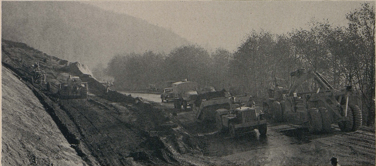
UPPER—Construction operations in progress just northerly of Stone Lagoon Summit. The new location through rugged country can be discerned in the distance descending to the sand spit, which can be seen at the extreme upper right edge of the photograph. LOWER—Grading operations at Stone Lagoon Summit at the south end of the project. The new location departs from the old highway at this point, the existing road being in the immediate foreground
