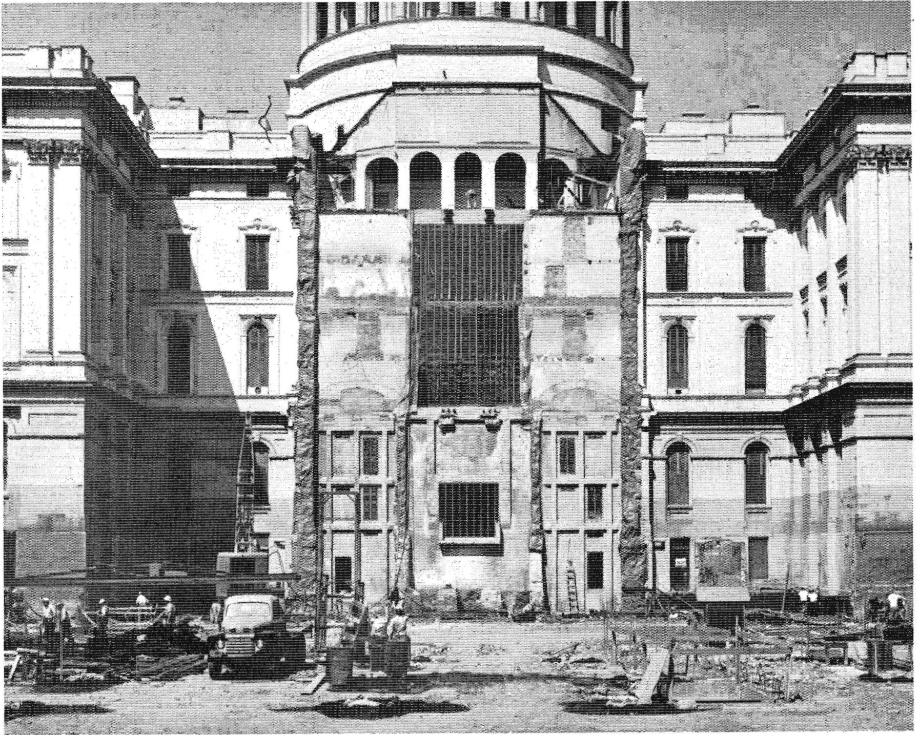
This is a view of reconstruction wall after removal of semicircular wing from the east side of the State Capitol Building
