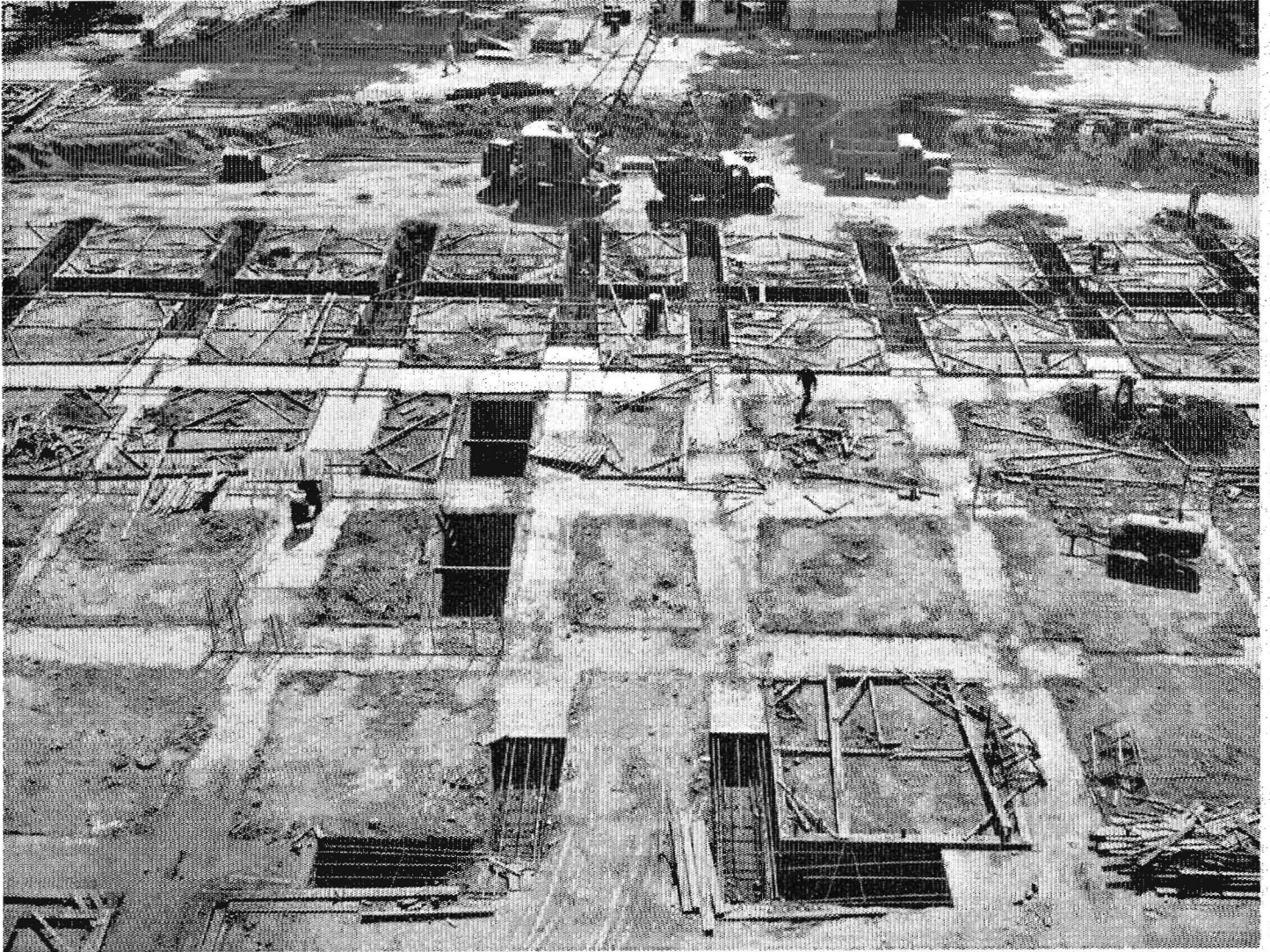
This is a partial view of the foundations for the new Capitol wing. Elevator pits are shown in center left
