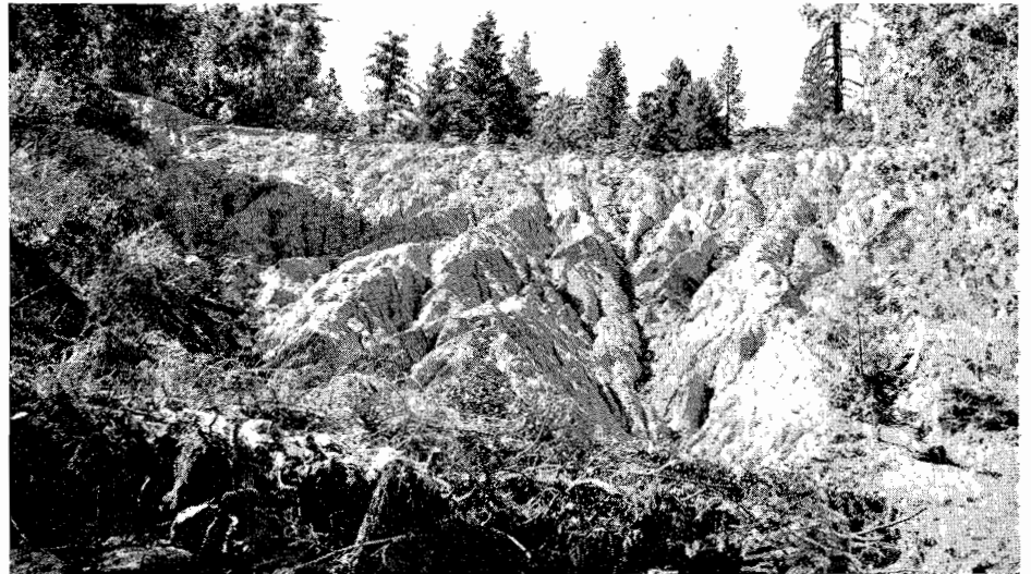
Hard, gullied disintegrated granite fill slope. Construction of log and brush crib at toe of slope is first step in repair procedure. (Near Weaverville, Trinity County)
