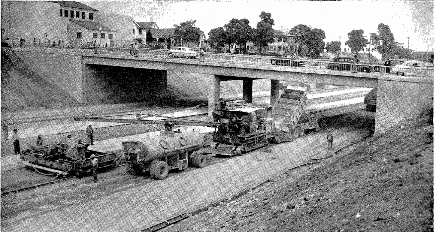
UPPER—Placing Portland cement concrete pavement on cement-treated subgrade. At Edgeware Road looking south toward Temple Street. LOWER—Portland cement concrete paving operations looking easterly at Edgeware Road Overcrossing
