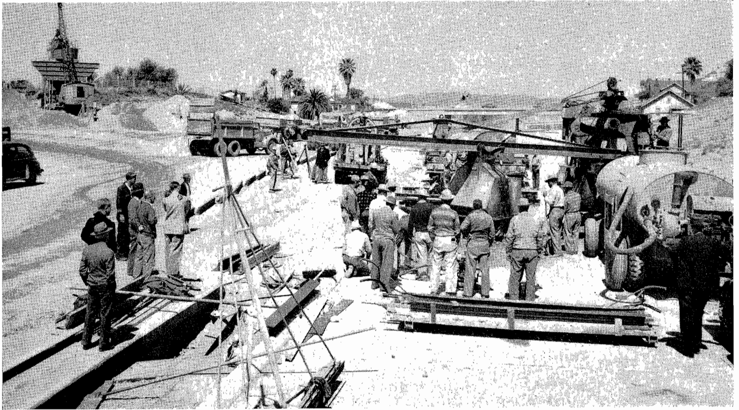
On May 4, 1950, the first concrete was poured for the pavement at westerly abutment of Glendale Boulevard grade separation
