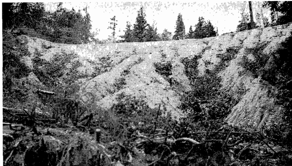
Brush is placed in gullies before backfill material is spread on slope face. Note log and brush crib at toe of fill. (Near Weaverville, Trinity County)
