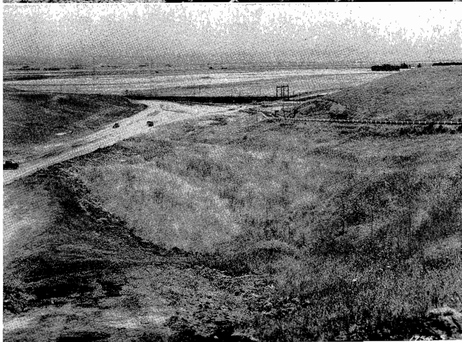
UPPER—Son-208-A. Shoulder widening on Sears Point Cut-off from excess excavation. LOWER—Son-8-A. Junction Black Point and Sears Point Cut-offs on relocated line looking north. Old road on right
