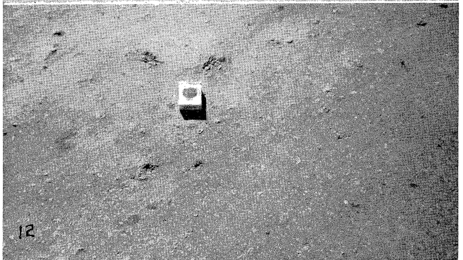
10—Failed section which was not treated with lime. This section was in satisfactory condition in October, 1948, but failed during the following winter. 11—Appearance in March, 1950. (Compare this with photo No. 7.) 12—Closeup of same section (compare with photo No. 8).
