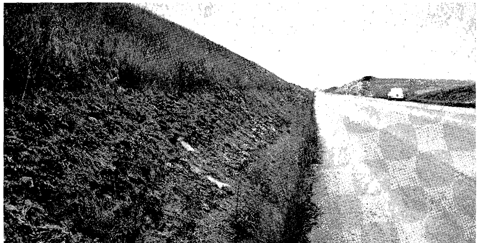
Fire-hazard-control strip formed by the "spray and burn" method. Note the quantity of unburned stems left on the slope after a quick burn. (Near Castroville)
