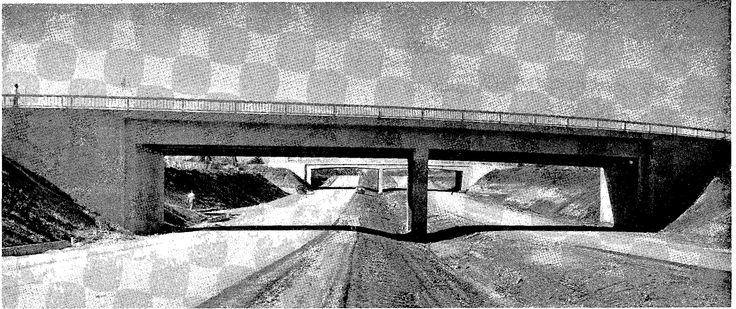
Main Street Overhead in foreground. Separation of U. S. 90 and U. S. 50 routes in background
