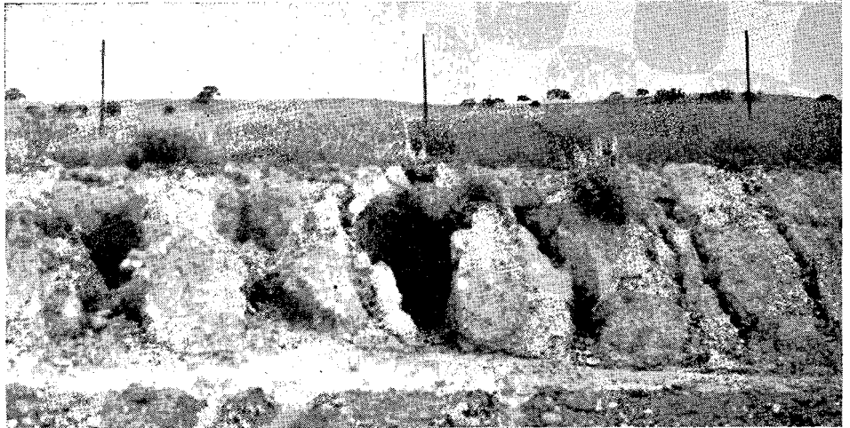
Damage caused by runoff water from adjacent property. (Near Goleta, Santa Barbara County)
