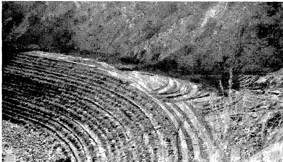
Brush layers and wire reinforced brush mats installed in a fill during construction. These mats have been allowed to protrude too far. Note rock protection at toe of slope. (City Creek Road, San Bernardino County)
