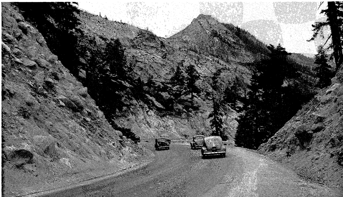
Placerville-Lake Tahoe Forest Highway. An example of roadway sections the Bureau of Public Roads is building in rough country as well as in milder terrain
