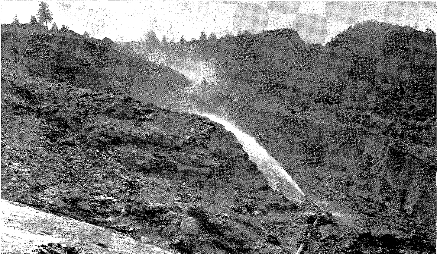
In constructing a highway between Weaverville and Junction City over Oregon Hill in Trinity County, Mr. Haselwood resorted to hydraulicking to level the obstacle. Over 10,000,000 yards of earth were removed in five years by this method
