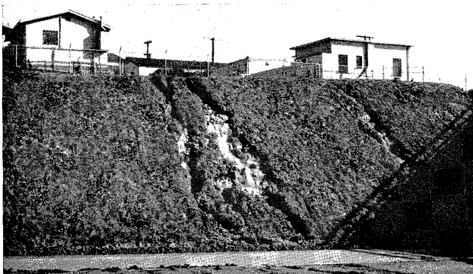
Gullies on a 1½:1 topsoil cut slope caused by runoff from adjacent property. An intercepting ditch and down drain are needed here. (Balboa Freeway, San Diego)
