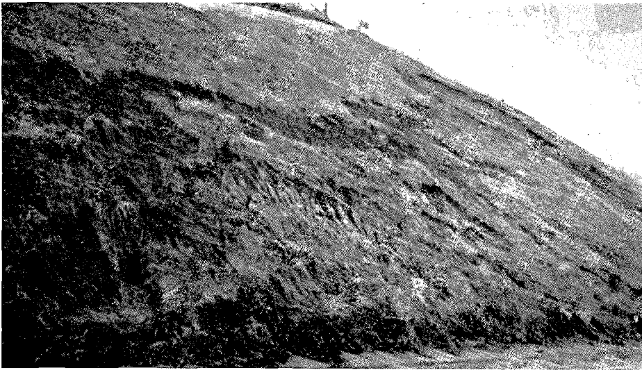
Surface slippage due to saturation caused by a 6-inch rainfall in 24 hours. (Vicinity of Salinas)
