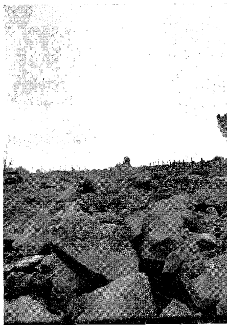
Looking up center line, showing typical construction difficulties encountered for nearly full length of project
