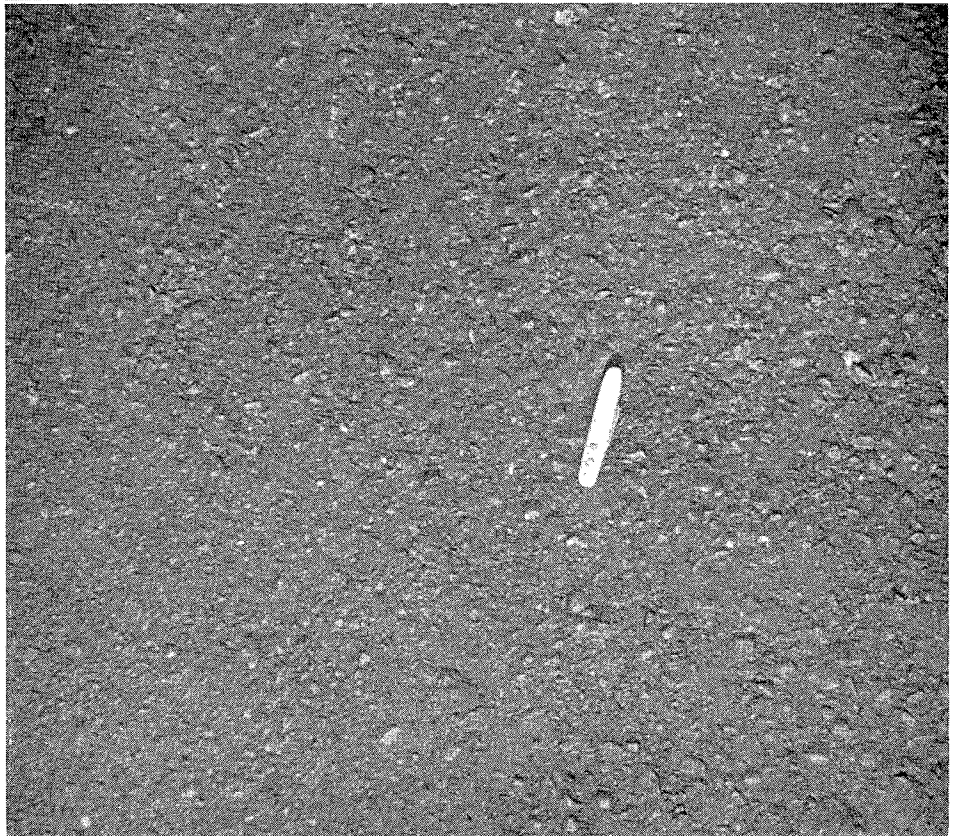
UPPER—Newly scarified pavement. LOWER—Texture of finished pavement. Average depth of pavement was approximately 8½ inches and about 1,825 tons were broken up and processed
