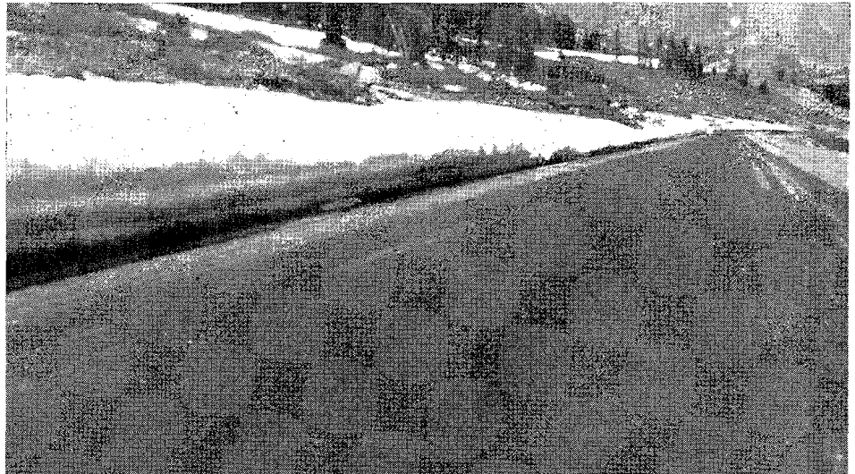
UPPER—Looking east from Station 13 showing melting snow condition, July 1950. LOWER—Looking west where spring appeared in traveled way, July 1950
