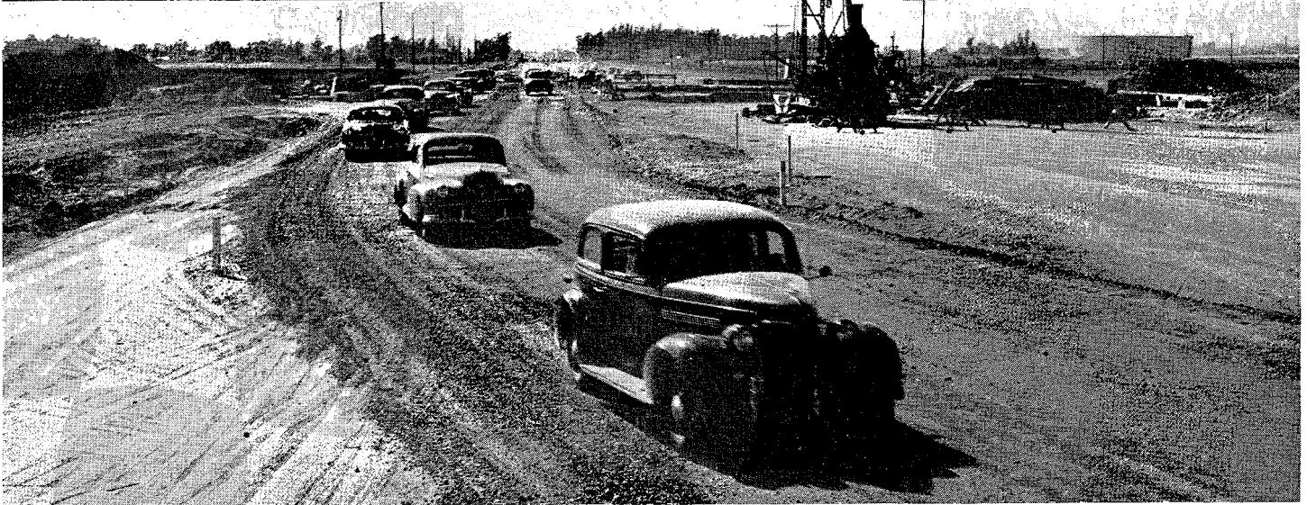
UPPER—Looking northwesterly showing construction under way near Miraflores in Orange County. LOWER—Looking northwesterly showing construction under way near county line
