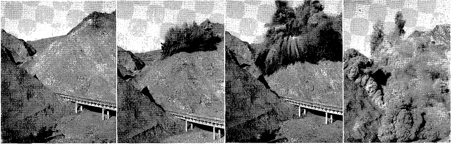
Blasting in Pyramid Cut in Piru Gorge. Left to right—Powder is in place in 350 holes in this cliff. Blast has just been set off. Blast eruption at its height. Huge smoke clouds begin to settle. The highway was closed for only 42 minutes before, during and after the blast when bulldozers cleared the roadway for traffic
