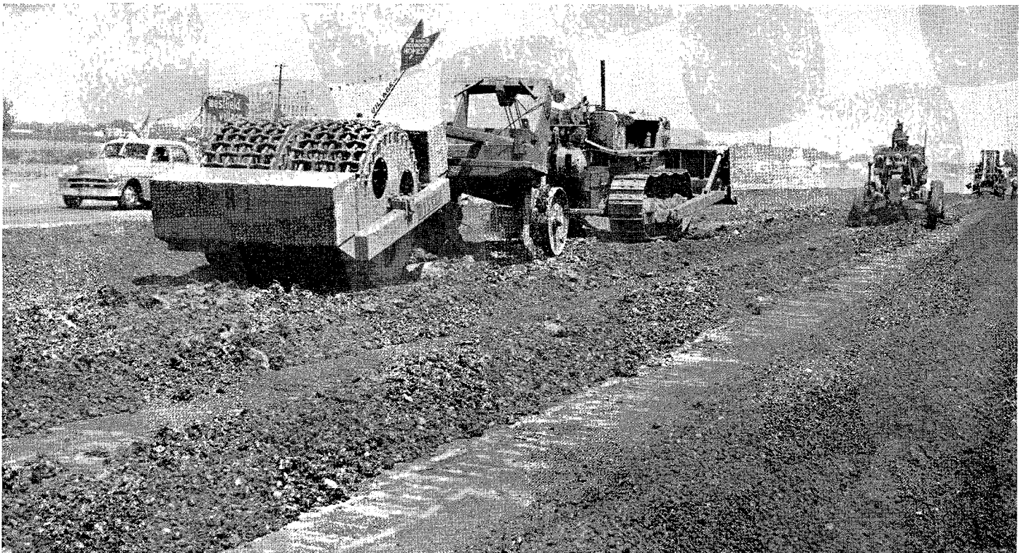
Gridroller and tractor pulverizing and motor grader sizing windrow for Athey loader. Athey loader and crusher operating, extreme right. Note windrow of material crushed by Athey in right foreground
