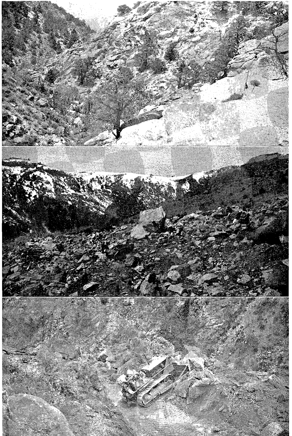
UPPER—Looking west up Slinkard Canyon before blasting. CENTER—After shooting boulders. LOWER—Dozer moving rock after shooting
