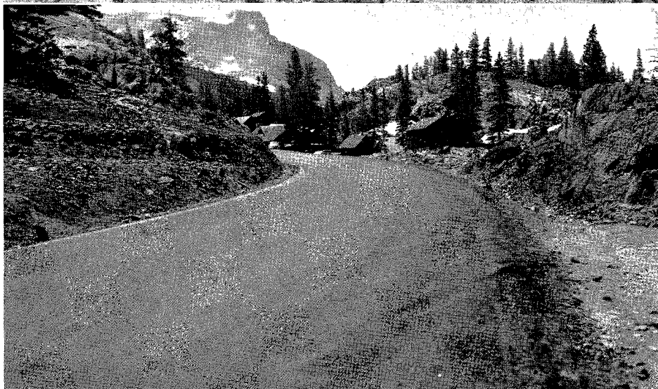
UPPER—Barber-Greene heavy duty travel plant in operation. Tioga Lake in background, 1948. LOWER—Looking west at Camp Tioga. Cut in foreground was one of worst failures before construction due to seeps and winter frost boils. Taken July, 1950 after two winters
