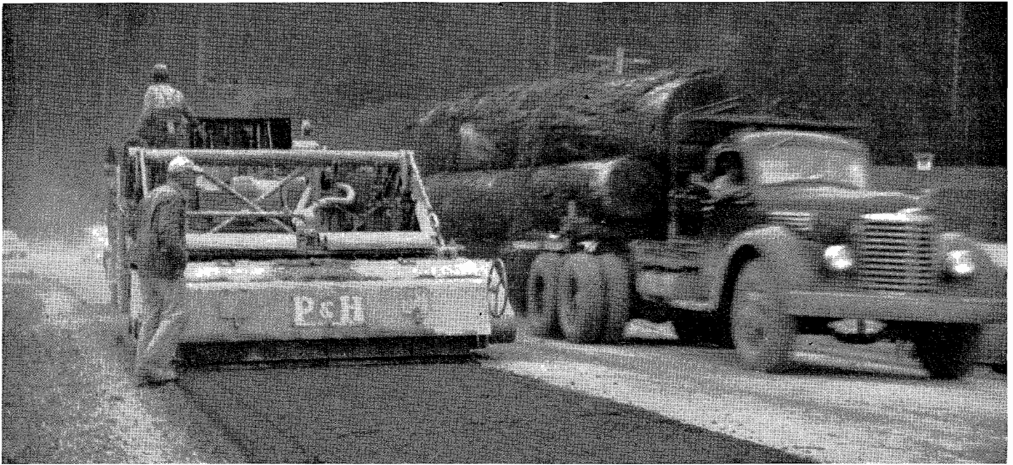
This photo shows the uniform spread of thoroughly mixed cement stabilized base material as the P & H Stabilizer processes 1,275 square yards per hour
