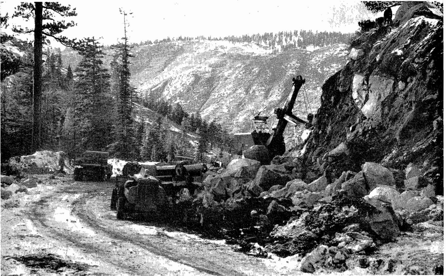
UPPER—Slide on Mt. Diablo Road, State Route 75, in Contra Costa County near Orinda. (Photo by San Francisco Examiner.) LOWER—Heavy equipment clearing U. S. 50 at Camp Sacramento
