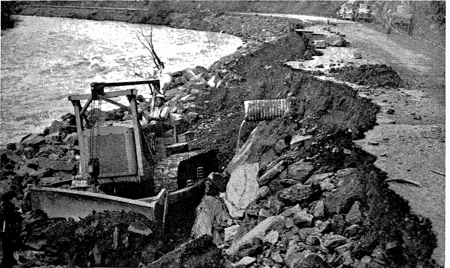
UPPER—Flood damage on Sign Route 140, the All-year Highway into Yosemite Valley, just east of El Portal. LOWER—Bulldozer equipped with Caterpillar diesel tractor at work on Sign Route 140. (Photo courtesy Caterpillar Tractor Company)
