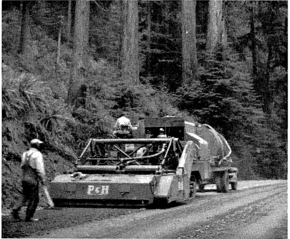
P & H Stabilizer processing cement stabilized base on U. S. 101 near Orick
