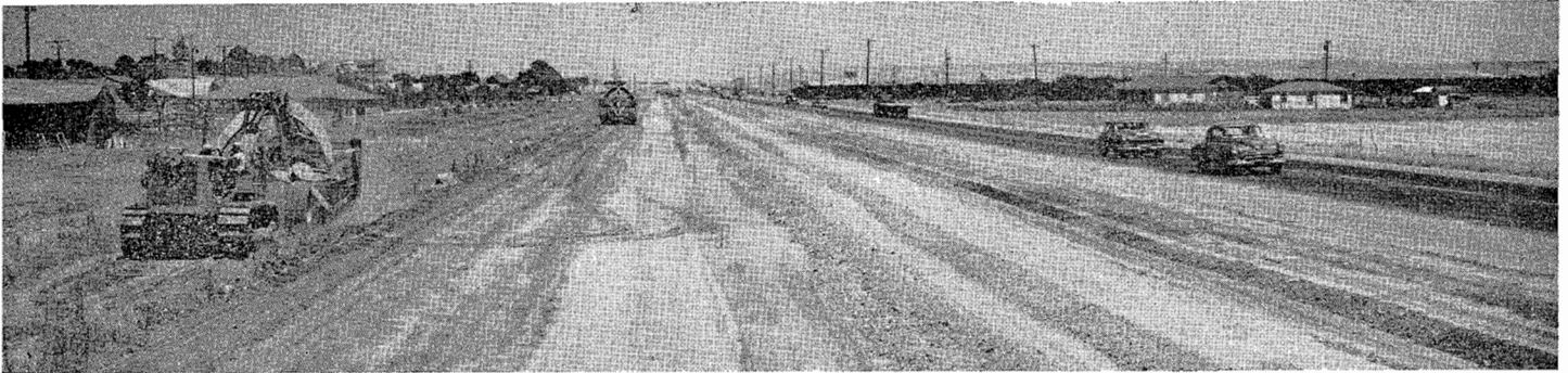
Grading two additional lanes for four-lane divided highway. Looking easterly from Vacaville.
