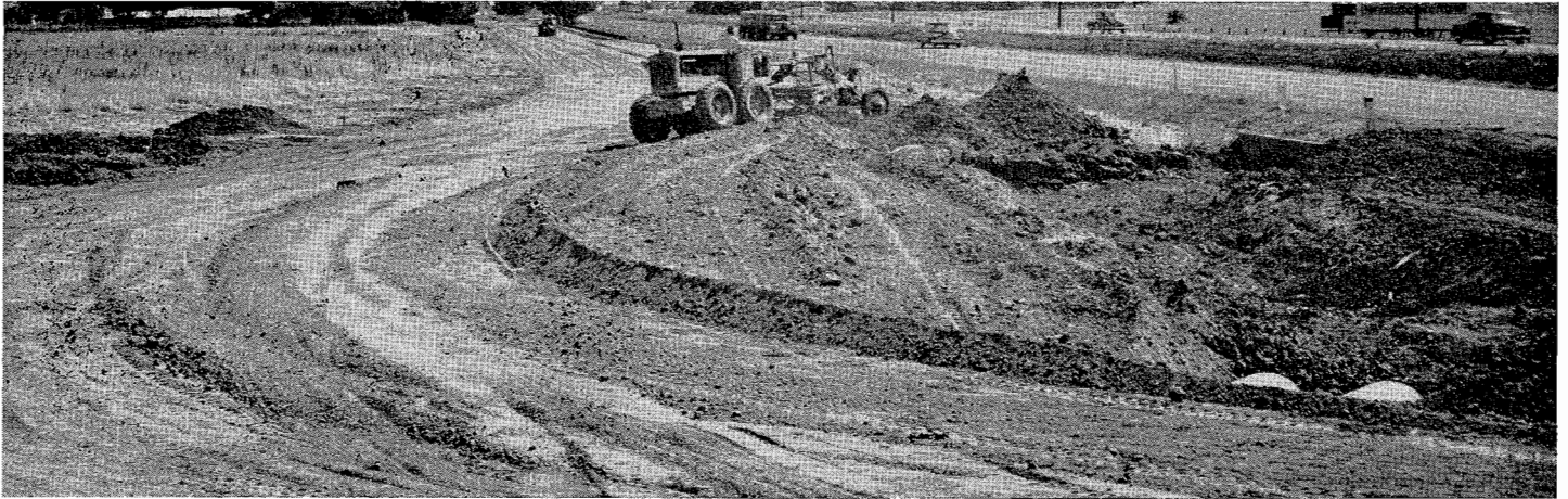
Grading for outer highway near Vacaville-Dixon substation of Pacific Gas & Electric Company
