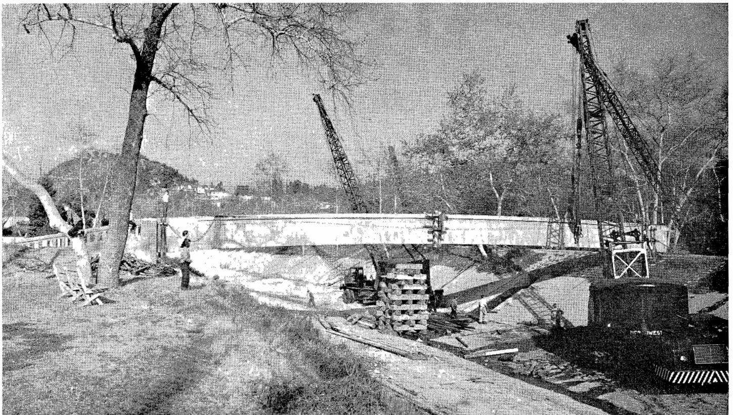
Arroyo Seco Channel Pedestrian Bridge in Los Angeles. Prestressed girder shown has just been hoisted into final position on abutments. Temporary steel cables on exterior of girder for rigging purposes only.
