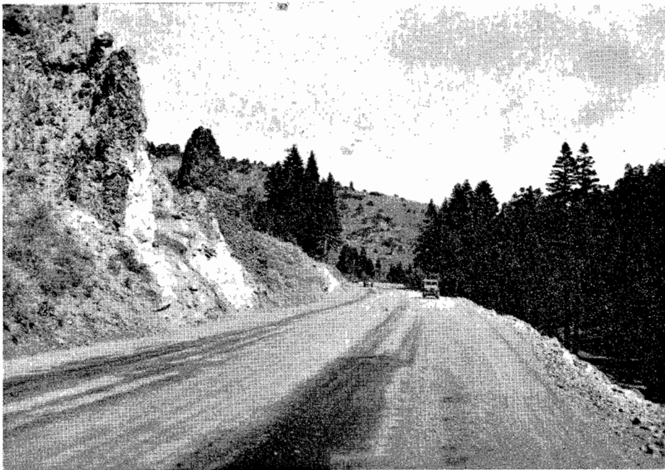
Near the summit of Bonner Grade after grading operations. This is the same section as shown in the photo on page 39
