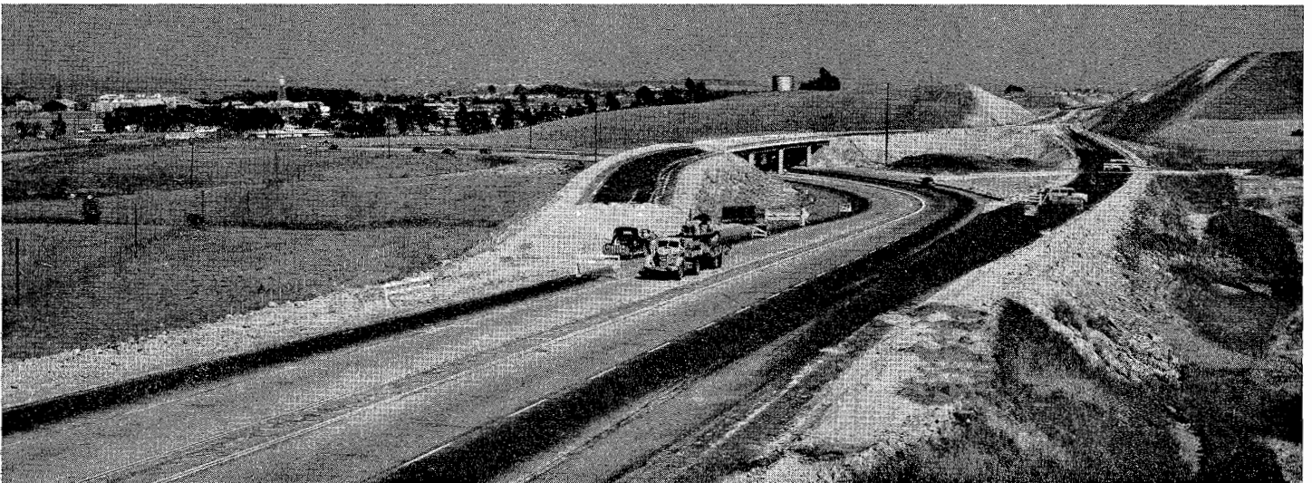
Connection to Port Chicago Road at beginning of project. Grade separation structure provides for the free merging of westbound traffic.
