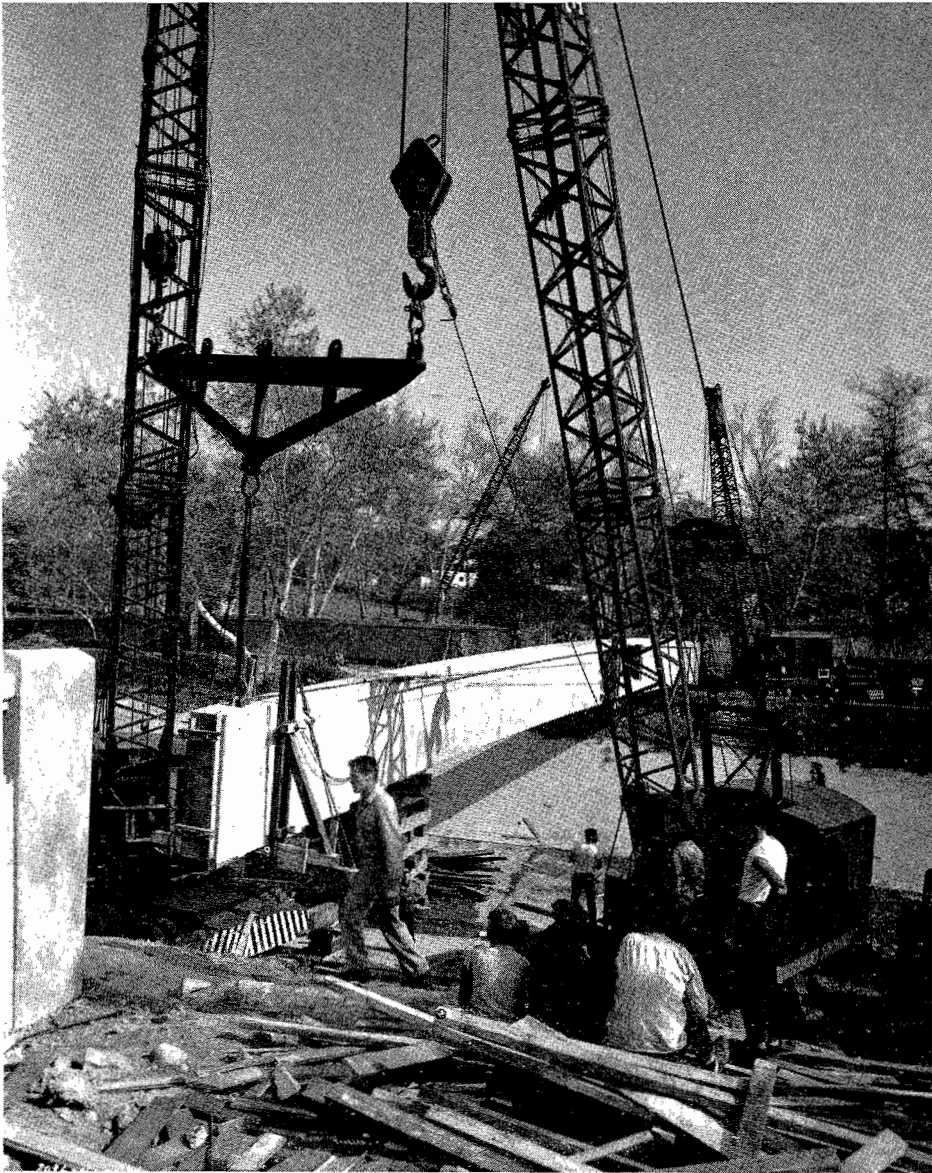
Downstream girder being hoisted onto abutments; upstream girder still in parking lot in background
