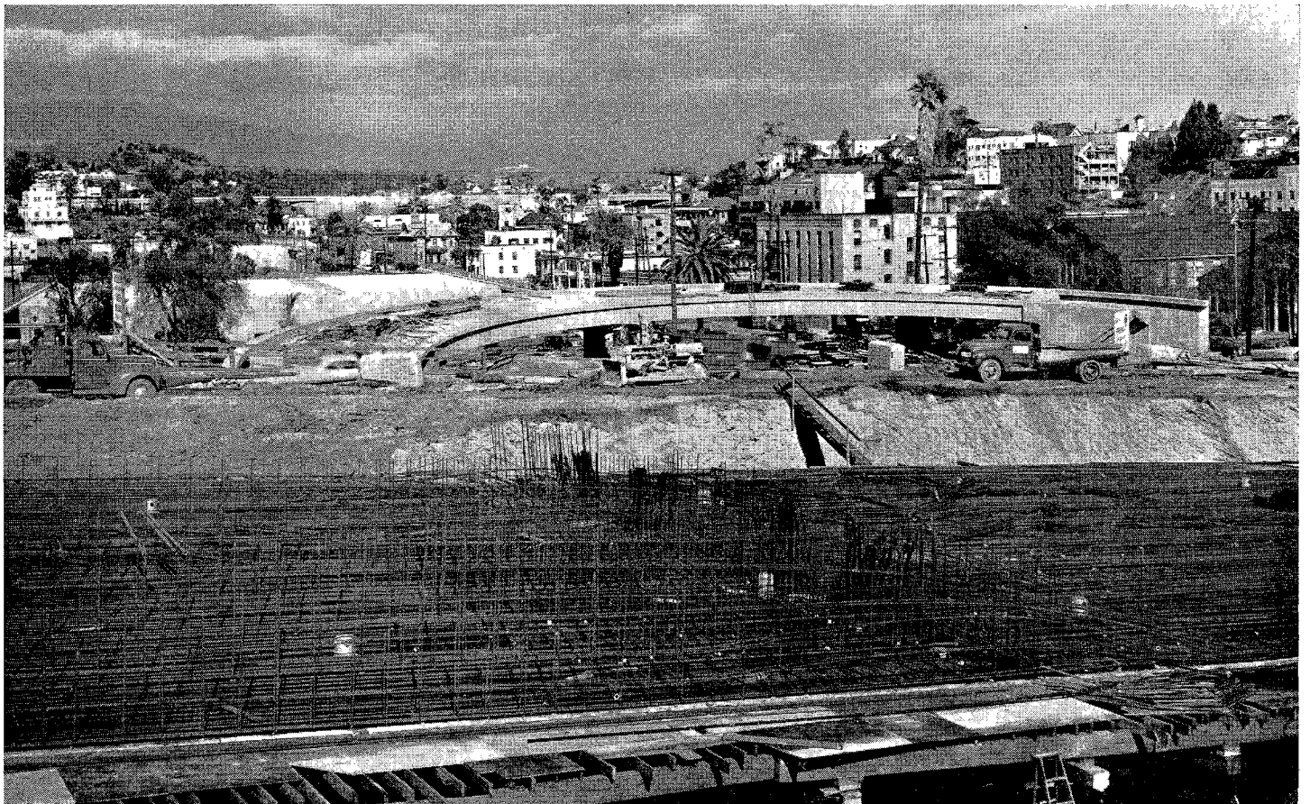
Looking northerly showing Harbor Freeway construction with steel in place for bridge deck of Third Street overcrossing grade separation in front foreground. The curving ramp bridge for traffic entering the Harbor Freeway southbound is shown in middle foreground. In background to the left is the four-level grade separation.
