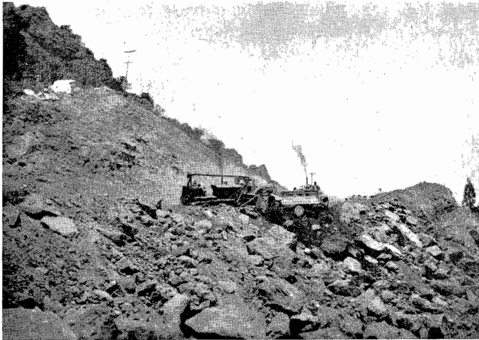
This picture graphically illustrates the rugged terrain in which bulldozers had to work on new alignment
