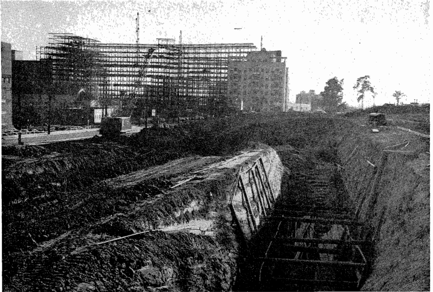
Looking southerly on Harbor Freeway showing in foreground excavation for east abutment of Sixth Street overcrossing grade separation. To the left is shown the steel framework of the Statler Center Hotel.
