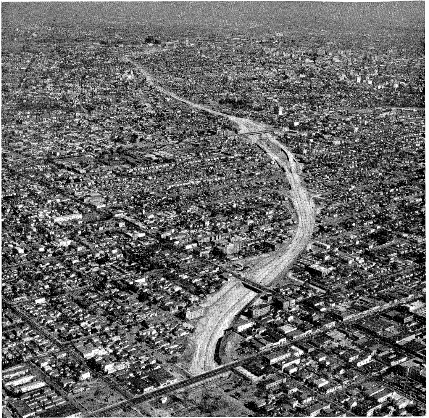
Aerial view of Hollywood Freeway, looking southeasterly and taken from above Western Avenue, showing in the foreground work under construction between Western Avenue and Virgil Avenue, with completed portion of freeway in background
