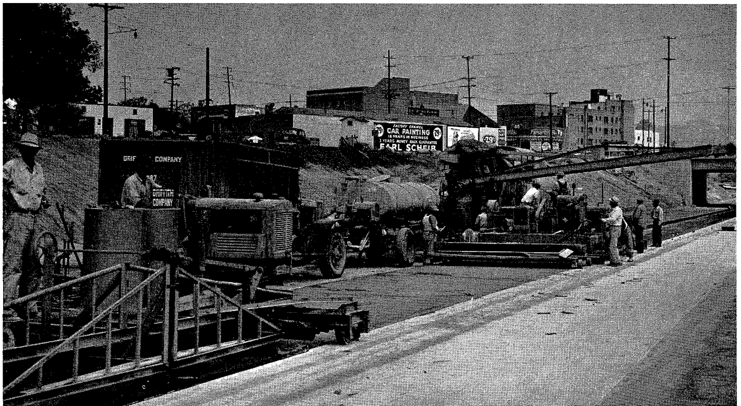
Paving machines in operation. Pouring and finishing work east of Western Avenue.
