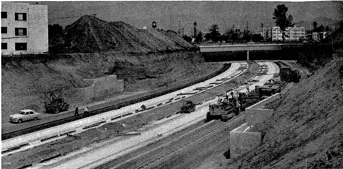
Looking west toward Western Avenue crossing, showing final roadbed preparation for pouring operations
