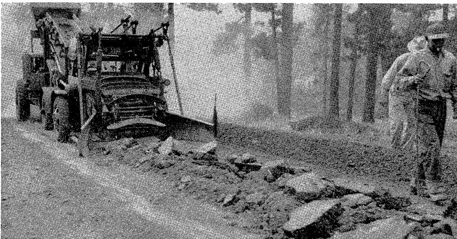
Combination loading and breaking equipment picks up and pulverizes hardened bituminous pavement in the process of remixing and stabilizing
