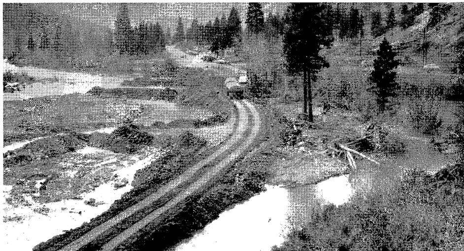
Emergency replacement and protection at washout on U. S. 40 east of Truckee last winter. First consideration is for the safety and resumption of traffic.
