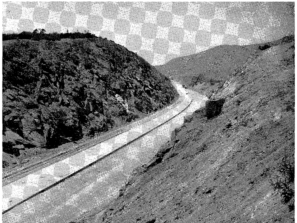
New alignment of U. S. 80 east of Alpine. Construction and paving operations.
