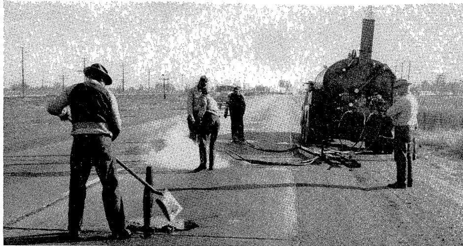
By increasing capacity of asphalt heating unit, subsealing can be done by two nozzlemen simultaneously
