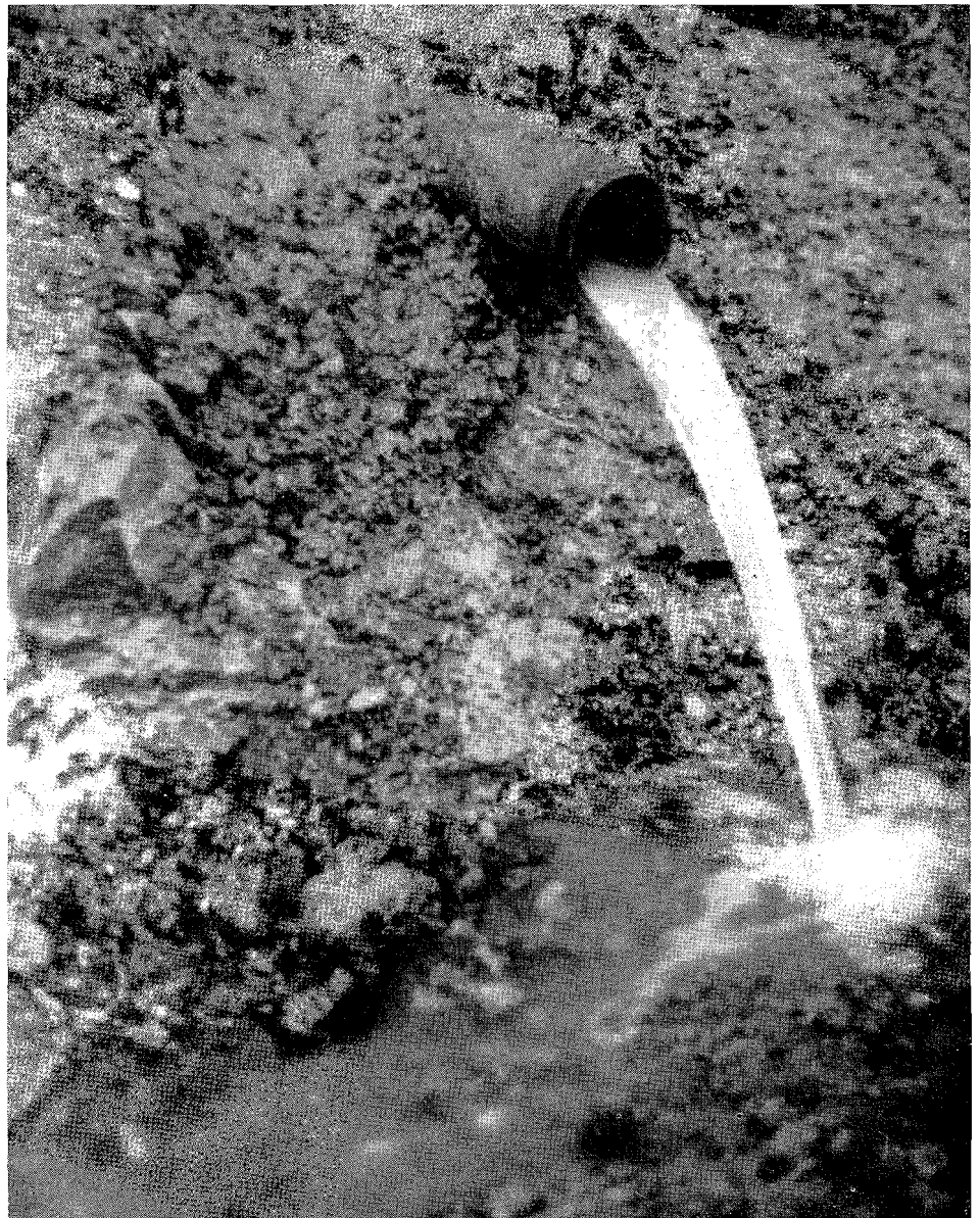
Drain at roadway level flowing 36,000 gallons per day
