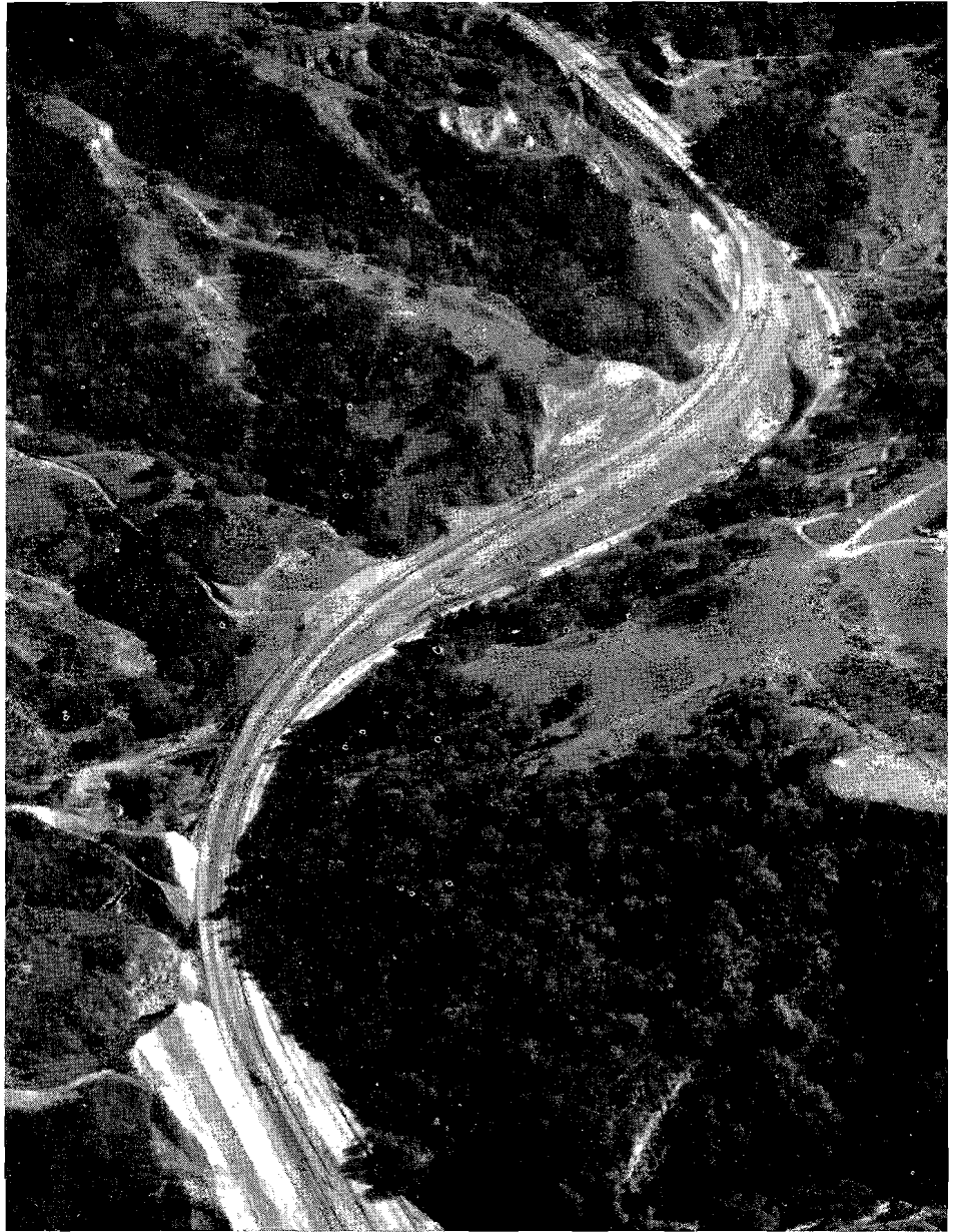
Aerial view of construction of divided highway in Weldon Canyon section of Ridge Route
