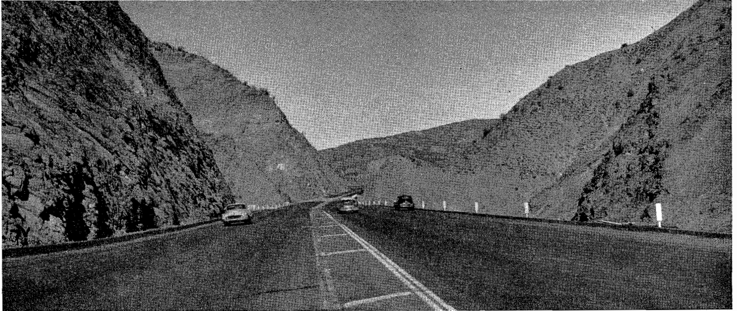
UPPER—Looking south from Pyramid Cut, showing completed roadway with channel change on left. LOWER—Looking northerly along completed Ridge Route in Piru Gorge.
