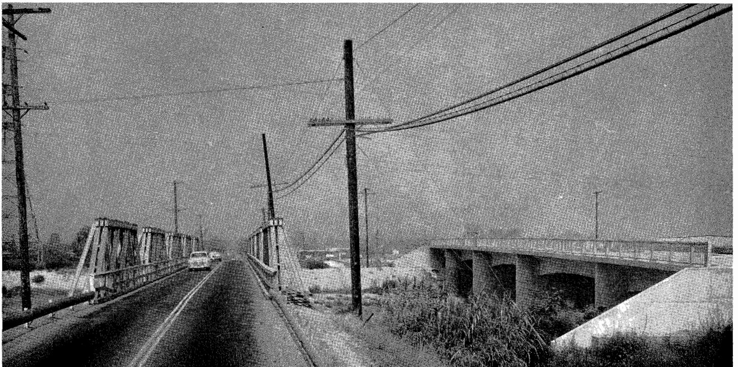
Bridge 13—Old narrow bridge over San Gabriel River on Center Street (F. A. S. Route 835) with new four-lane reinforced concrete bridge under construction on right
