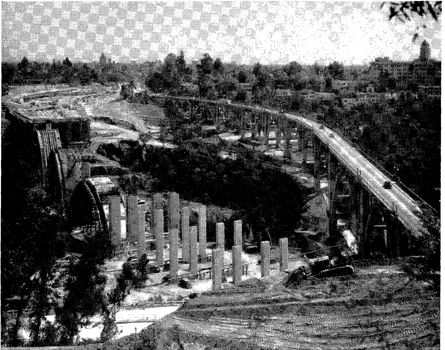
Looking easterly across Arroyo Seco, showing old Colorado Street Bridge on right and new construction in progress on left for the Colorado Freeway Bridge. Buildings in business district and civic center of Pasadena show in background.
