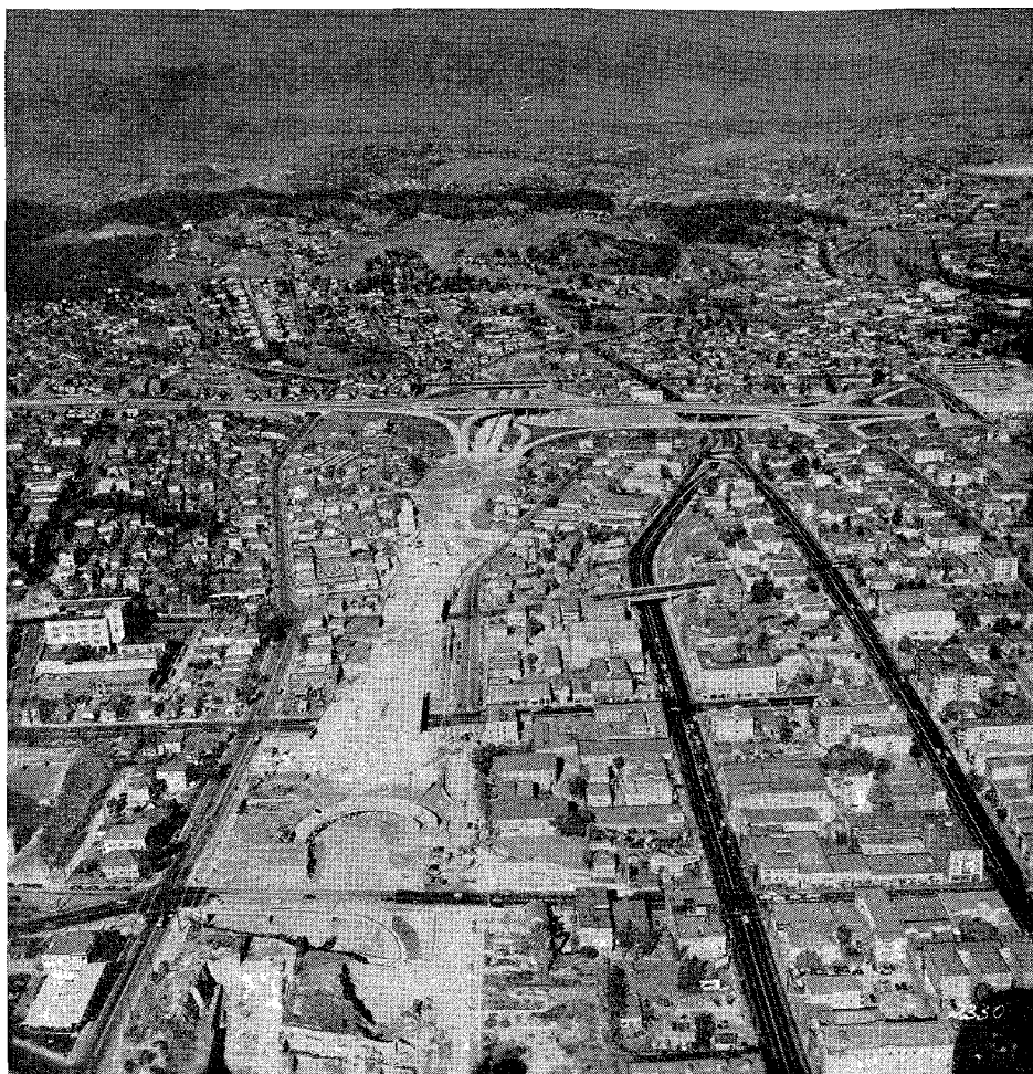
Looking northerly along Harbor Freeway construction between Beaudry Avenue on the left and Figueroa Street on the right. The four-level grade separation structure and the Hollywood Freeway appear in the central part of the photograph with Pasadena in the background. The completed construction in the foreground is the Third Street Overcrossing.
