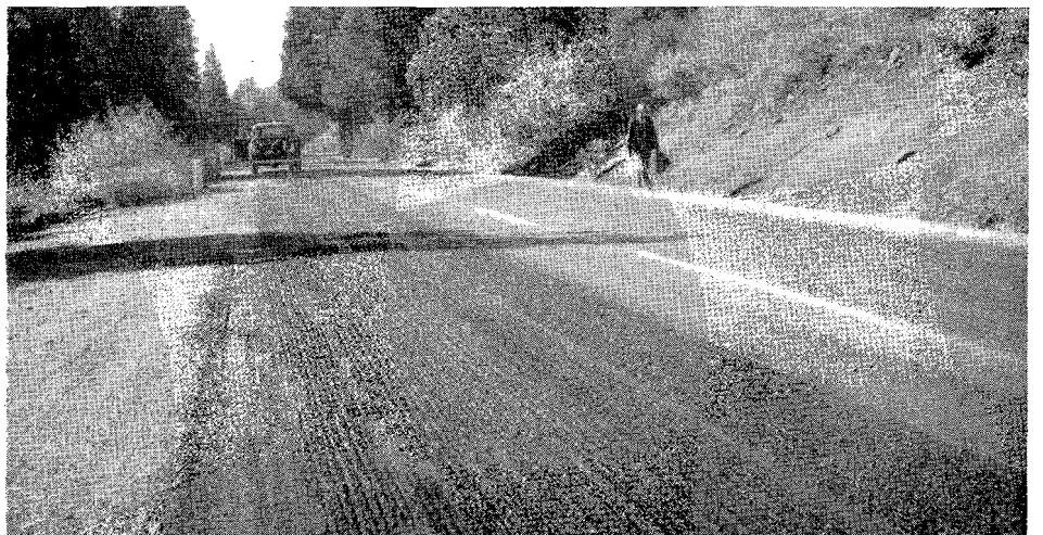
UPPER—Heating and raking equipment used on U. S. 40 in District III. CENTER—Top of burner and spike drag used in District II. LOWER—Portion of U. S. 40 treated by heating and raking.
