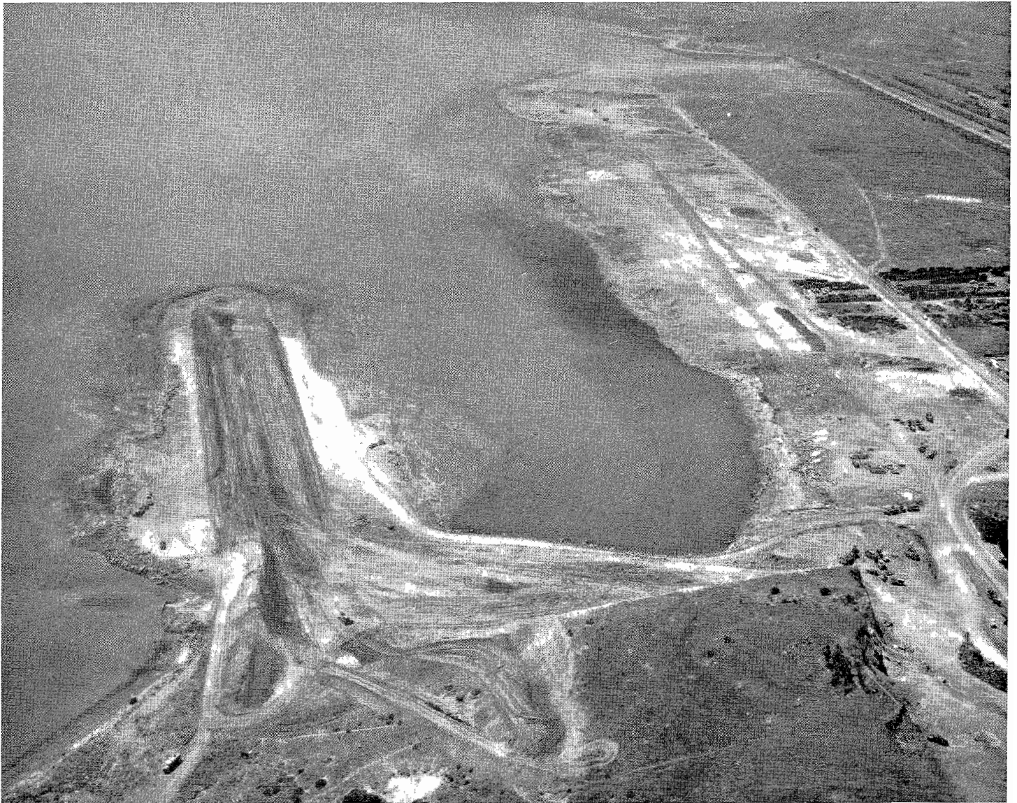
Aerial view of experimental fill looking south from Candlestick Point toward Sierra Point, the ultimate terminus of the open-water fill
