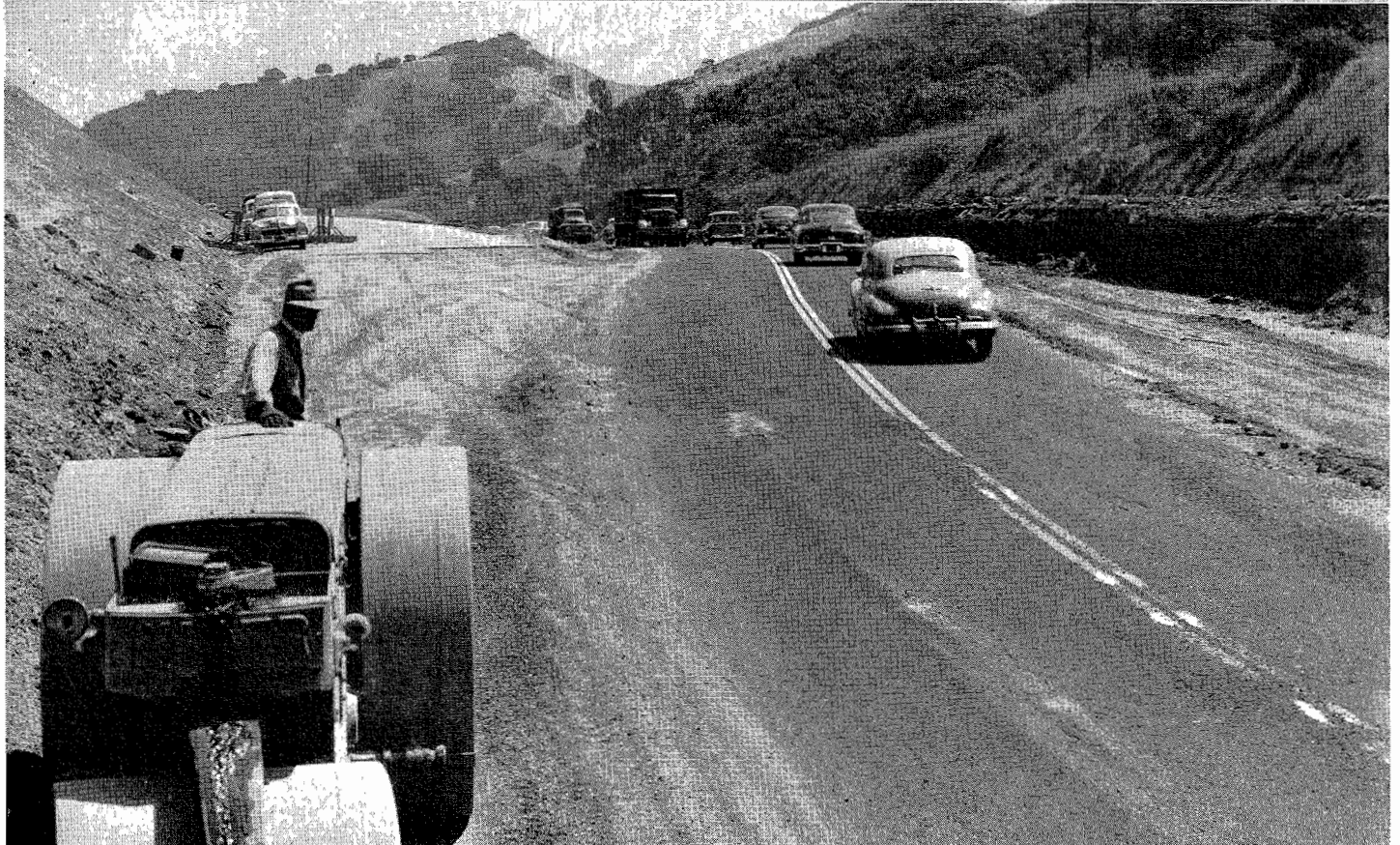
UPPER—New alignment one mile west of State Route 21 and Dublin. LOWER—New construction in same area.
