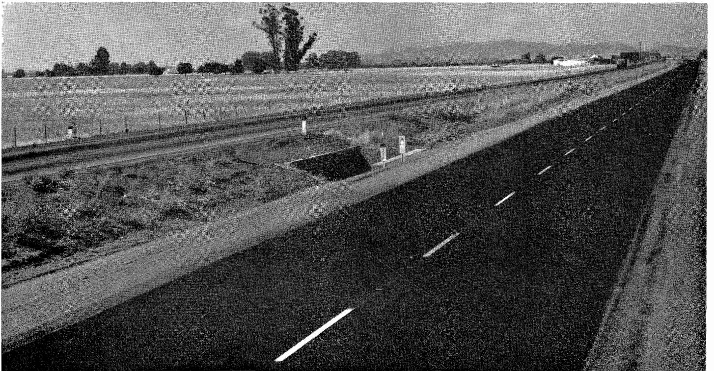
Recently completed resurfacing of U. S. 40 near Vacaville with a bituminous mixture
