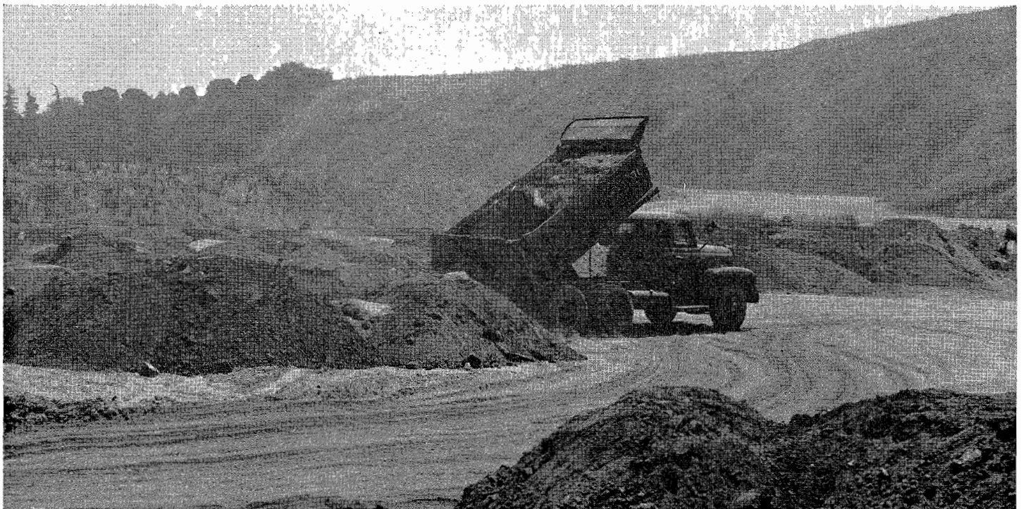
Truck depositing waste material from Santa Ana Freeway excavation now in progress for the Alameda Street overcrossing. Dumping operations where shown are at the 585-foot level of the Bishops Road disposal area. Trees in left background are in Elysian Park. The top of the ridge is at approximately 675-foot elevation, and this ridge is the southwest property line of the Bishops Road disposal area.
