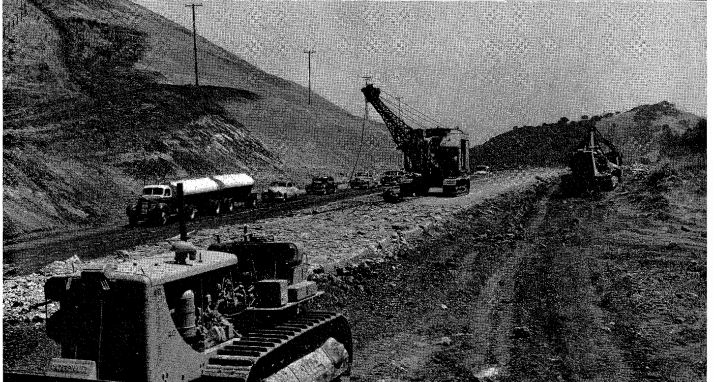
Heavy equipment working on construction one mile west of State Route 21 and Dublin
