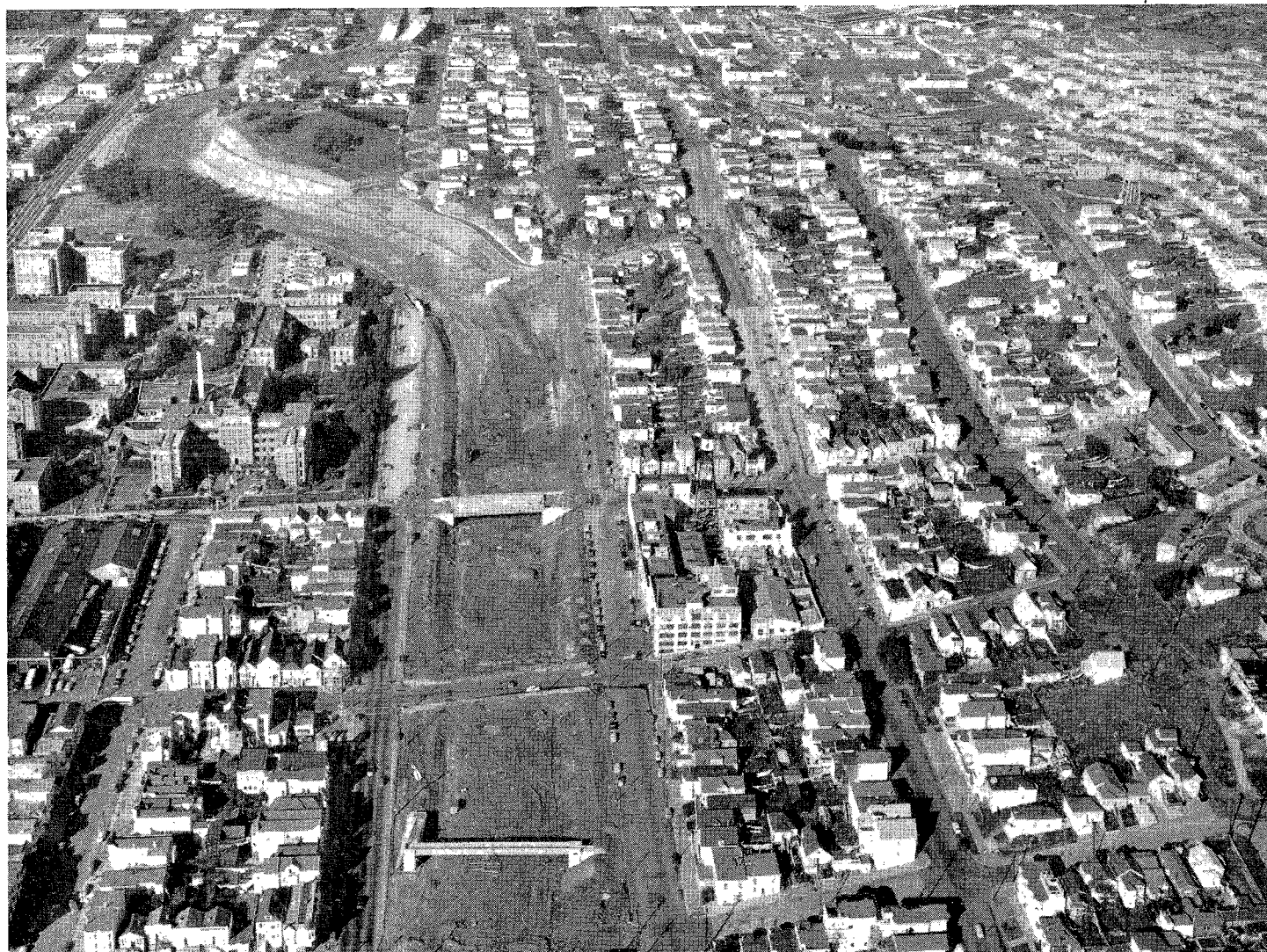
Looking northerly from Army Street showing progress of freeway construction from Army Street to 17th Street. Twenty-fifth Street pedestrian overcrossing and 23d Street vehicular overcrossing visible in foreground. Steel viaduct construction now in progress is visible in background.
