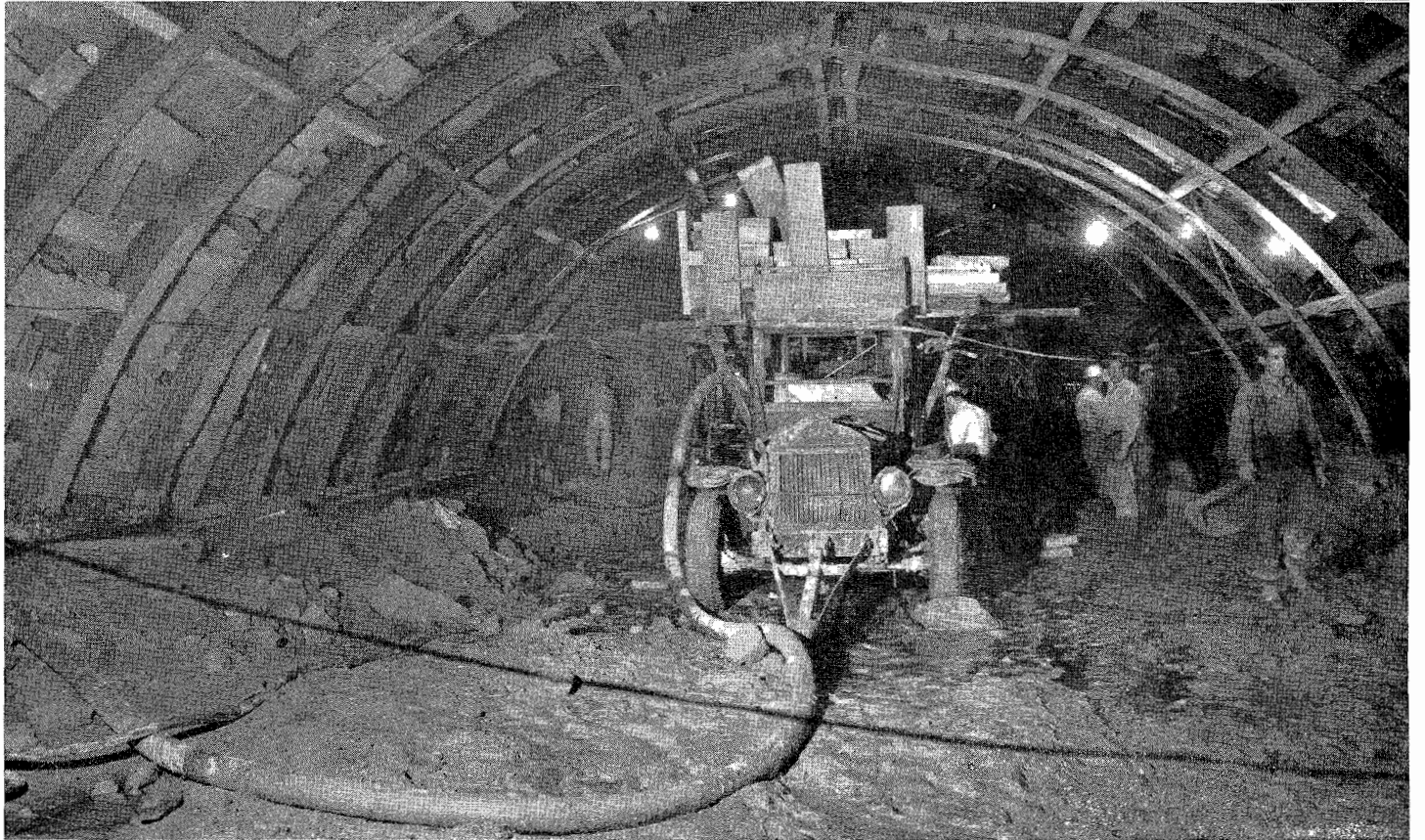
UPPER—South portal showing the timbered left and right wall plate drifts. Unstable rock above the right drift necessitated the construction of two oversize square sets. LOWER—Scene at the face of the heading showing the drill jumbo in the center. To the left of center can be seen the wall plate upon which the steel segment is secured. Miner at left is setting up to drill the left wall plate drift.
