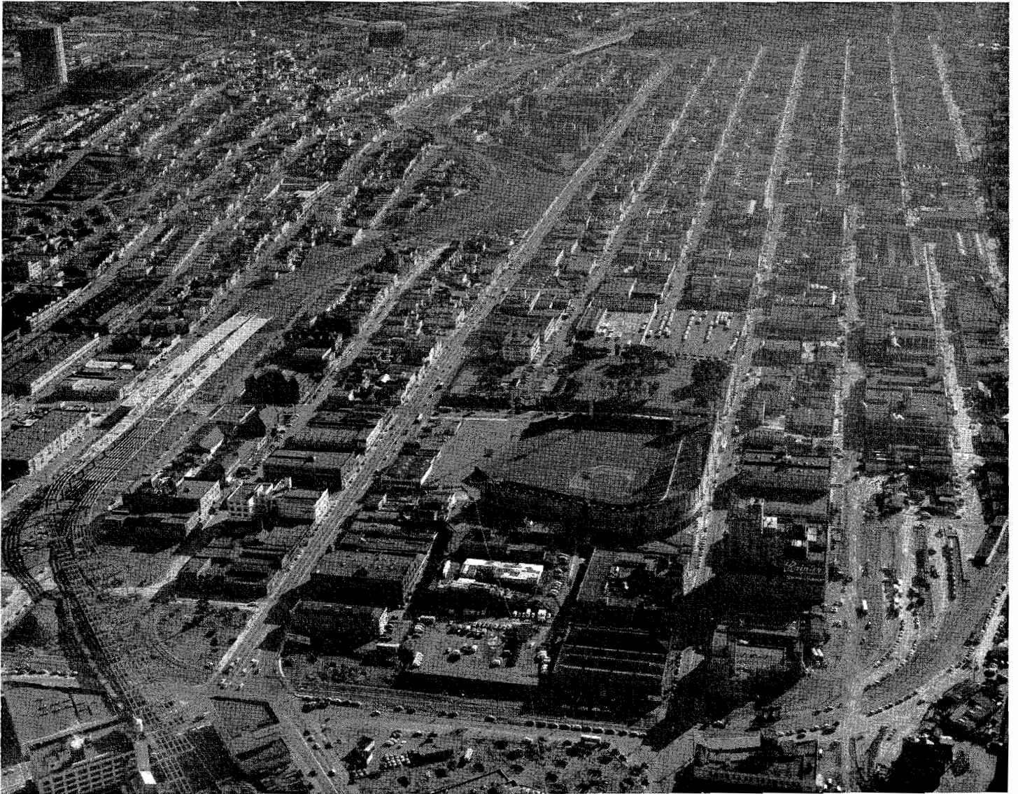
View looking southerly showing freeway under construction between Bryant Street and Army Street in San Francisco. Steel for Ninth and 10th Streets off ramps in foreground. Portion of completed freeway visible in background.
