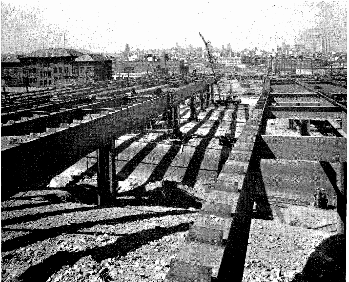
View looking northerly across 17th Street showing steel superstructure under construction. Site of Division Street interchange in background.
