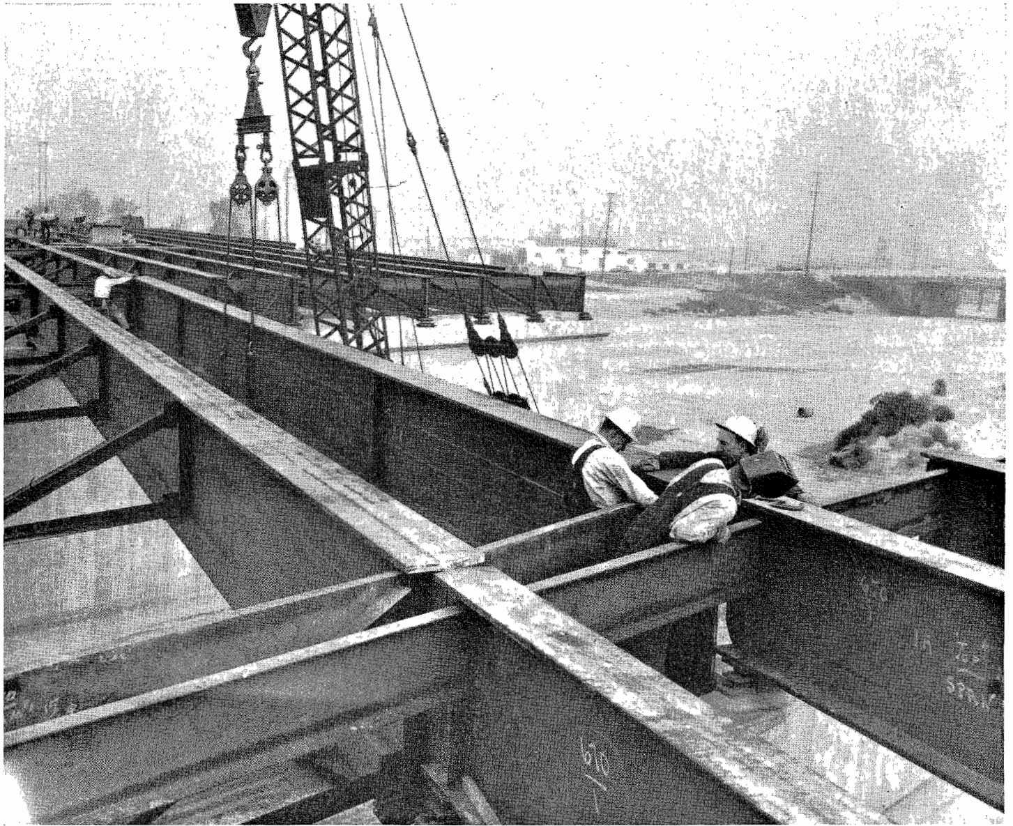
Erecting steel beam in span seven. Photo by Ray Graham, Los Angeles Times
