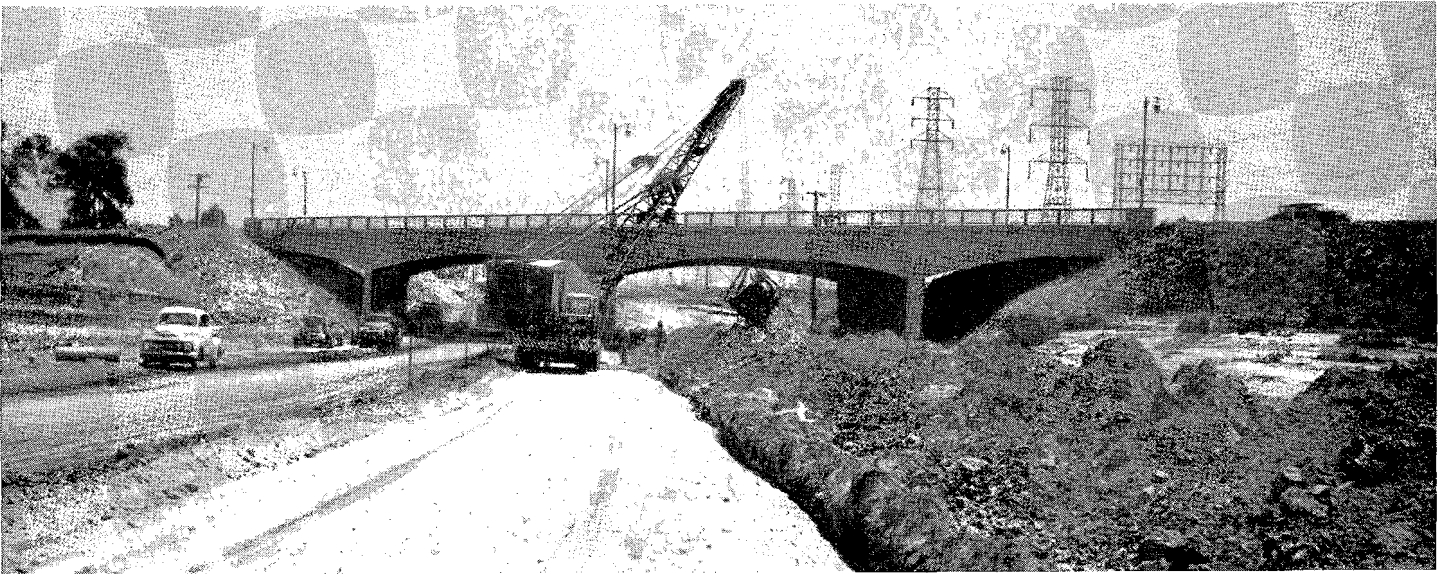
Looking northerly along Long Beach Freeway showing construction operations in vicinity of Long Beach Boulevard Bridge which was designed and built under supervision of the City of Long Beach
