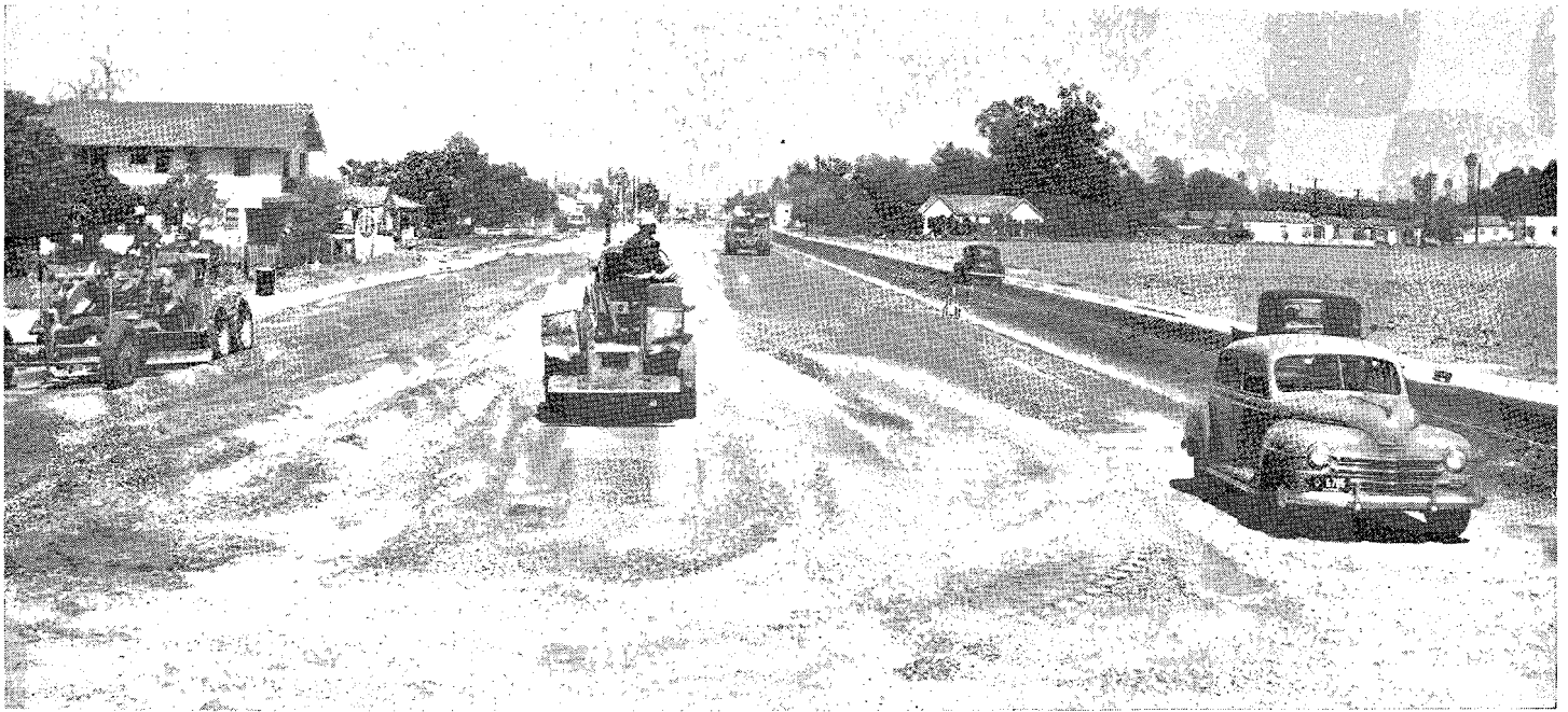
Artesia Street looking easterly showing typical construction operations now in progress between Alameda Street and Long Beach Boulevard
