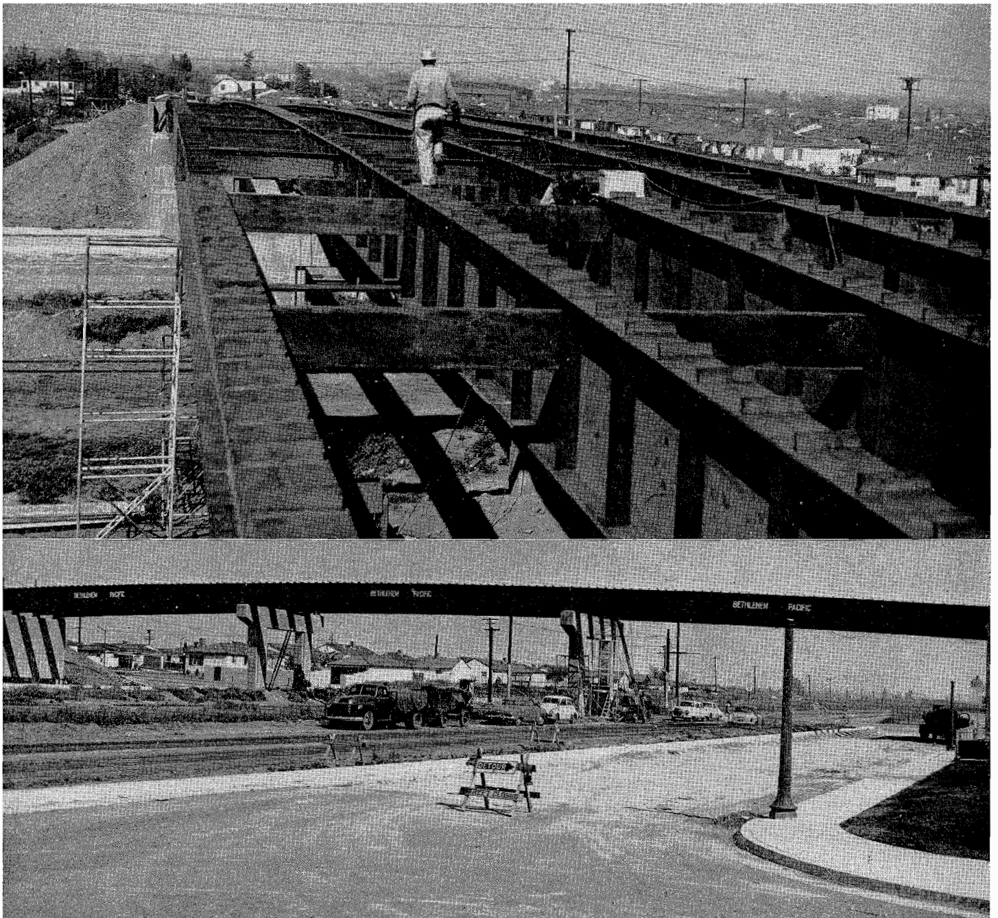
UPPER—All structural steel in place and field welding of diaphragm connections under way. Note welded shear lugs on top flanges of girders. LOWER—Side view looking northeasterly showing all three spans of steel in place.
