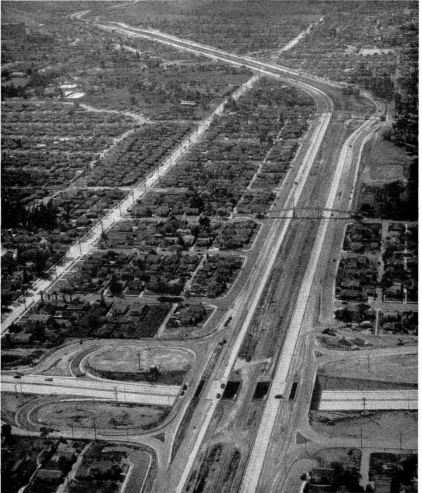
Aerial view looking westerly along Ramona Freeway, showing construction in progress. The grade separation in background is at Atlantic Boulevard. Completed section of this freeway recently opened to traffic from Fremont Avenue to Eastern Avenue is shown in background.
