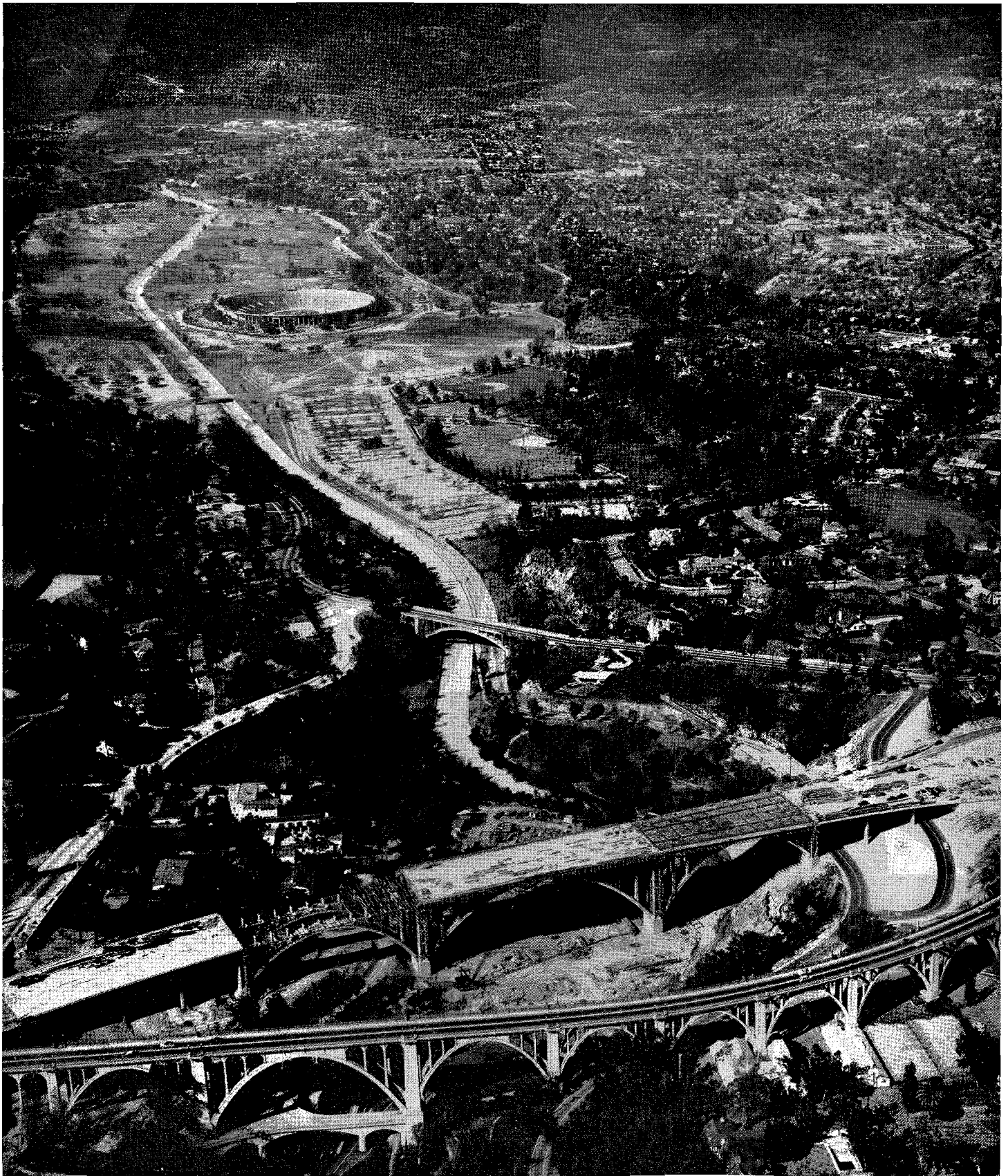
Looking northerly up the Arroyo Seco showing in foreground the old two-lane Colorado Street Bridge built in 1912 and the new Colorado six-lane freeway bridge under construction. The famous Rose Bowl will be seen upper center, left. Northwestern portion of Pasadena and community of Altadena shown in background.
