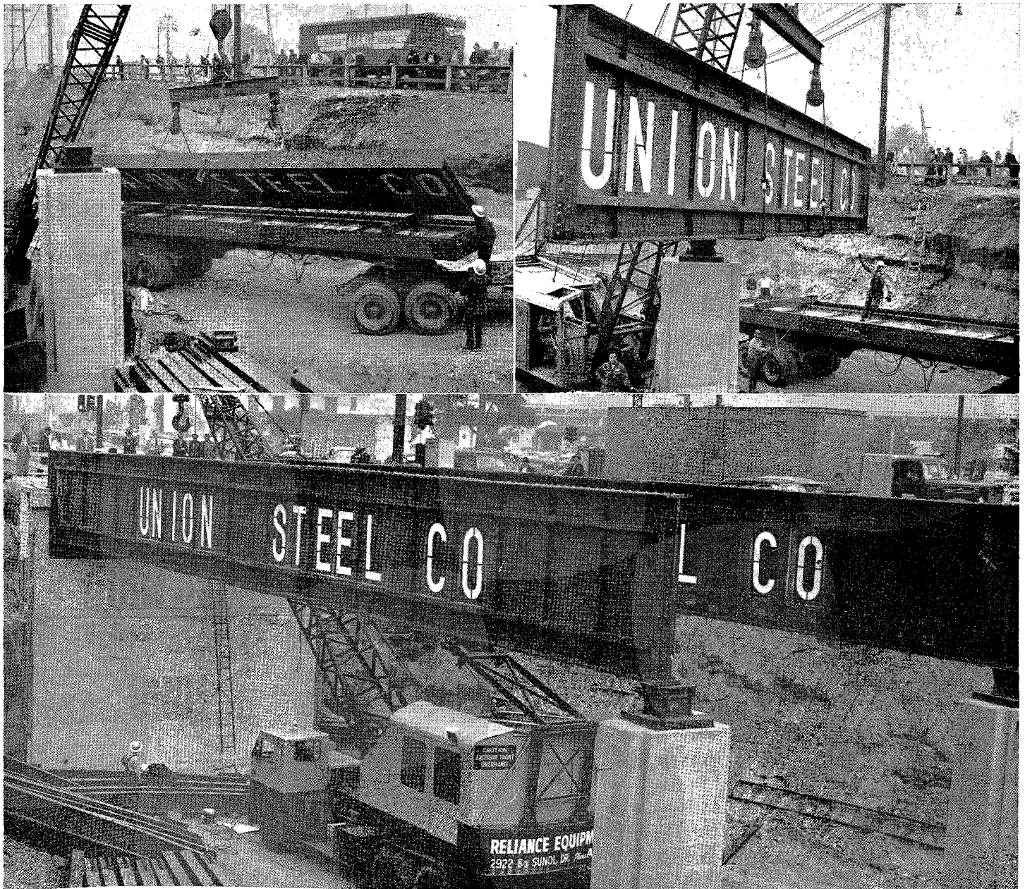
UPPER LEFT—Raising steel girders from truck to place on piers. Note great number of sidewalk superintendents. UPPER RIGHT—Swinging girder into position. LOWER—Girders for first span in final position. Note Los Angeles Union Station in background.
