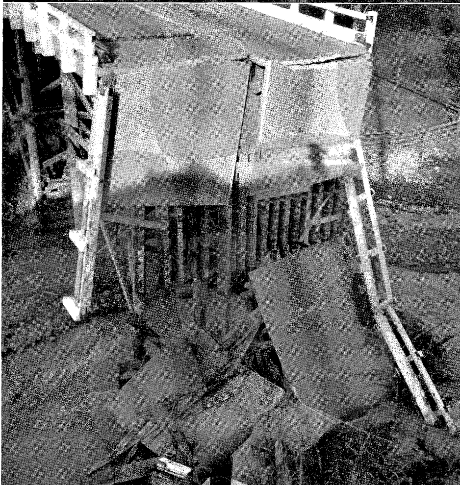
Washed out bridge at Gilbert Creek two miles south of Oregon state line on Roosevelt Highway
