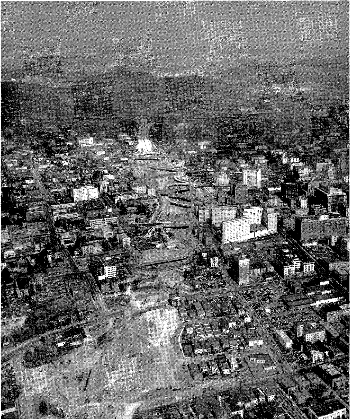
Looking north along Harbor Freeway, taken from above Olympic Boulevard. Construction in progress is shown between Ninth Street and Third Street. Statler Hotel will be noted center right and four-level interchange structure in background.
