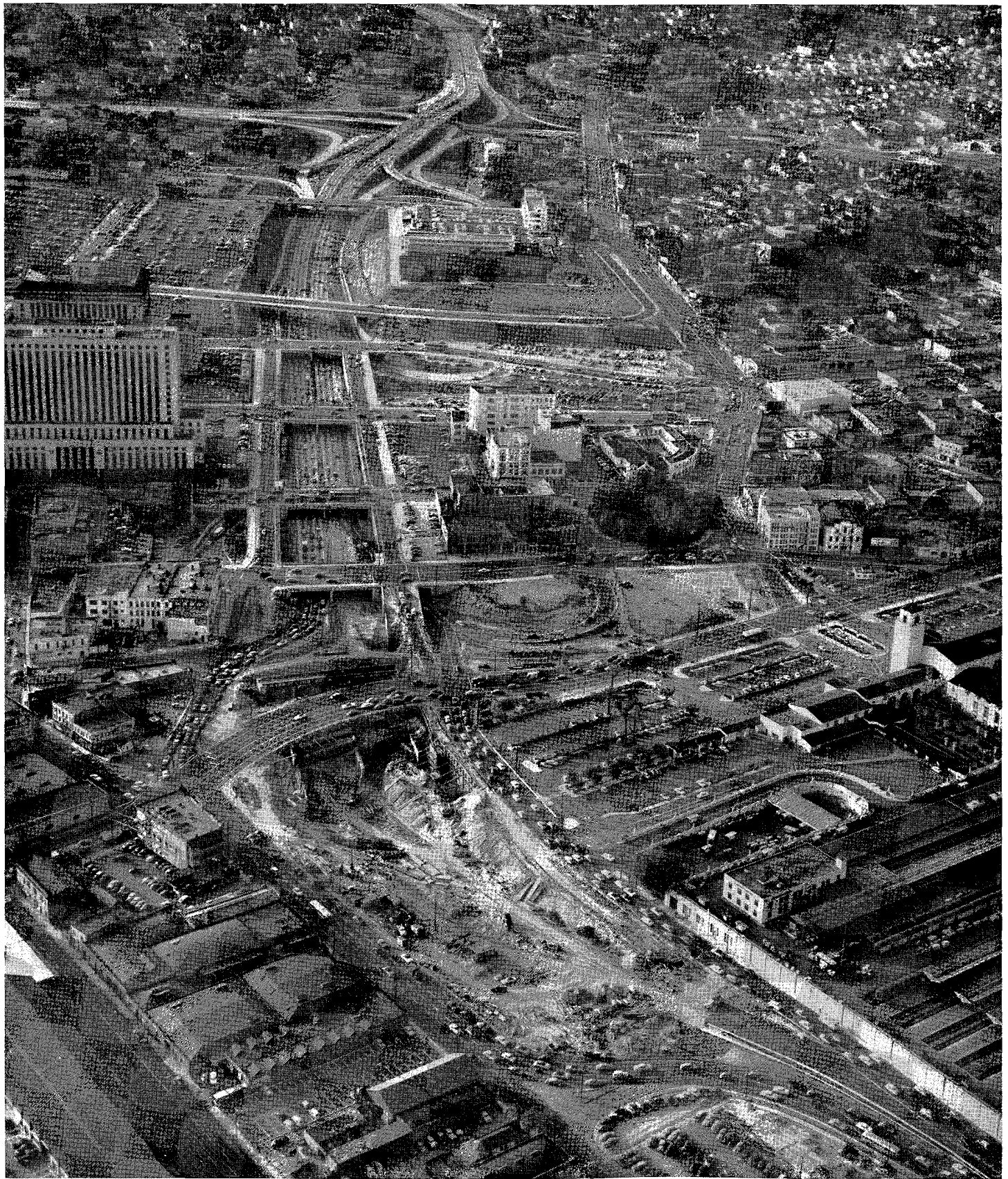
Aerial view looking westerly along Santa Ana-Hollywood Freeway. Los Angeles Civic Center area foreground. Heavy traffic using detours around site for Alameda Street grade separation under construction. Los Angeles Union Railroad Station shown foreground right. Federal Building and other Civic Center buildings shown center left. Four-level interchange structure in background with Harbor Freeway extending to the left and Arroyo Seco Parkway to the right.
