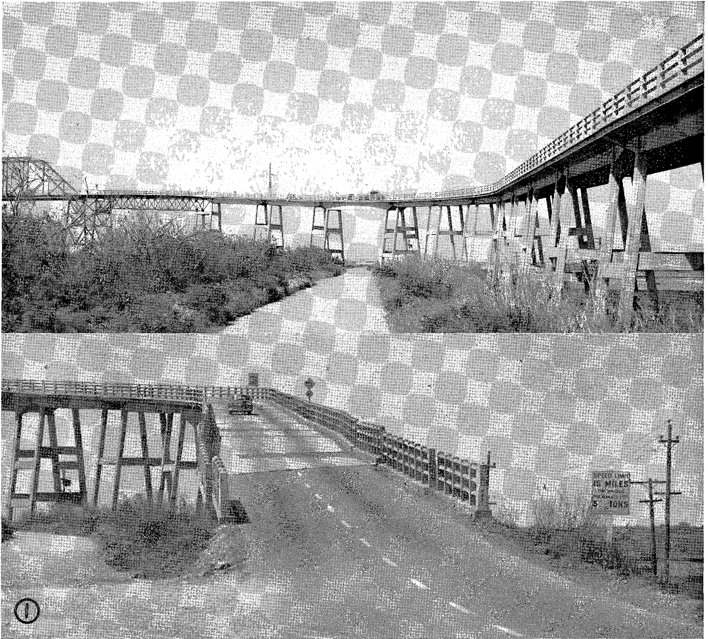
UPPER—Looking west along levee road. General elevation of north approach trestle looking west along top of levee. LOWER—Contra Costa County, Route 11, Antioch Bridge, roadway view looking west.
