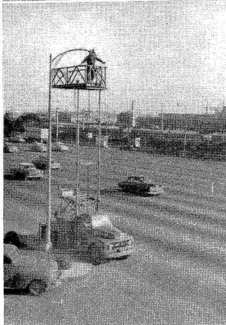
Hydraulically-raised truck-mounted lift, used in maintaining high voltage freeway lighting systems
