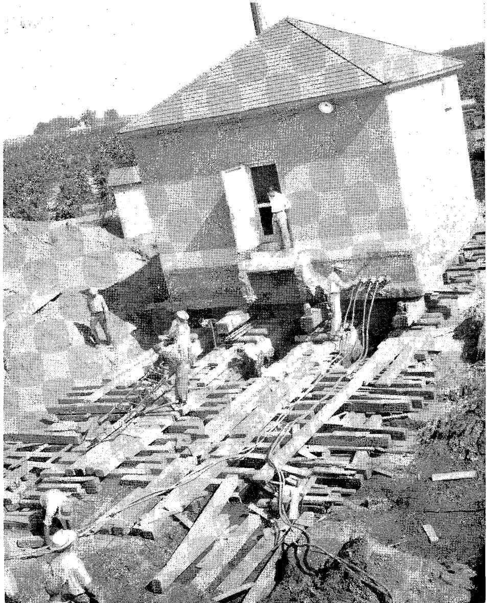
Moving Pacific Telephone & Telegraph Company's repeater station
