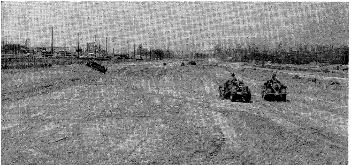
View looking westerly along Camarillo Freeway from near Arneill Road showing grading operations in progress. Existing state highway shown on left with frontage road and housing development operations on right.
