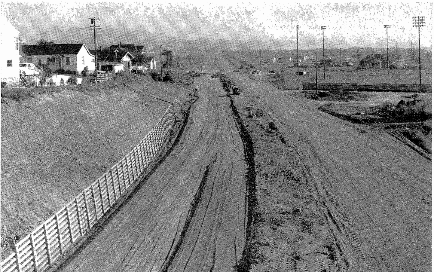
Looking south from 11th Street crossing showing cribbing on left. Highway lighting will be installed at intersection in middle distance
