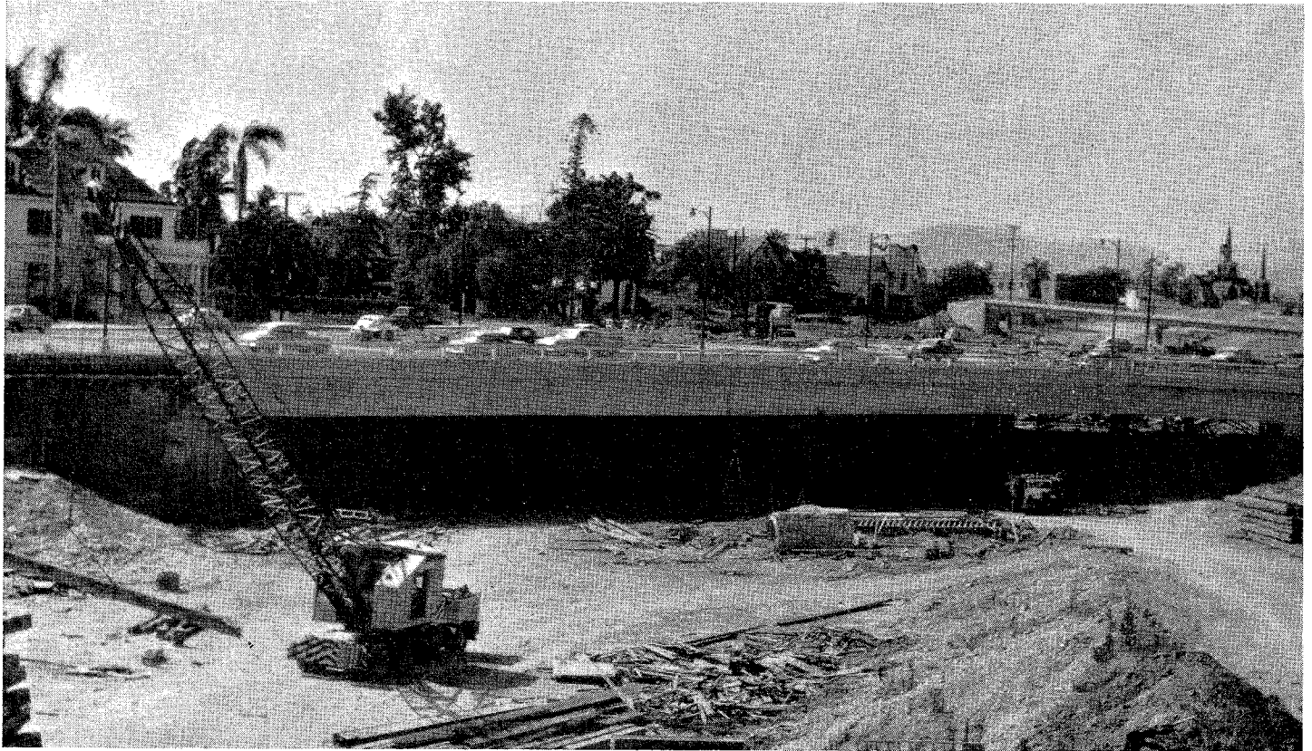
Looking northwesterly along Harbor Freeway construction, showing nearly completed Figueroa Street bridge at 23d Street
