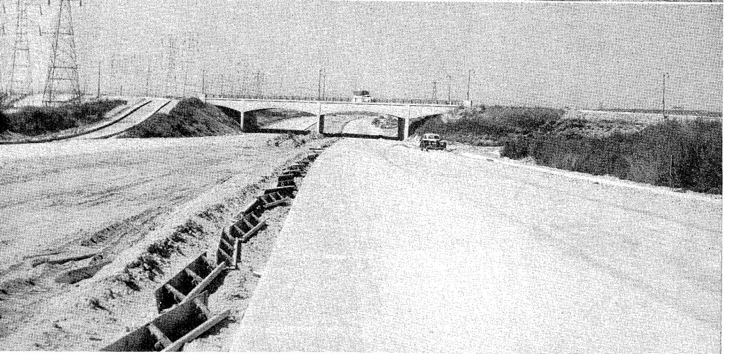
UPPER: Looking northerly toward Atlantic Avenue Undercrossing. The pavement on main traffic lanes of freeway has been completed, and construction operations are in progress on the side collector roads and ramps. CENTER: Looking easterly along Dominguez Street showing, on left, steel girders in place for Pacific Electric grade separation and on right steel girders in place for Union Pacific Railroad grade separation. LOWER: Looking southerly along Long Beach Freeway showing the overpass bridge carrying Long Beach Boulevard over the freeway. Northbound on-ramp from Long Beach Boulevard shown on left.
