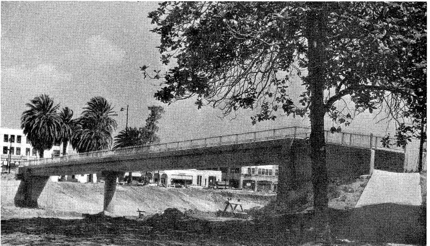
UPPER—Looking easterly along Washington Boulevard showing nearly completed underpass bridge structure carrying the Harbor Freeway. LOWER—Looking southeasterly, showing Harbor Freeway in vicinity of 21st Street, construction details of pedestrian overcrossing.
