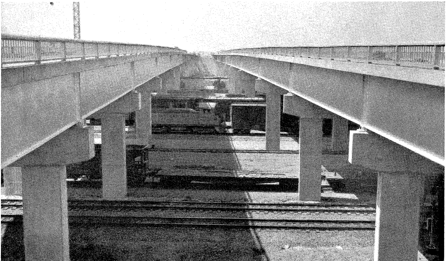
Union Pacific Railroad tracks under East Yard Overhead as viewed from the north abutment of this bridge
