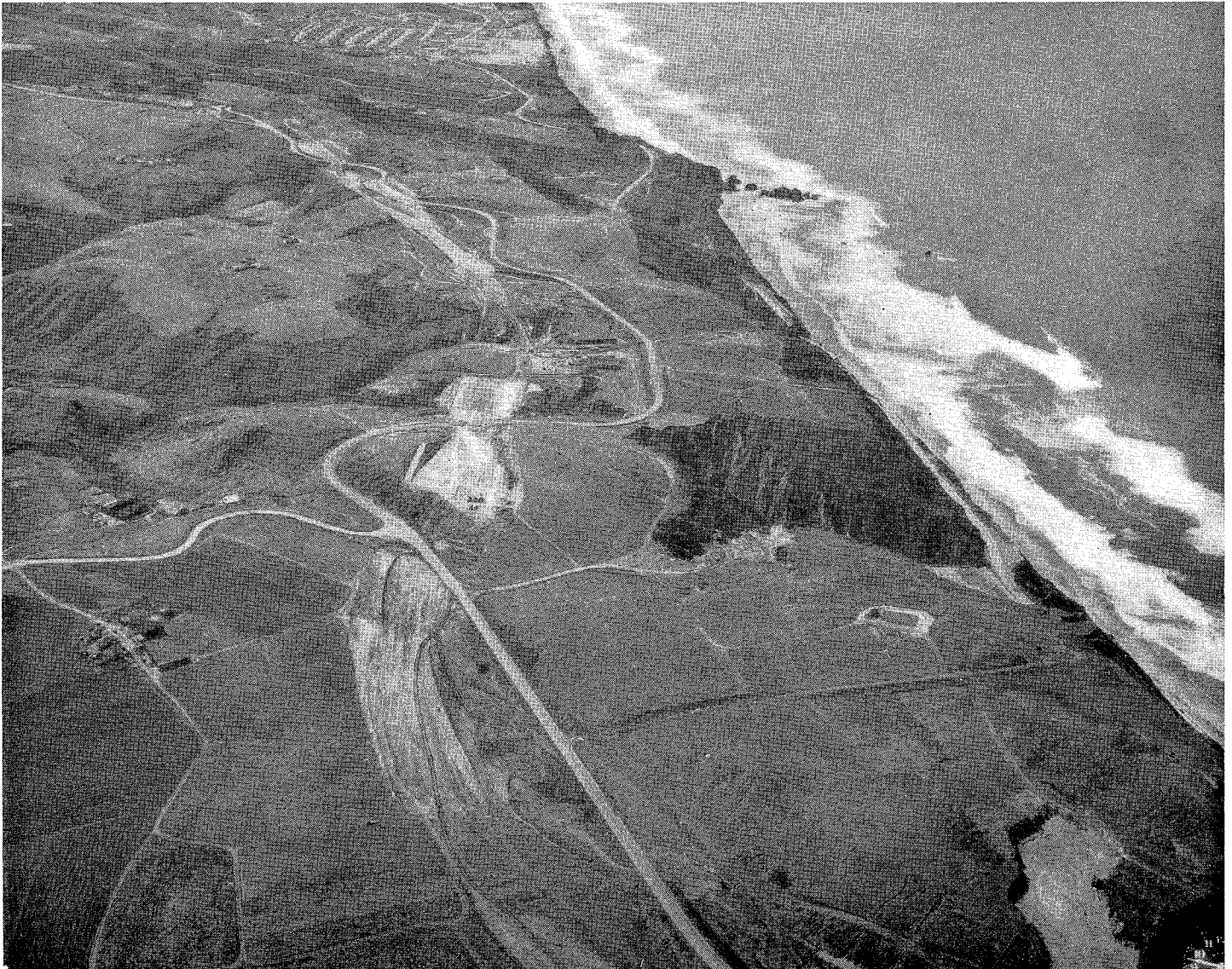
View showing progress of grading operations for Skyline Boulevard from Edgemar Road to junction of Routes 55 and 56 in Daly City
