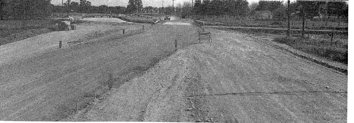
UPPER—View of project south of Gustine, looking north toward Borelli's Corner, showing new bridge with new alignment curving to right. CENTER—Bridge at Gustine Canal. View looking westerly showing bank lining. LOWER—View of project south of Gustine looking south, showing new alignment at south connection.
