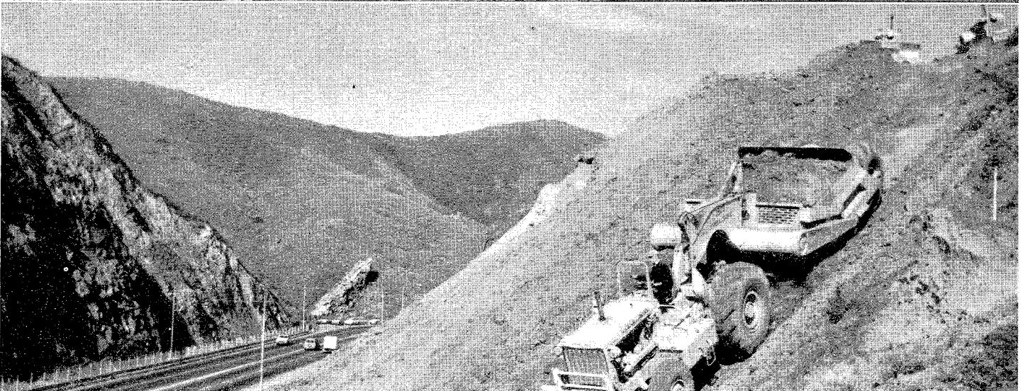
These photos courtesy of Caterpillar Tractor Company show construction on Waldo Grade approach to Golden Gate Bridge. An ingenious and carefully worked out sequence of construction operations is being followed with the result that the work is being accomplished with minimum interference to passing traffic.
