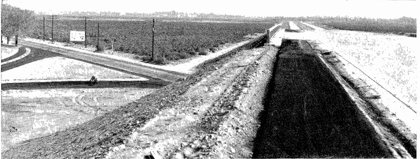
UPPER: Looking easterly at east end of project showing Archibald Avenue in background. CENTER: Looking westerly along completed freeway showing Sixth Street Overcrossing Bridge in City of Ontario and Campus Avenue Bridge in background. LOWER: Looking easterly along freeway at San Bernardino Avenue.
