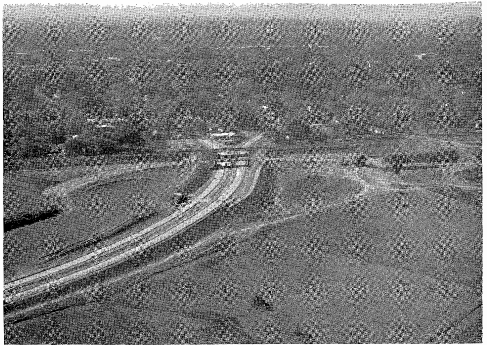
"A" Street Overcrossing and floodgates are shown in center foreground with Southern Pacific Railroad line immediately in back of these structures. View is looking south toward Sacramento.
