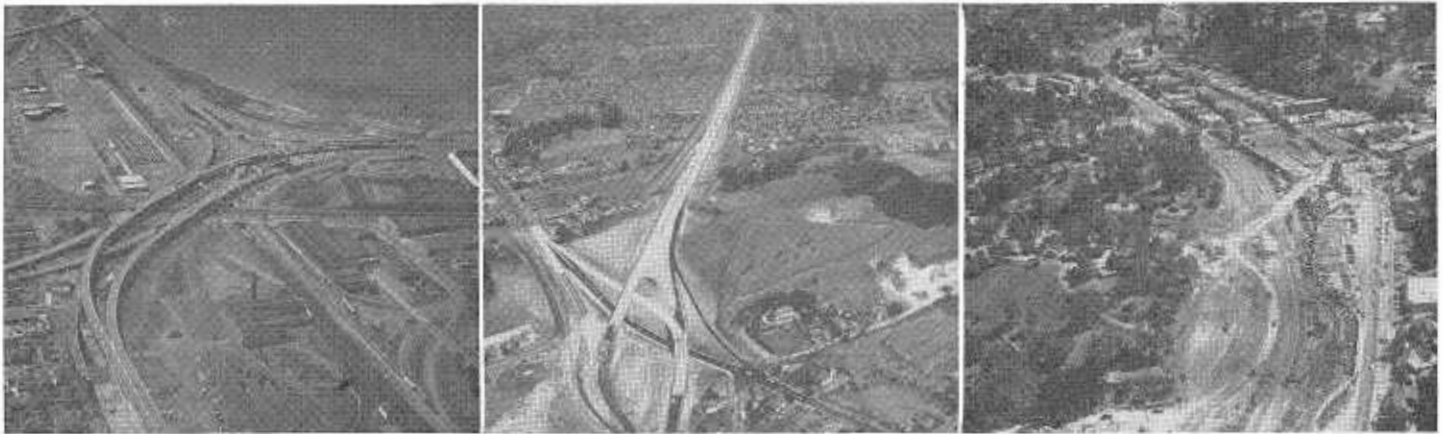
LEFT: East Bay Distribution Structure, showing pier construction for additional ramps under way; Bay Bridge toll plaza in background is also being improved. CENTER: Looking east toward Dublin Canyon on newly opened Castro Valley Freeway former US 50 Route curving toward left. RIGHT: Looking easterly along route of Placerville expressway, showing construction operations.
