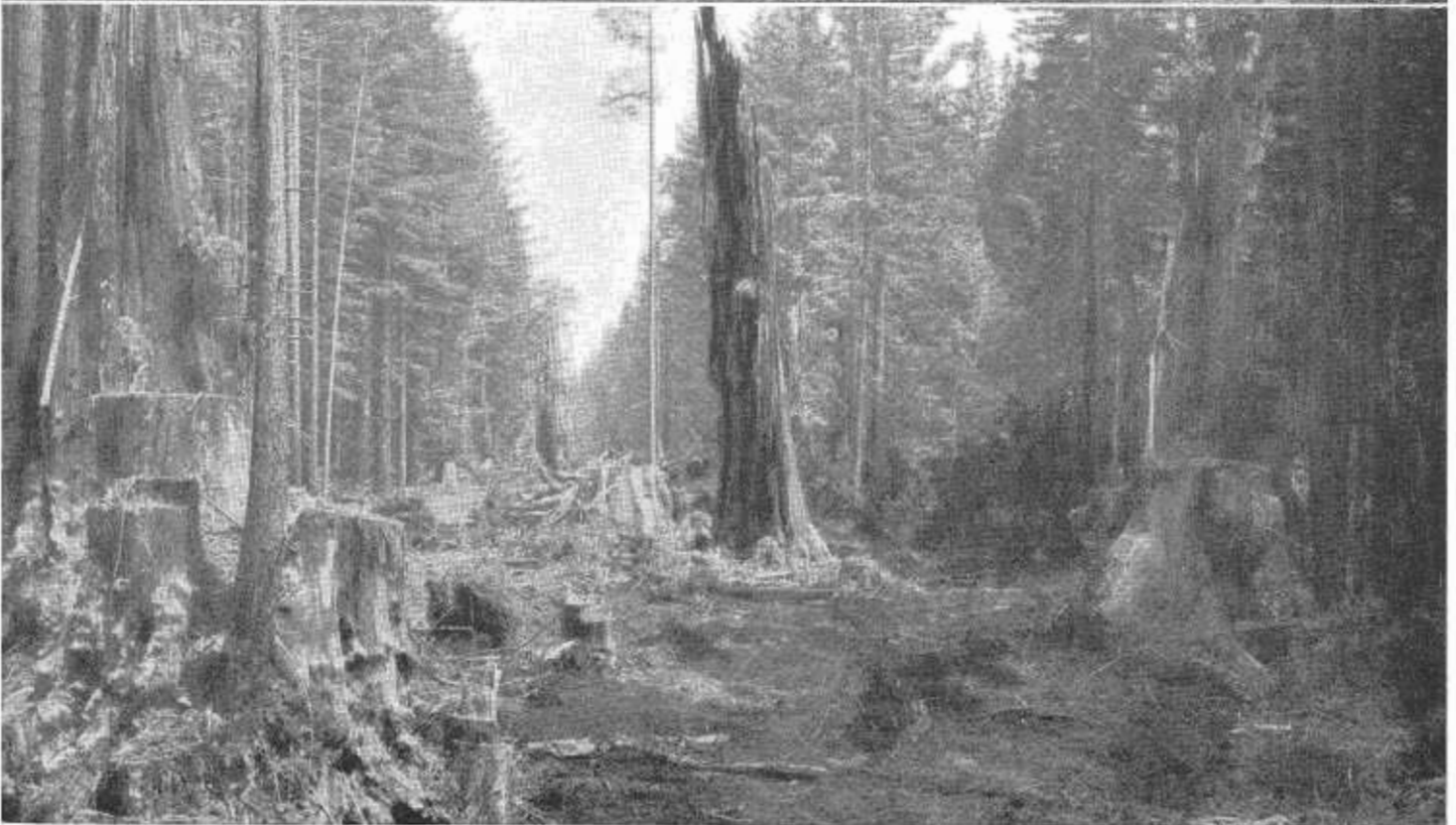
UPPER: This blasting scene has been repeated many times in order to remove the legion of stumps resulting from logging and clearing operations. LOWER: View showing clearing partially completed through an area of dense second-growth redwood forest. The large stumps resulted from logging operations in the 1890's. Approximately one-half of the new alignment passes through this type of forest.
