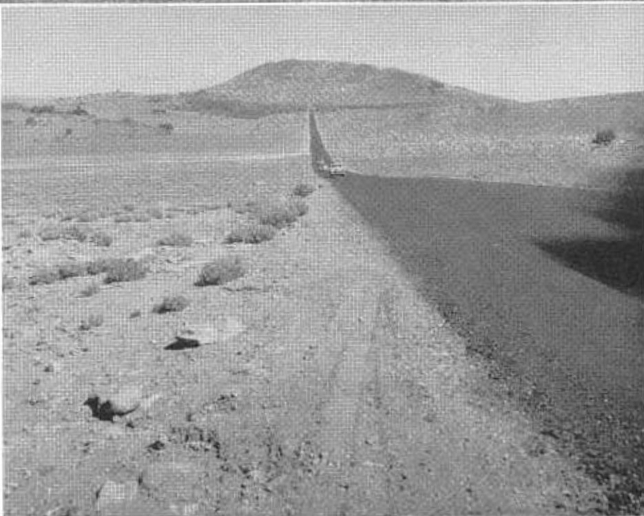
UPPER: New highway looking from just west of Alpine county line. LOWER: Looking east on new road.
