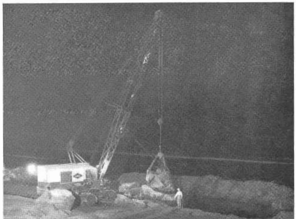
Looking oceanward showing Lima 803 crane placing 11-ton toe rock behind sand dike
