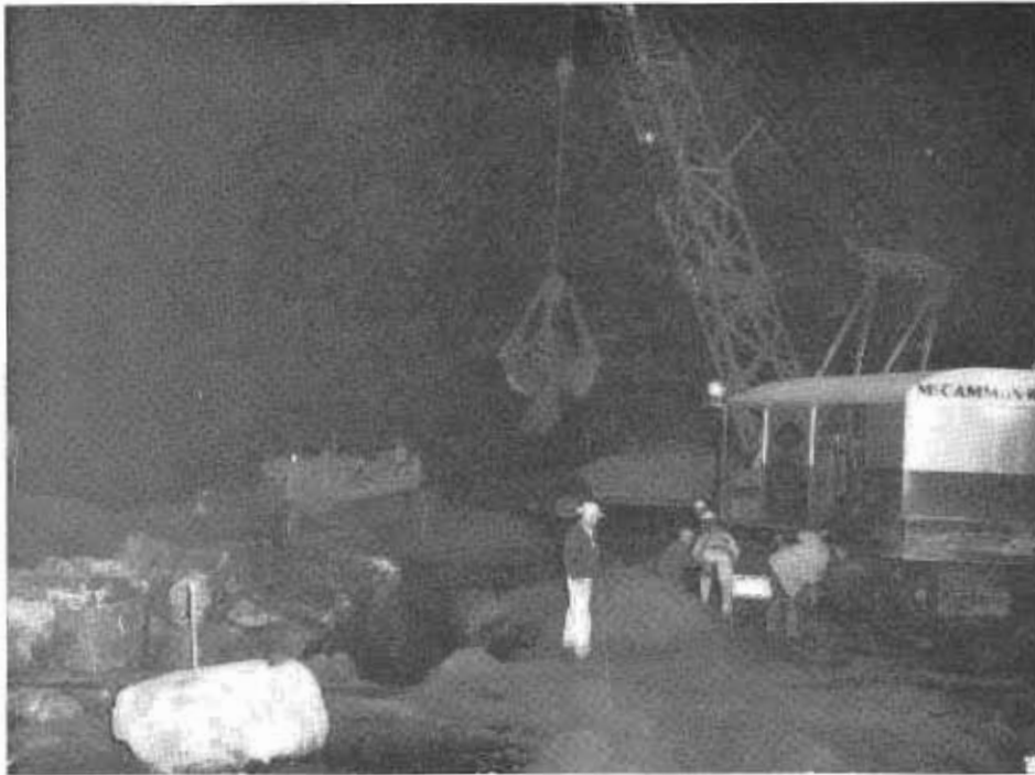
Lima 803 crane with 70-foot and 2-cubic-yard Esco orange-peel bucket with rock hooks placing rock backing in riprap section
