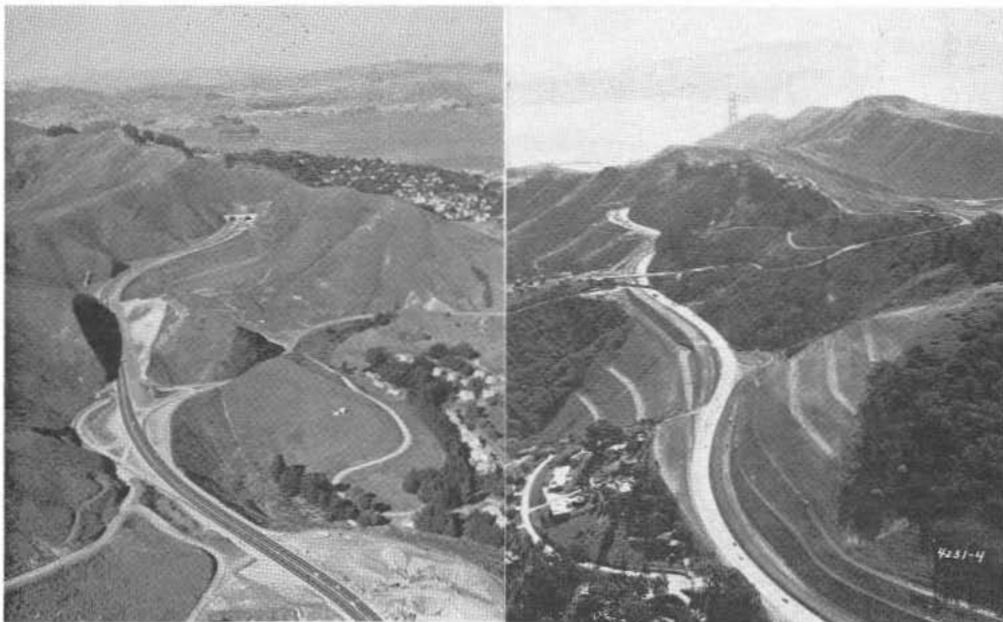
LEFT—Construction operations on Golden Gate Bridge Freeway immediately north of the bridge. New lanes will lead to portal of twin bore of Waldo Tunnel which appears to right of existing tunnel portal, RIGHT—Construction operations for Golden Gate Freeway.
