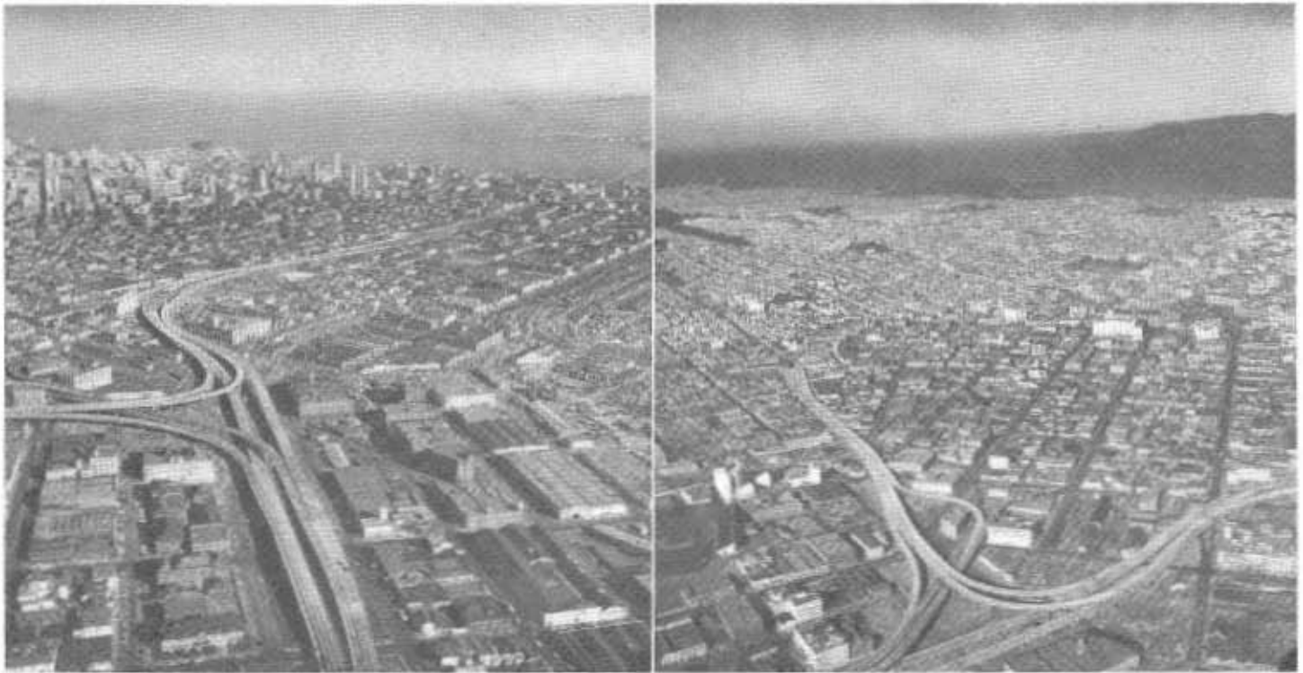
LEFT—Division Street Interchange on Bayshore Freeway in San Francisco showing progress of construction on final units of the freeway which will connect with the Bay Bridge approach in the center right of the picture. RIGHT—Looking westerly along the initial unit of the Central Freeway in San Francisco from its junction with the Bayshore Freeway at the Division Street interchange to its present terminus at 13th and Mission Streets.
