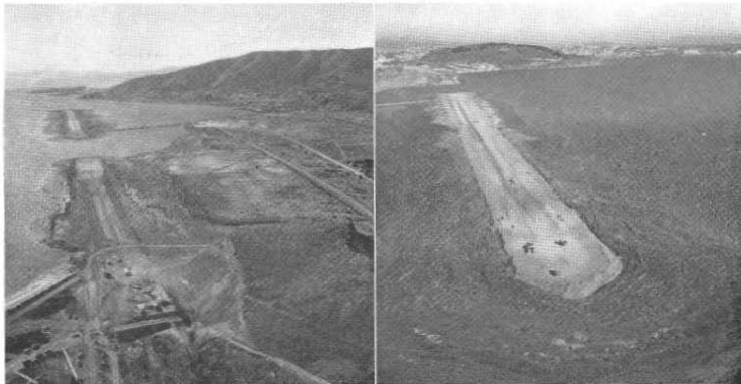
LEFT—View of construction operations for closing of 3.6-mile gap in Bayshore Freeway. Candlestick Point in foreground, looking south across open water toward Sierra Point. RIGHT—Fill operation for Bayshore Freeway midway between Candlestick Point and Sierra Point. Wedge-shaped form is used during end-dumping operation to maintain outward flow of mud. This view, which shows shape of mud wave, was taken during low tide.
