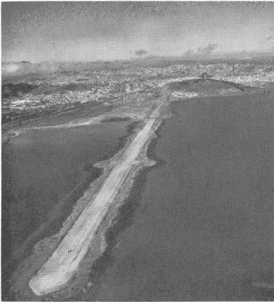
Fill for open water section of Bayshore Freeway across Candlestick Cove. Widening at center of picture is location where reinforced concrete box culverts will be constructed to equalize water level.
