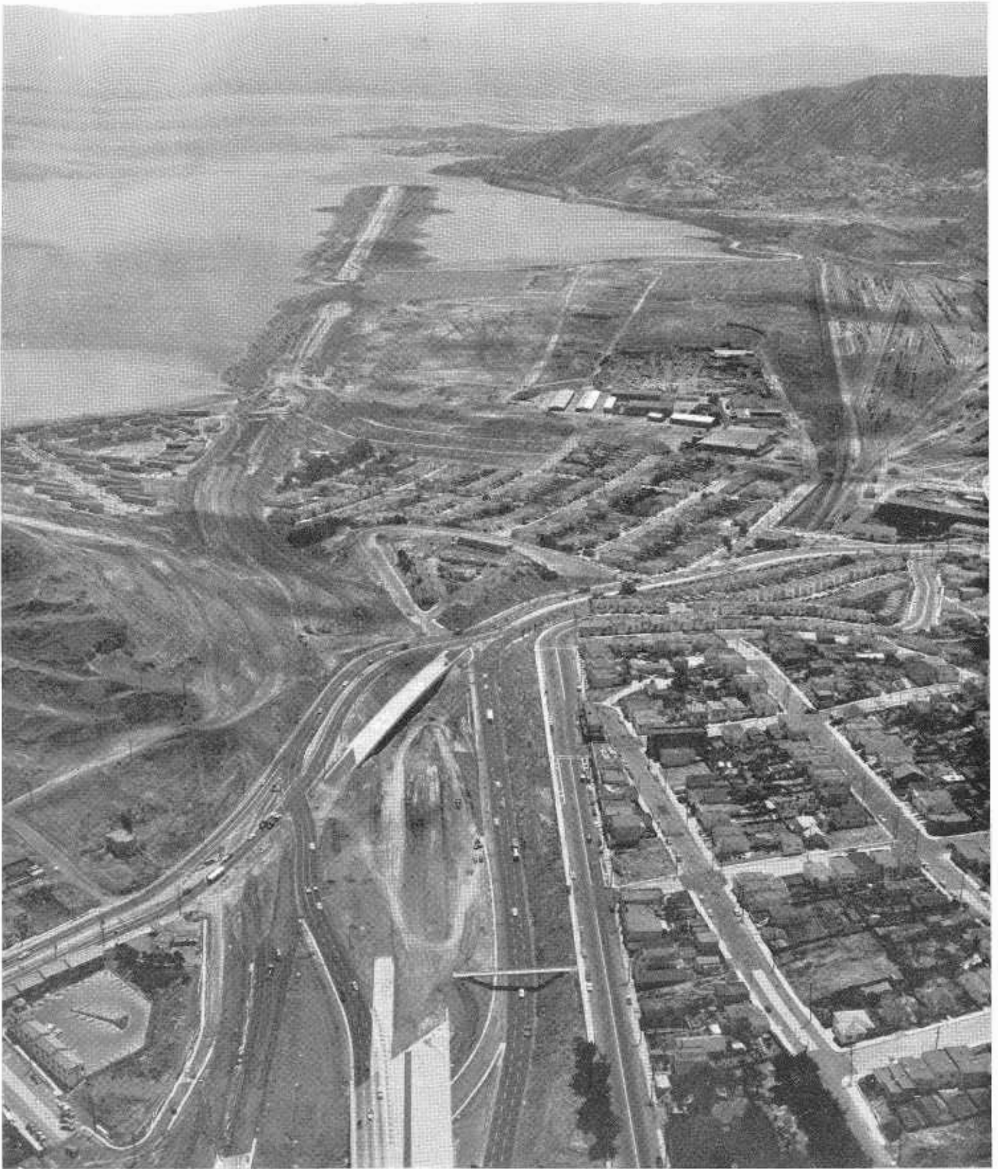
Construction operations on Bayshore Freeway from Third Street Interchange in foreground. Looking southerly along open water fill toward Sierra Point. The Division of Highways is advertising for bids on a project which will complete all rough grading and structures required to close the overwater gap on the freeway.
