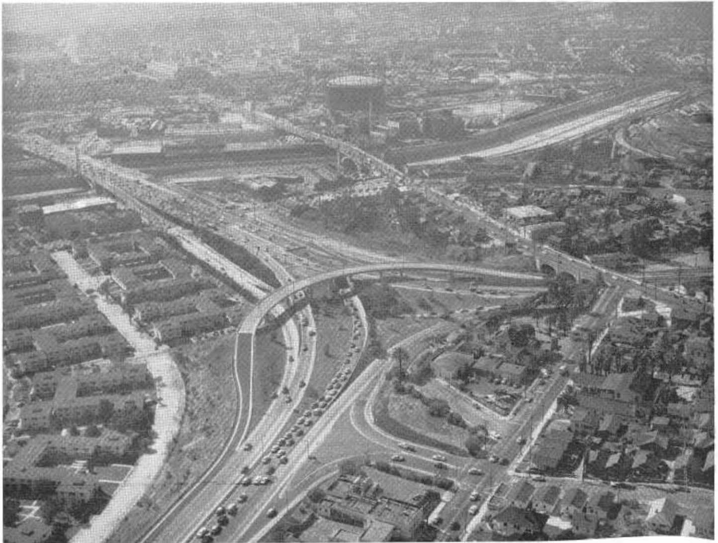
Looking northwesterly toward Santa Ana-San Bernardino interchange with widening construction in progress on Los Angeles River bridge shown center left
