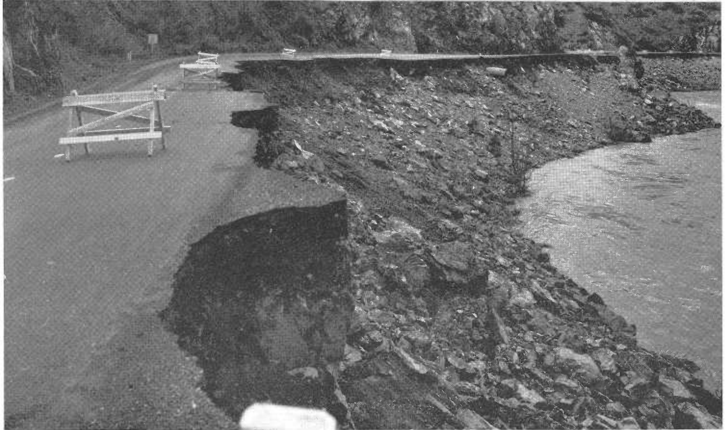
UPPER—Temporary detour under construction on Trinity River two miles from Douglas City. LOWER—Typical damage along Trinity River.
