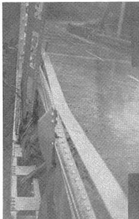
Large logs battered vital truss members of Trinity River structure at Cedar Flat, US 299. Bridge saved by diverting flow through gap bulldozed in road fill.
