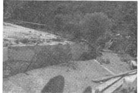
Flood damage vicinity El Portal—Looking westerly from box culvert, showing pathway to temporary pedestrian bridge. Express parked on detour approach to Pigeon Creek temporary bridge.
