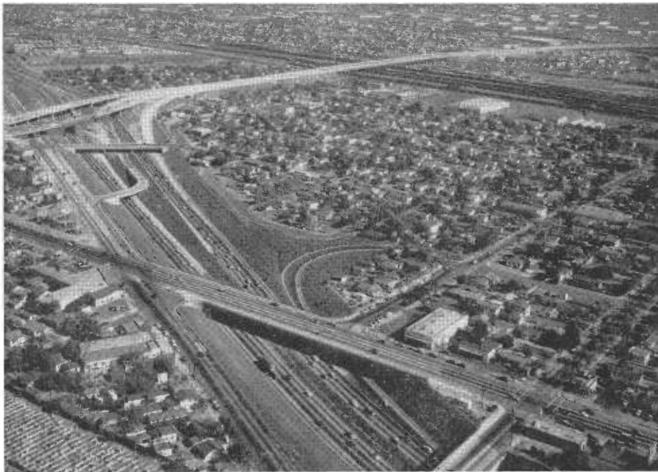
Looking southeast along Santa Ana Freeway showing construction in progress now nearing completion on Long Beach Freeway. New construction provides traffic interchange between the two freeways.
