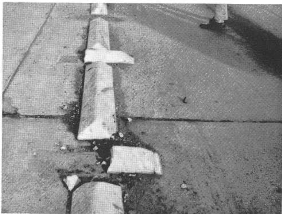
UPPER—Experimental traffic bars immediately after installation. LOWER—Traffic bars cemented with asphalt emulsion after two to three months.
