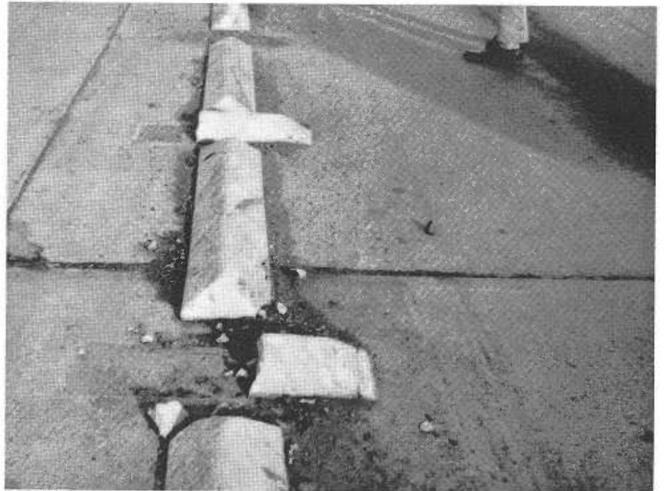
UPPER—Experimental traffic bars immediately after installation. LOWER—Traffic bars cemented with asphalt emulsion after two to three months.
