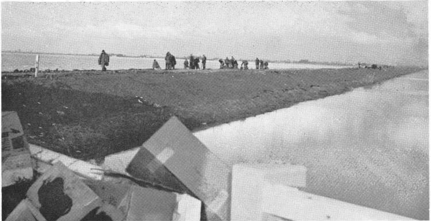
Crews work to save north levee of Natomas Cross Canal. (US Air Force photo)
