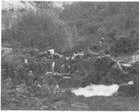
Flood damage vicinity El Portal—Excavating for footings for detour bridge to be constructed right of Station 198. Note rock foundation.
