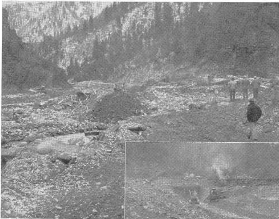
Chippis Creek Bridge on US 40 Alternate near Belden buried in silt and rock carried by rampant stream. Insert shows digging out operation.
