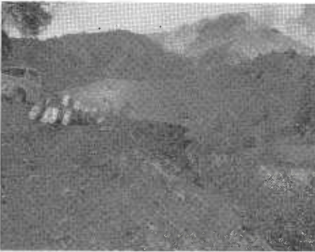
Flood damage vicinity El Portal—Inlet end of culvert plugged by tree Station 198.
