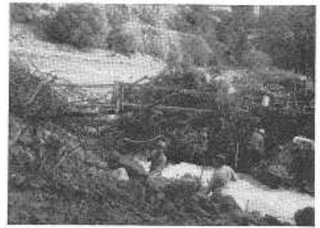
Flood damage vicinity El Portal—Excavating for footings for detour bridge upstream on Pigeon Creek.
