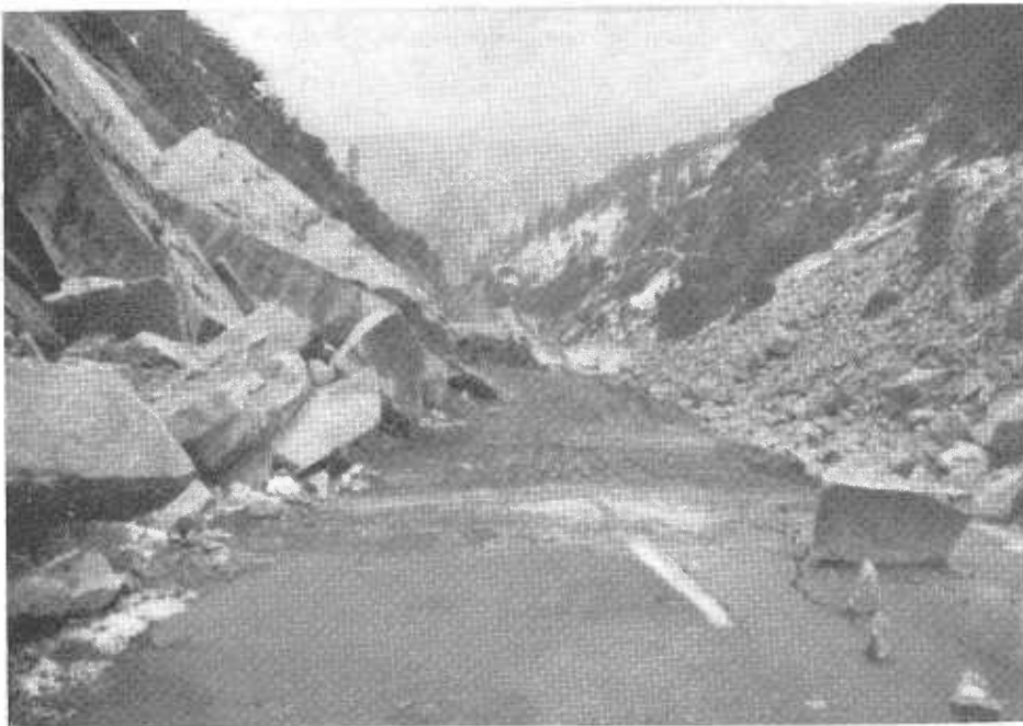
Slides and erosion east of Arch Rock Tunnel on US 40 Alternate, Butte County
