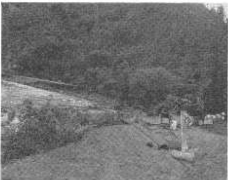
Flood damage vicinity El Portal. Looking easterly over damaged 8' x 8' concrete box Station 198. Also shows temporary walkway constructed over tree blocking culvert.
