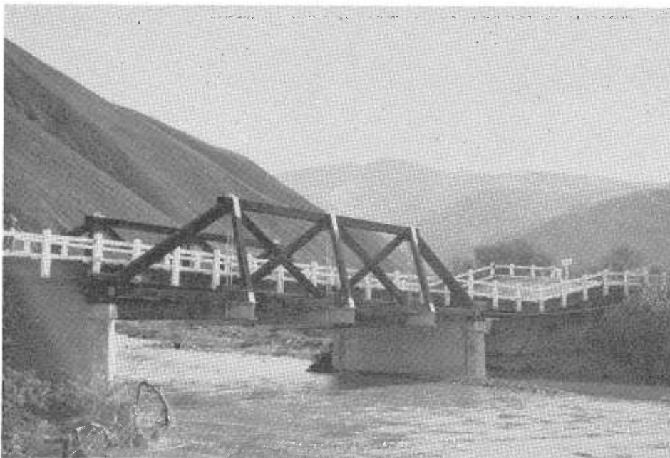
View of downstream side of San Carpojo Creek Bridge 22 miles north of Cambria on Sign Route 1, San Luis Obispo County
