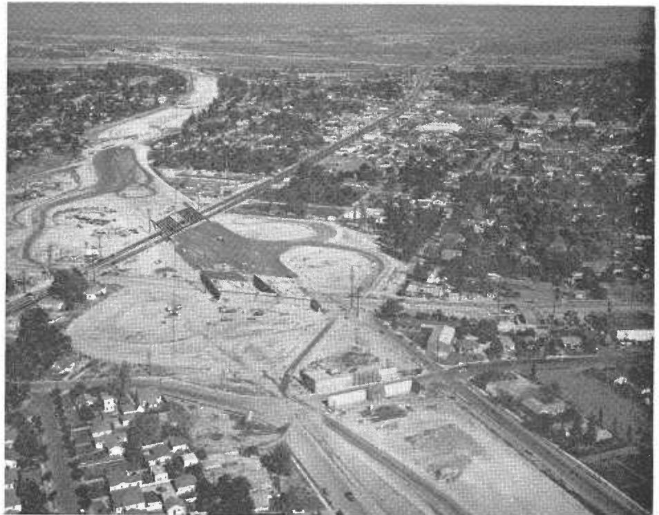
Looking east along San Bernardino Freeway, showing construction progress through City of El Monte
