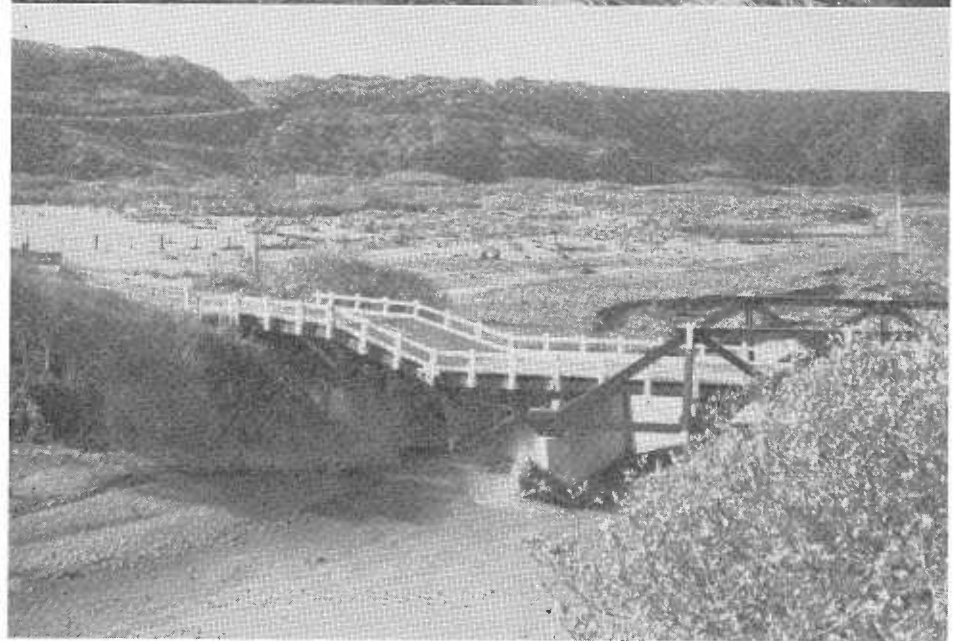
UPPER—View of upstream side of El Capitan Creek showing debris at inlet end of structure. El Capitan Creek is located 16.5 miles north of Santa Barbara on US 101. LOWER—View of upstream side of San Carpojo Creek Bridge 22 miles north of Cambria on Sign Route 1, San Luis Obispo County.
