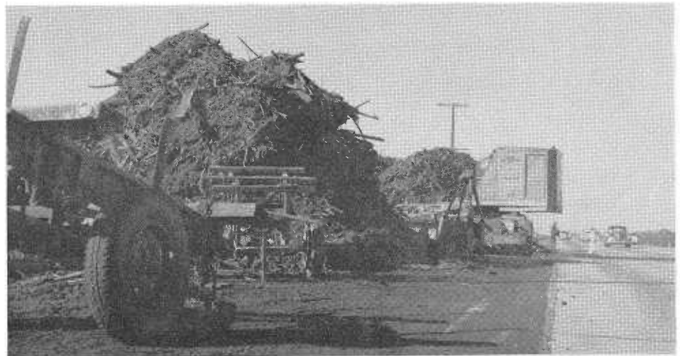
Debris removed from entrance of single span Saratoga Creek Bridge north of Santa Clara. Clogging flooded Bayshore Highway, US 101 Bypass.
