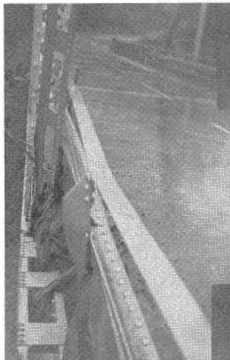
Large logs battered vital truss members of Trinity River structure at Cedar Flat, US 299. Bridge saved by diverting flow through gap bulldozed in road fill.
