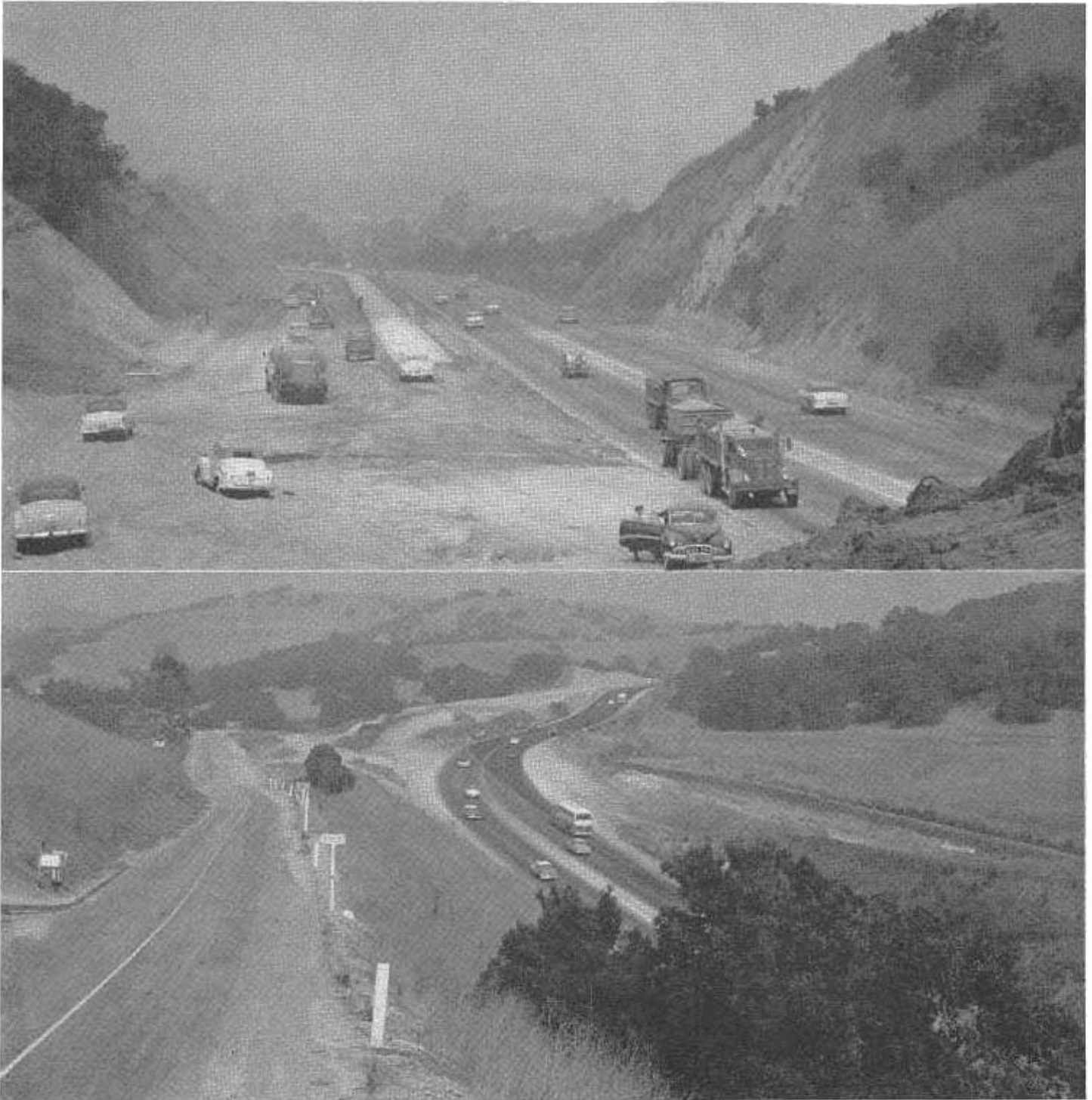
UPPER—Looking westerly from eastern end of paving construction. LOWER—Looking westerly showing grading between Pomona and West Covina.
