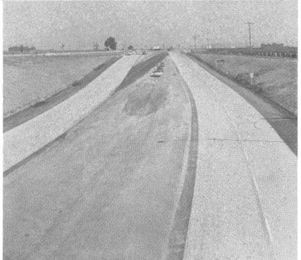
UPPER—North Delano Overhead Crossing. In right background Southern Pacific Railroad and old US 99, looking northerly. LOWER—South end of project. Temporary crossing in foreground. View is looking southerly. Old south entrance to Delano in left center.
