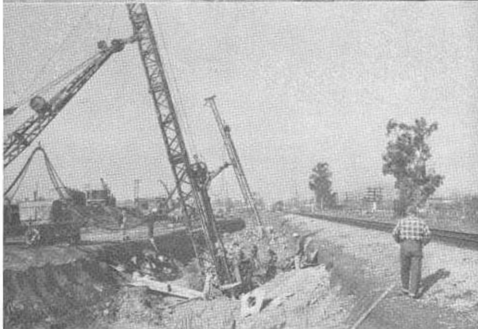
UPPER—Erecting steel at East El Monte structure. LOWER—Drilling pile holes at El Monte structure.
