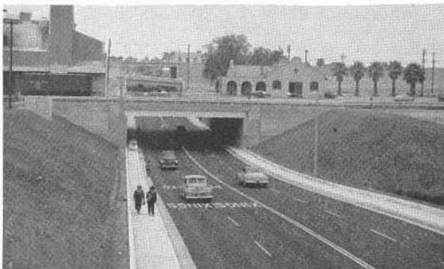
Looking northerly along Eighth Street, showing in turn the Eighth Street Underpass, the J Street Off-ramp undercrossing, and the Eighth Street Undercrossing. Note completed embankment for the San Bernardino Freeway shown in right background.
