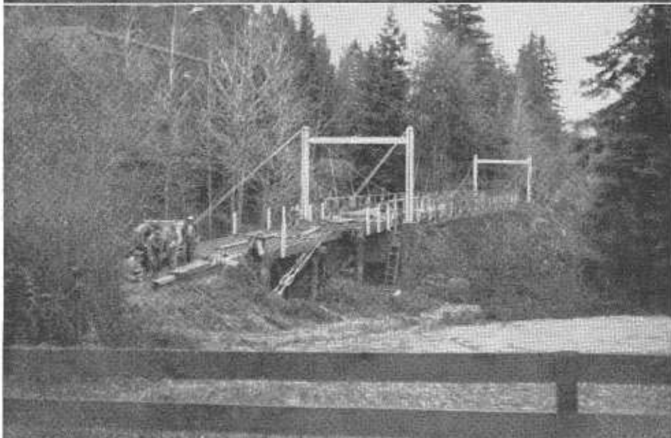
UPPER—Showing flood-damaged Larrabee Creek Bridge. LOWER—Repair work on bridge under way.
