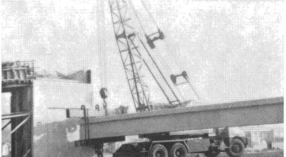
UPPER—Typical undercrossing, Sunset-Irwindale Undercrossing. CENTER—Prestressing operation at Big Dalton Wash. LOWER—Erecting precast superstructure at Bess Avenue.
