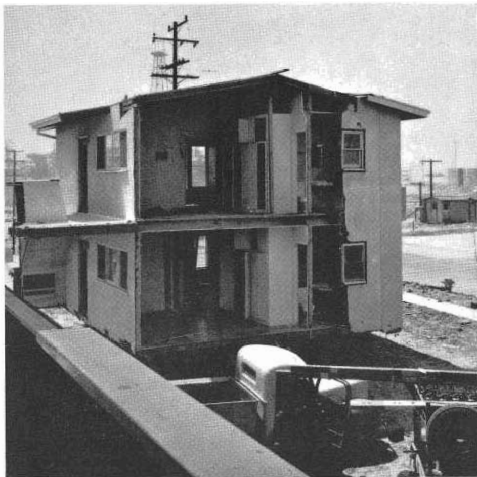
A 16-unit apartment house was cut into five units to facilitate moving. This is a view of one of such units.
