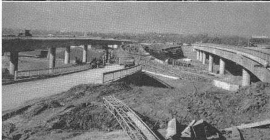
UPPER—Looking westerly at Long Beach-Santa Ana Interchange. LOWER—Looking northerly showing in center interchange structures that will provide for traffic movement between the Santa Ana Freeway and the Long Beach Freeway. Completed structure to left will carry southbound Long Beach Freeway traffic and one to right will carry northbound.
