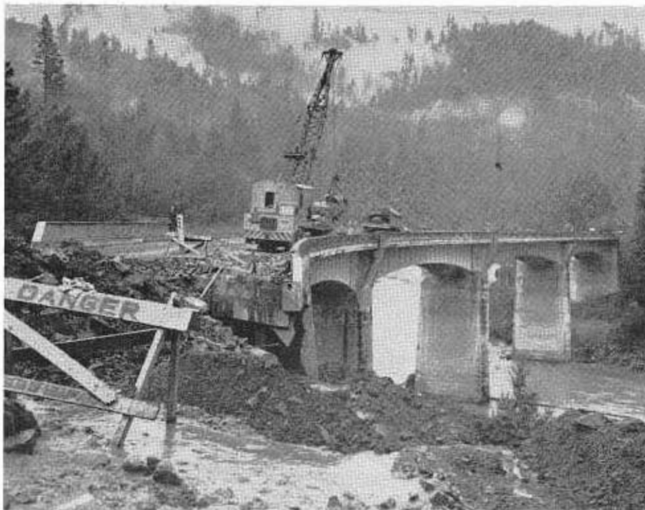
Flood damage repair work to the Smith Point Bridge across South Fork Eel River on US 101, six miles south of Garberville. Note damaged north approach span.
