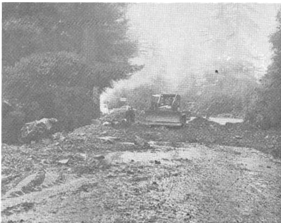
US 101 near Piercy, Mendocino County; removing slide after Christmas week storm and floods
