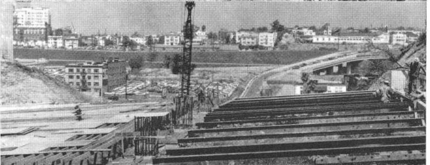
UPPER—Grading operations in progress. Timber bridge shown was erected as traffic detour for Hope Street. CENTER—Grading operation under way across Grand Avenue. Traffic was detoured to east on timber bridge not shown in photograph. LOWER—Shown in foreground are details of falsework for Hope Street Bridge on Fourth Street. Harbor Freeway in background.
