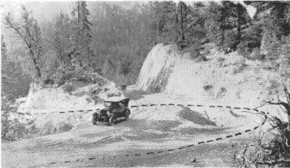
Typical highway construction in Sacramento Canyon about 1928. Dotted line shows road before relocation.
