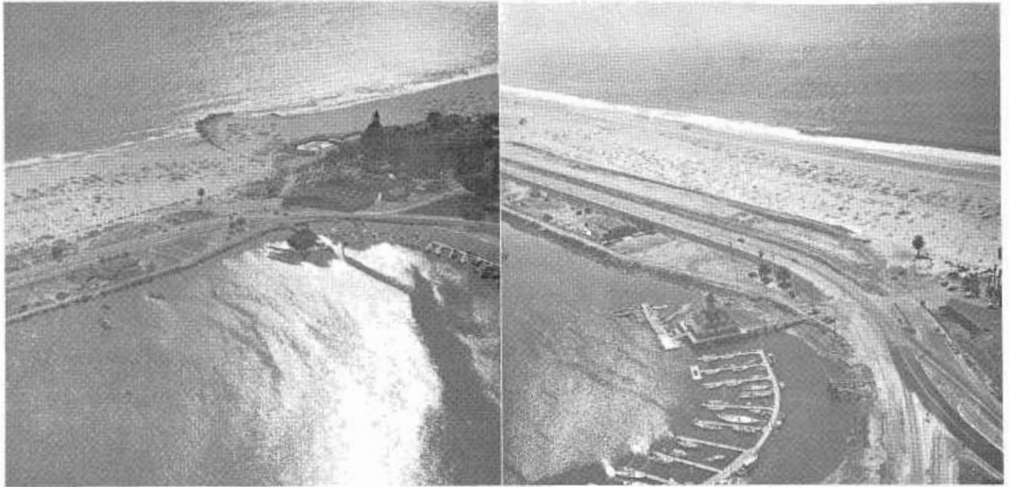
LEFT—View northerly toward Coronado. New lanes for southbound traffic under construction on left. Existing concrete pavement on right provides two lanes of travel for northbound traffic. Note new frontage road on right serving bay development area. RIGHT—Northerly end of Strand before construction.
