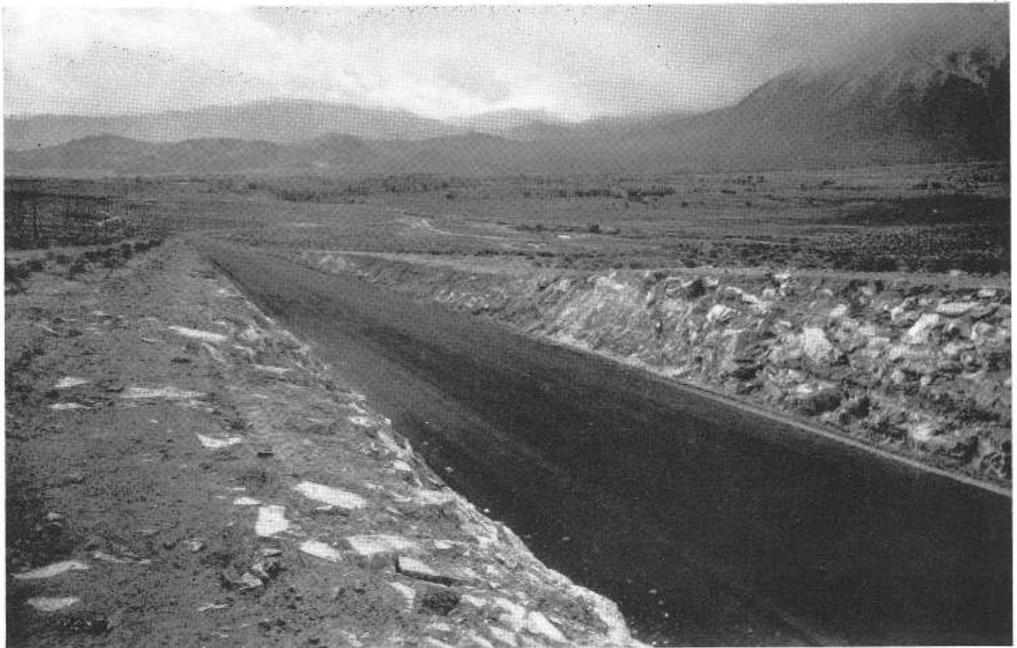
Showing typical lava rock cut and junction with old highway at foot of grade
