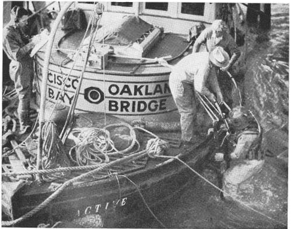
Expert divers were used extensively in laying the foundations for the bridge caissons
