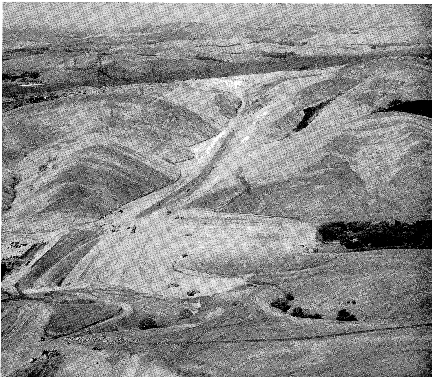
Excavation material from the "big cut" is being placed in a fill which will be 140 feet high when completed. To date approximately 5,000,000 cubic yards of earth have been excavated from the "big cut" and rolled and compacted in the fill which should be to grade in February, 1957.
