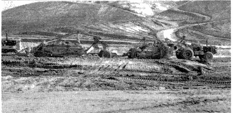
UPPER—Picture showing "tandem" hookup consisting of one tractor and one operator hauling two scrapers. This picture shows equipment ascending top of "big cut" preparing to be loaded. LOWER—Picture shows "tandem" scrapers being loaded. Rear scraper is loaded first with the assistance of a powerful pusher in the rear. After rear scraper is completely loaded, the front scraper is loaded. After both are loaded, the single operator and tractor take off down the hill to dispose of the material on the fill. East slope of the "big cut" can be seen in the background.
