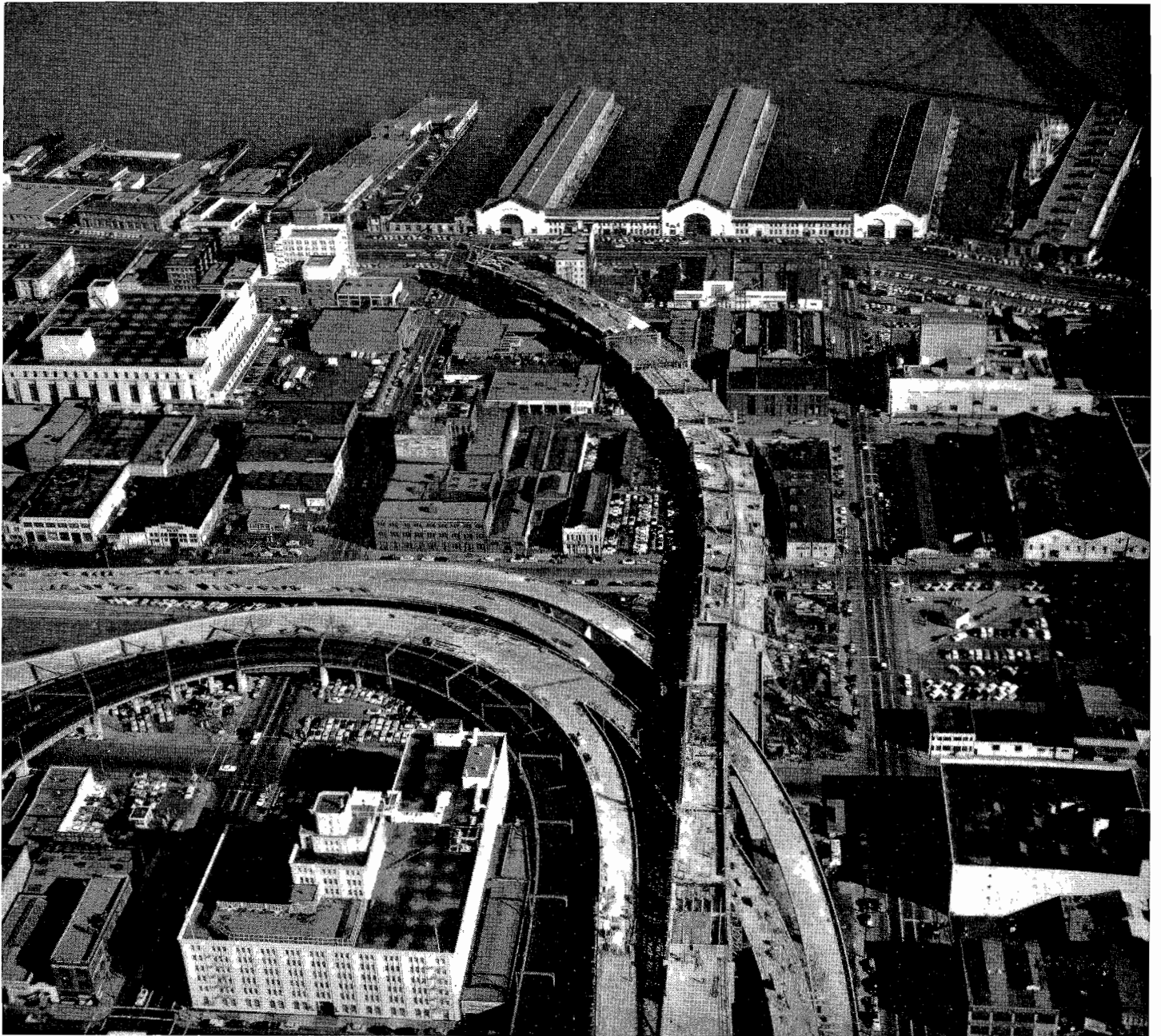
Looking west at Embarcadero Freeway construction. Foreground shows progress toward Embarcadero with Main and Beale ramps in center.
