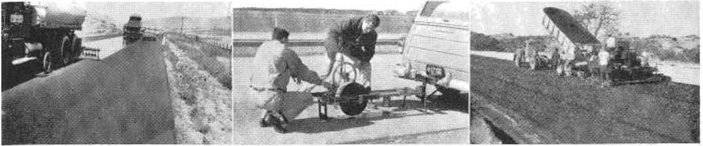
LEFT—Experimenting with bituminous binder containing rubber latex for seal coat work. CENTER—Measuring skid resistance of pavement surface. RIGHT—Placing of Zaca to Wigmore experimental asphalt test sections to determine quality of asphalt necessary for durability.
