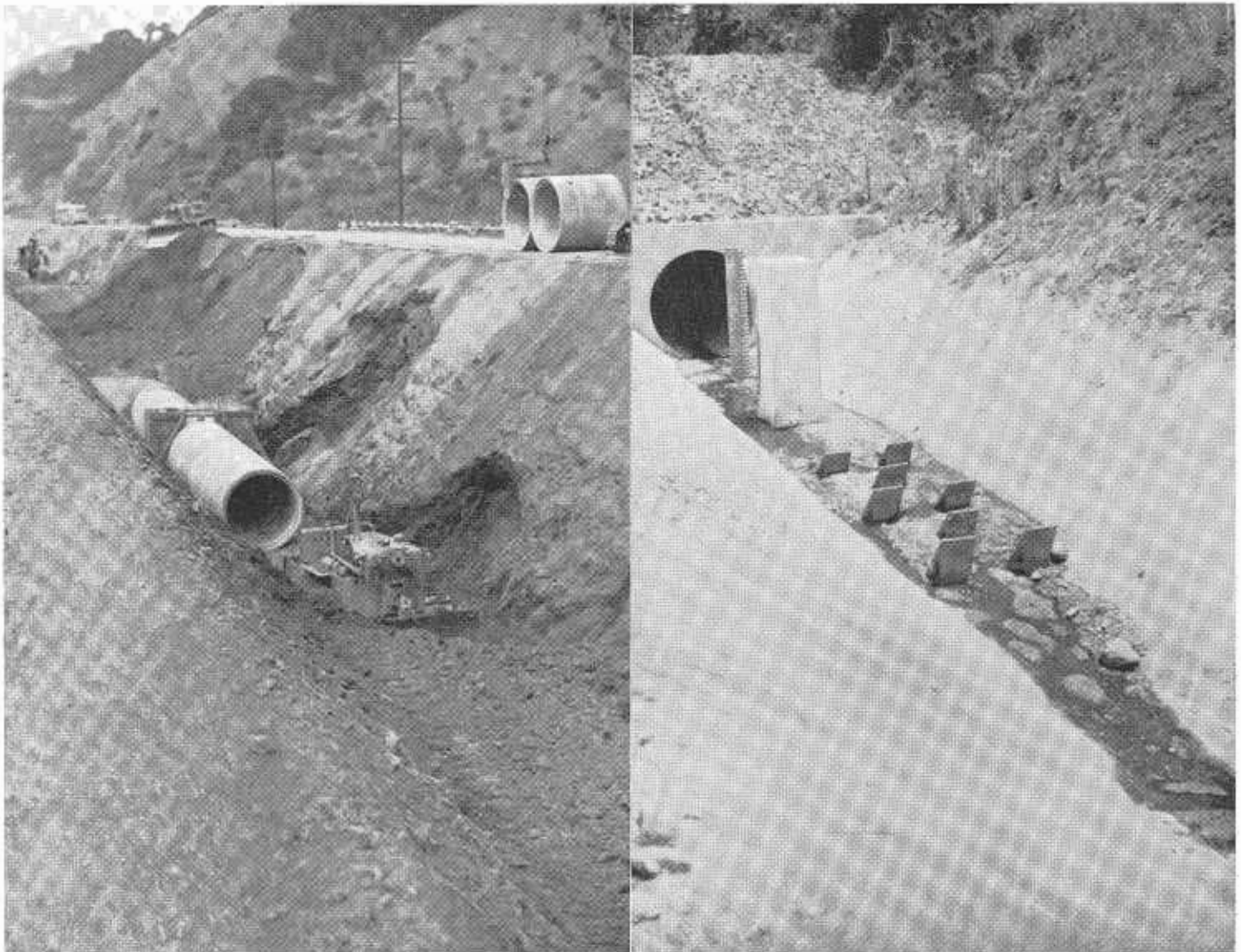
LEFT—Looking westerly toward 84-inch reinforced concrete pipe installation, showing depth of cut from existing traveled way. RIGHT—View of completed aero energy dissipators.
