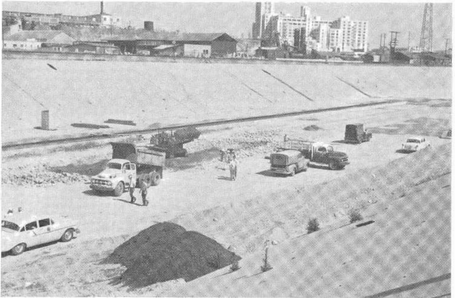
Looking southeasterly showing start of construction work excavating for center pier in the Los Angeles River channel for Santa Monica Freeway bridge. In background is Sears, Roebuck building.
