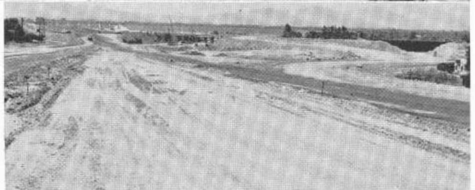
UPPER—Closeup of belt loader. Note dozers feeding belt. LOWER—On San Diego Freeway looking north- erly across interchange roadways. Picture taken from Camarillo Avenue.
