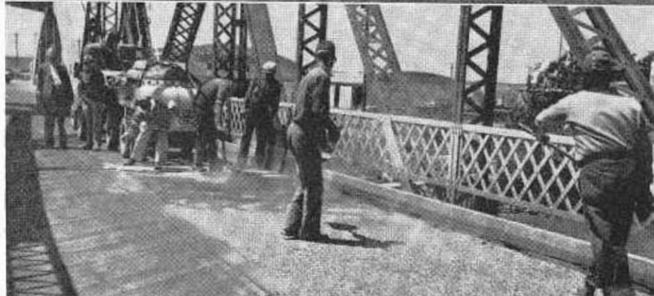
UPPER—Test specimens cut from pavements by coring or sawing. CENTER—Experimental installation of wire mesh to determine whether it will be effective in preventing cracks in asphaltic resurfacing. BOTTOM—Experimental installation of asphalt-latex seal coat to protect wooden bridge deck.
