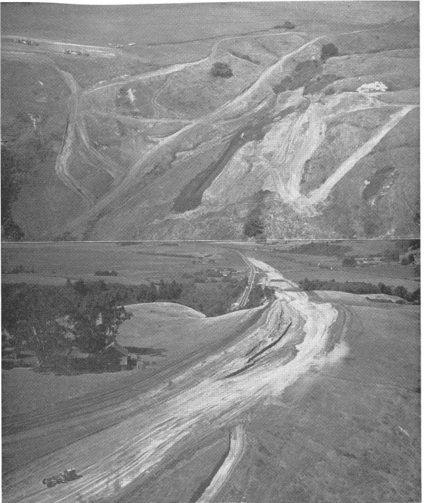
UPPER—Stripping wet material and constructing stabilization trench. Highway centerline is diagonally across picture between lower left-hand corner and upper right-hand corner. This is the site of the heaviest stabilization work on the project. LOWER—General view of new construction at north end of project looking northerly. Junction with present highway in top center.
