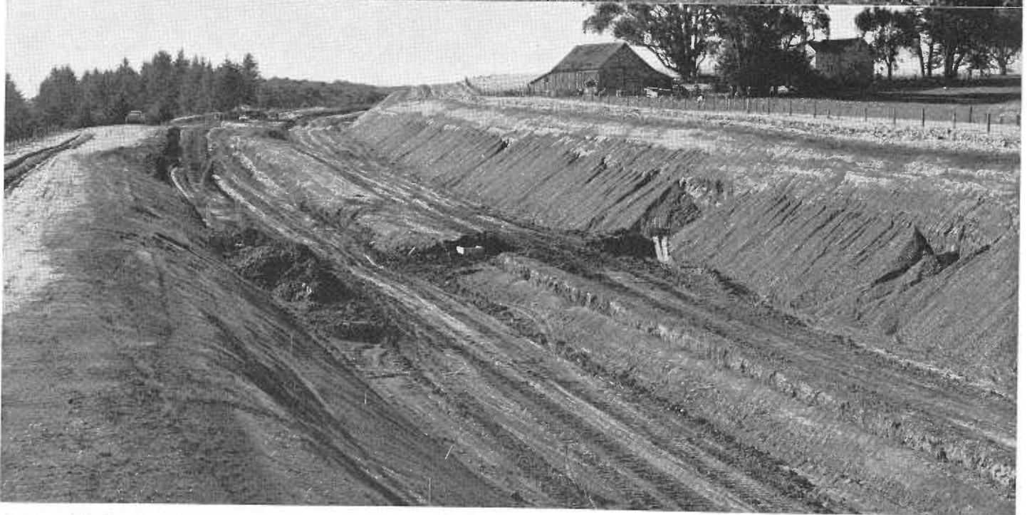
UPPER—Stabilization trench right angles to centerline. Note filter material on slope to allow for percolation of underground water. LOWER—On top of Table Bluff Hill in thorough cut. Note filter material on cut slopes on right replacing material that sloughed away by concentration of underground water.
