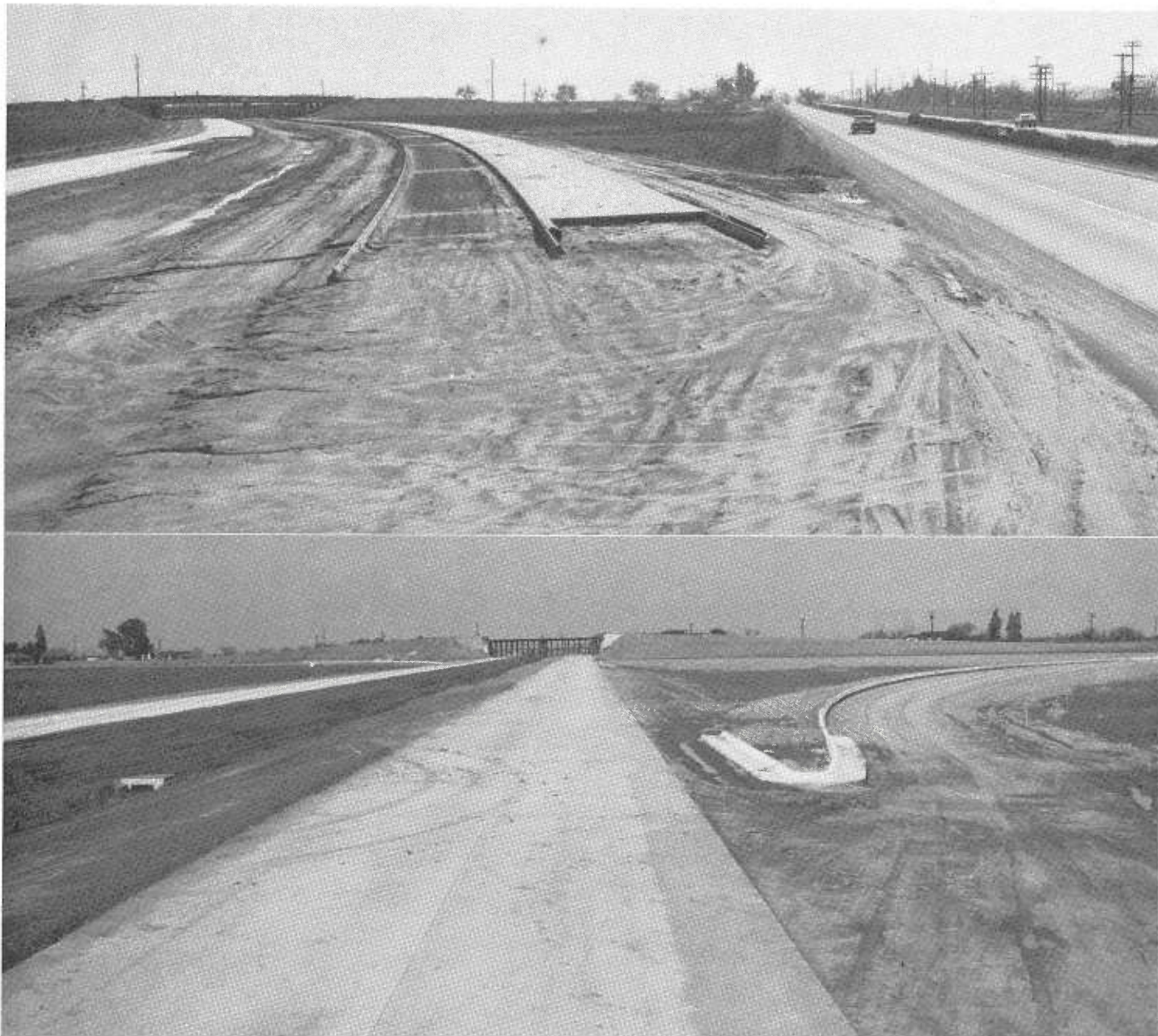
UPPER—Looking southerly at north end connection. LOWER—Looking northerly showing road 26E overcrossing and ramps, which will connect US 99 to the City of Chowchilla.
