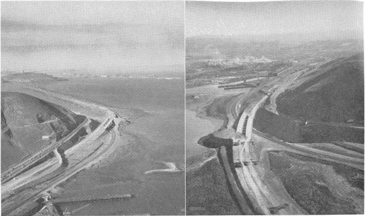
LEFT—Looking northerly at Open Water Fill on Bayshore Freeway. Sierra Point in foreground and Candlestick Point ahead. Note north-bound off-ramp to existing highway in foreground. RIGHT—Bayshore Freeway construction at Sierra Point looking southerly. Note S. P. R. R. relocation. Tunnel right center eliminated.
