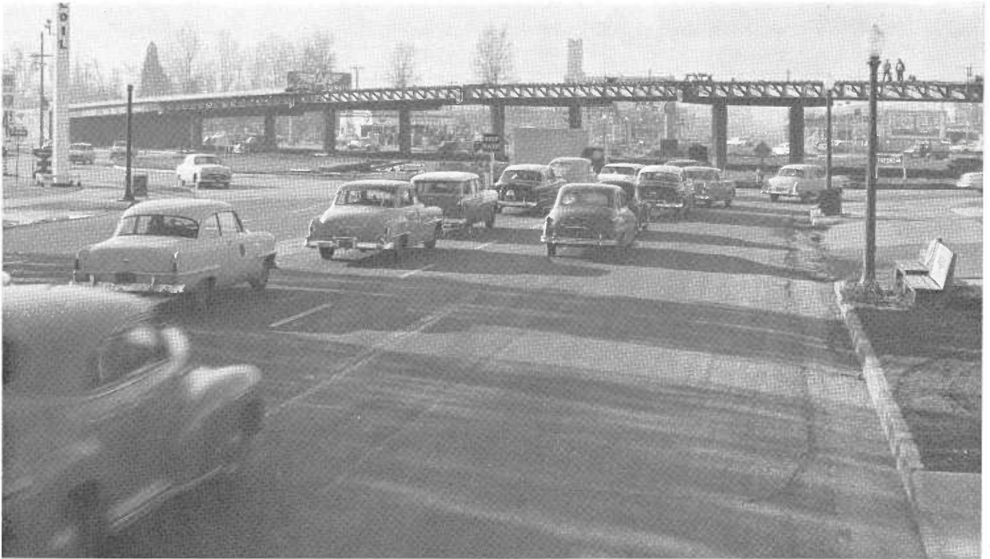
This photo looking north shows steel all in place at Garces Circle Bridge
