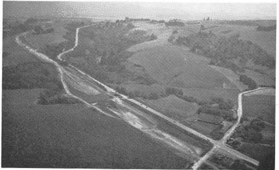
Looking southerly from Hookton Road near north end of project with new highway under construction on left, and existing Table Bluff Grade on right
