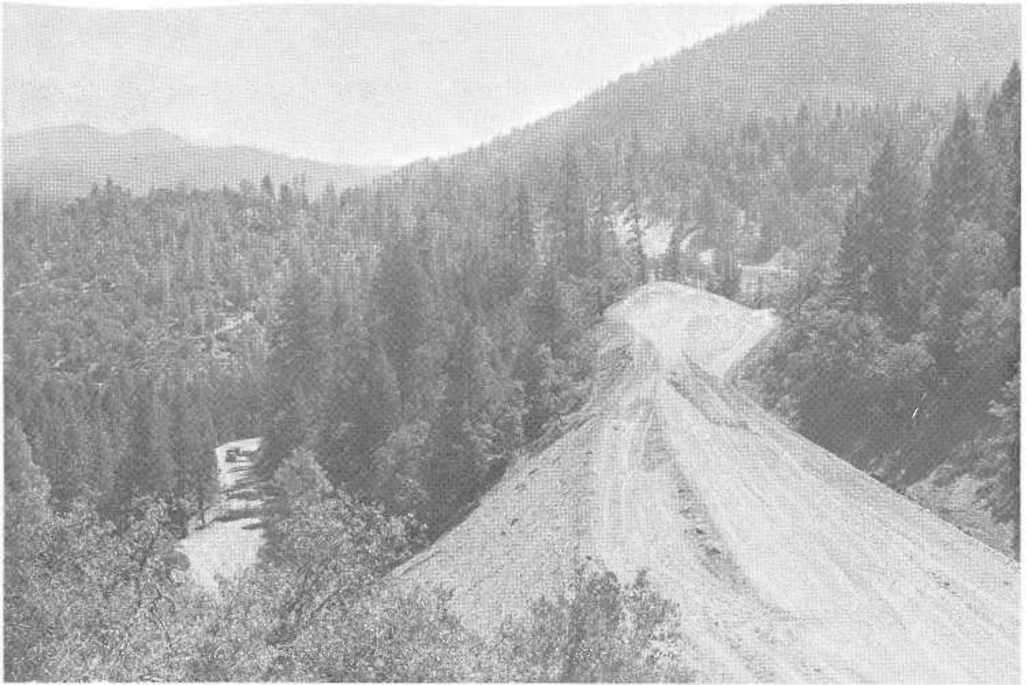
Relocation on the McNutt job meant heavy grading. Old road on the left.
