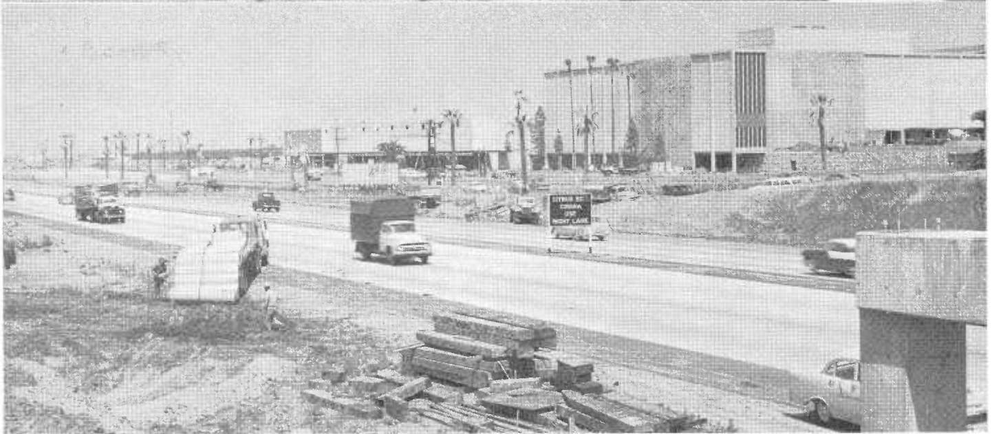
UPPER—Looking westerly along completed San Bernardino Freeway in City of Baldwin Park, showing the Bess Avenue-Frazier Street overcrossing bridge under construction. LOWER—Looking westerly along completed San Bernardino Freeway, showing in foreground construction in progress on Barranca Street overhead bridge in West Covina. In background is shown May Company shopping center now under construction and nearing completion.
