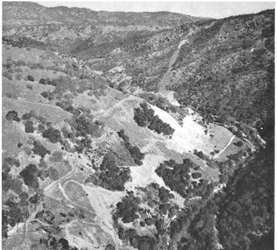
Rugged sidehills are being traversed by relocation of State Highway 20 in canyon of East Branch of Russian River. Existing highway and river will be noted in lower right-hand corner.
