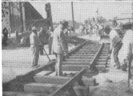
Setting up track section across US 99W at south city limits of Woodland
